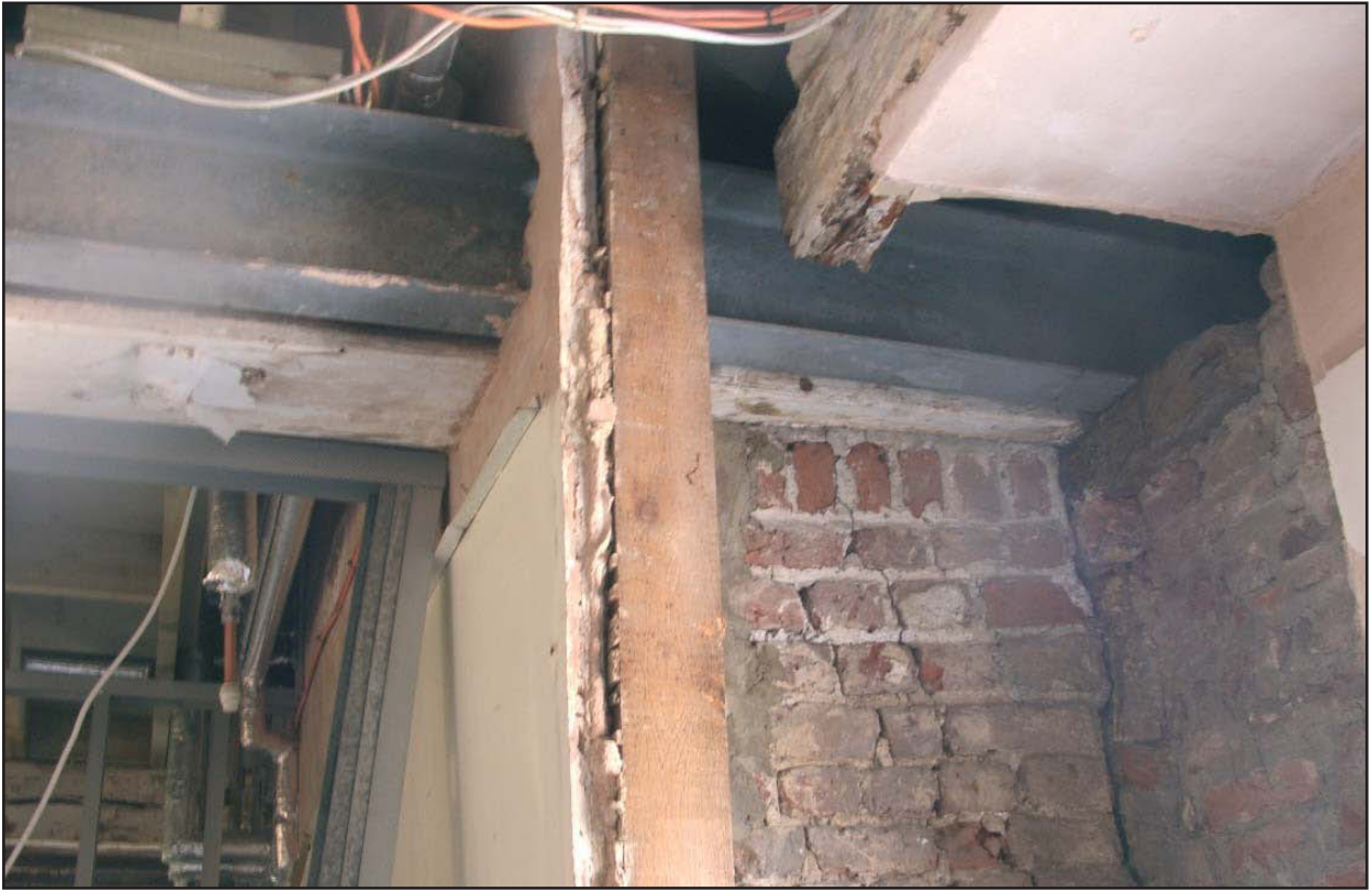
Plate 11: Exposed brickwork of chimney breast (centre right) and inner face of exterior north wall (extreme right)
