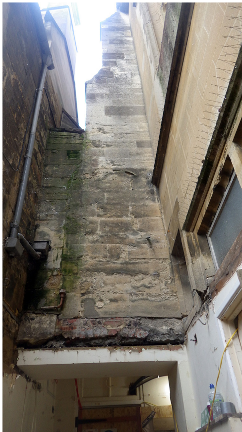
Plate 8: Butters 407 surviving from 1st floor level
