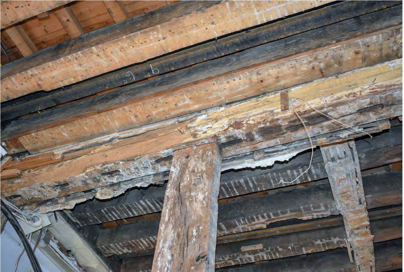
Plate 15: Underside of head rail showing empty mortices
