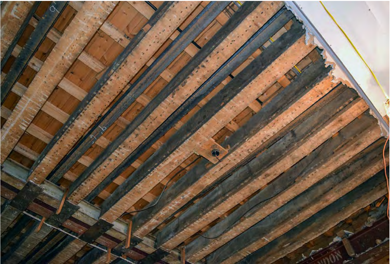
Plate 28: Exposed floor in Old Bursary
