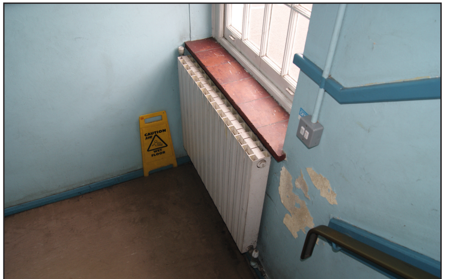
Plate 24: Radiator in stair well
