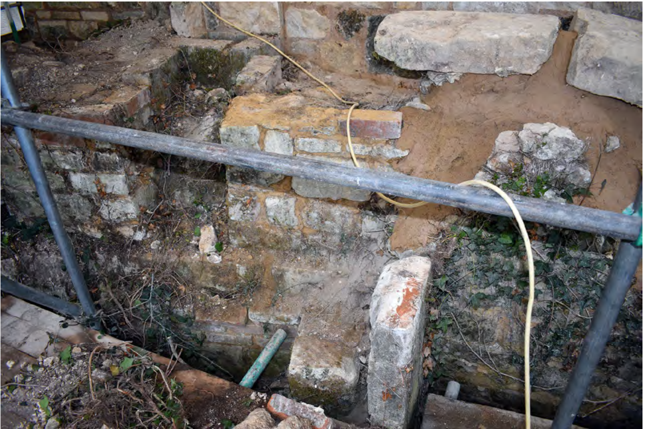
Plate 20: Location of former fireplace (not in section of wall to be dismantled)
