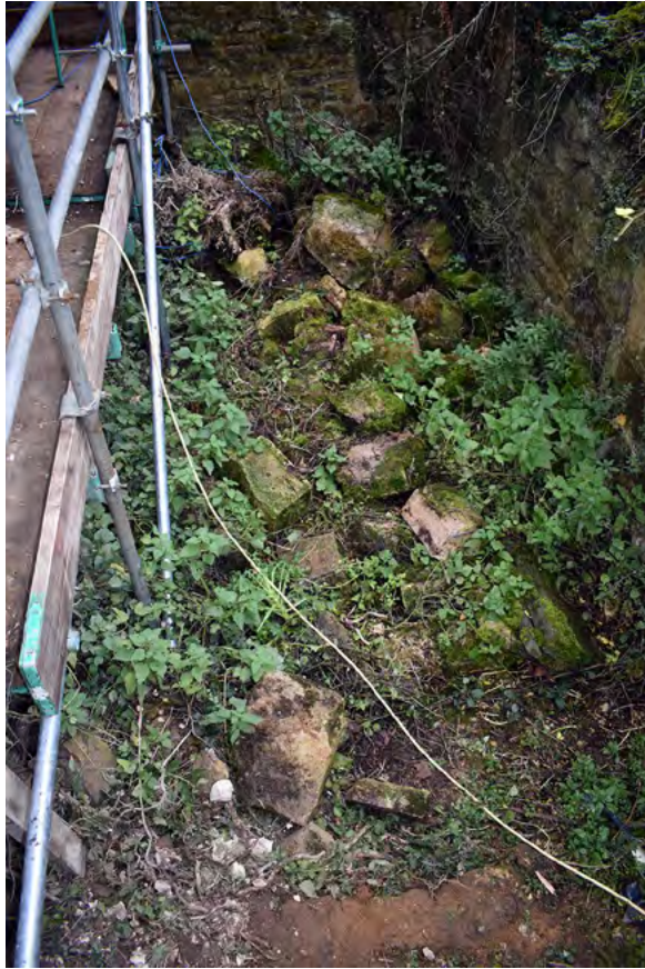
Plate 23: Collapsed stonework within former Prior's Lodgings (looking east)
