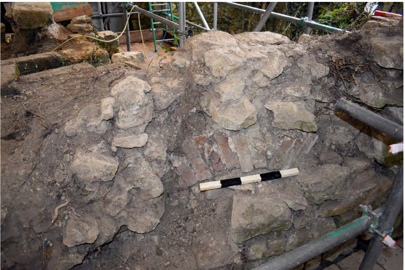
Plate 13: West side of wall during dismantling with rear of brick arch from oven visible
