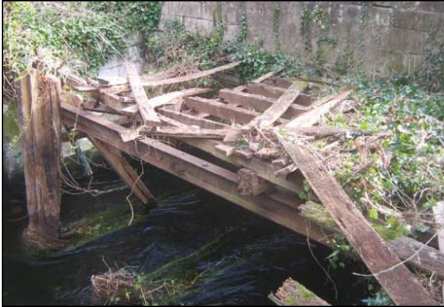
Plate 77: Abbey Mill Bridge, remains of deck to west of bridge
