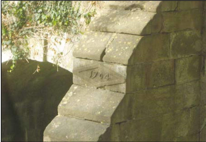
Plate 79: Abbey Mill Bridge, date stone in butters on east face of bridge
