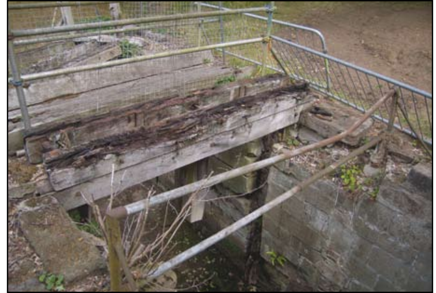
Plate 62: Gazebo Bridge, decayed remains of sluice gates
