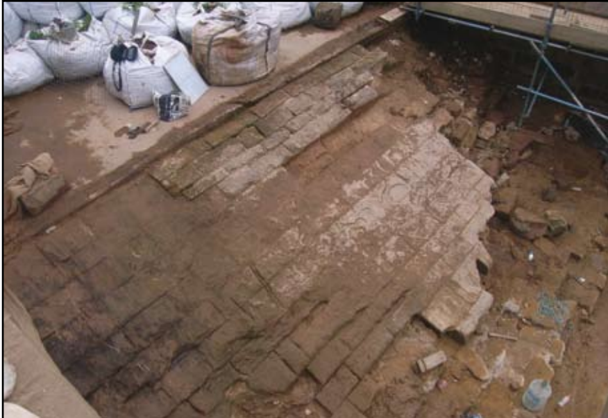
Plate 19: West Park Weir spillway before reconstruction
