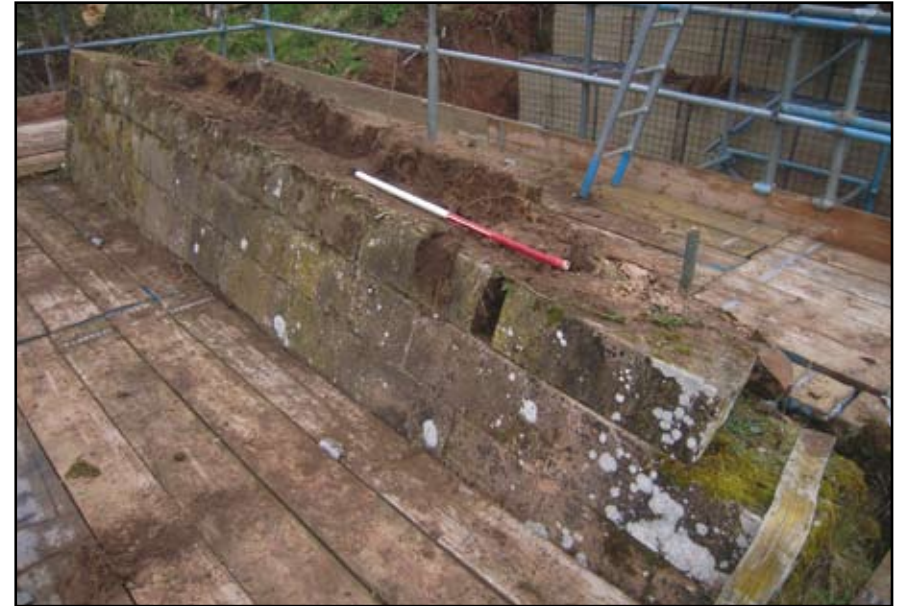
Plate 10: West Park Weir top of wall to west of weir during dismantling
