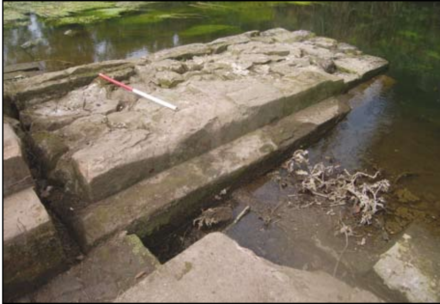
Plate 29: Island Weir, collapsed section of weir prior to works
