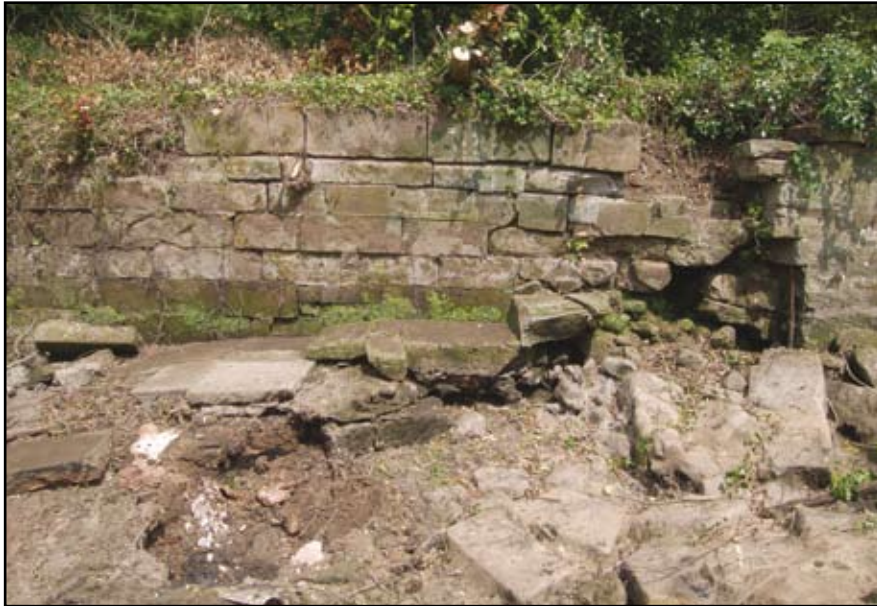
Plate 33: Island Weir, scar on north wall from lost weir
