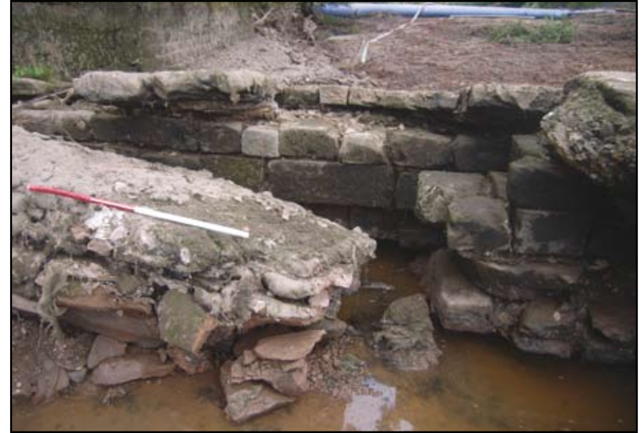
Plate 38: Island Weir, collapsed weir between upper and lower spillway
