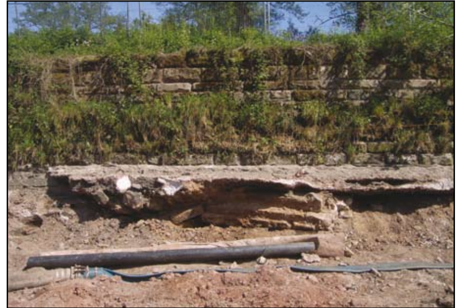
Plate 16: West Park Weir, east wall during works showing surviving block at base
