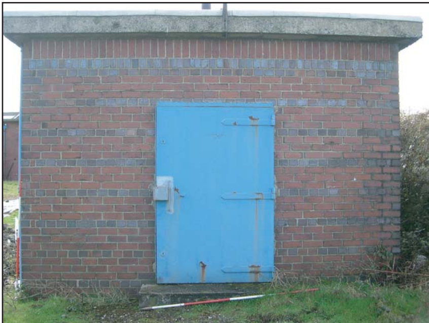
Plate 19: North-west end of substation
