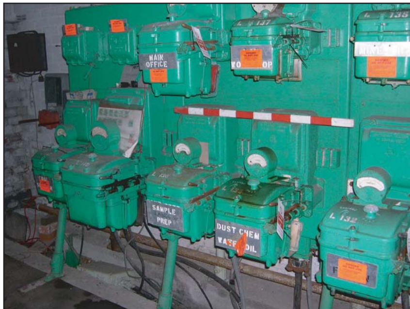
Plate 23: View of switchgear in substation
