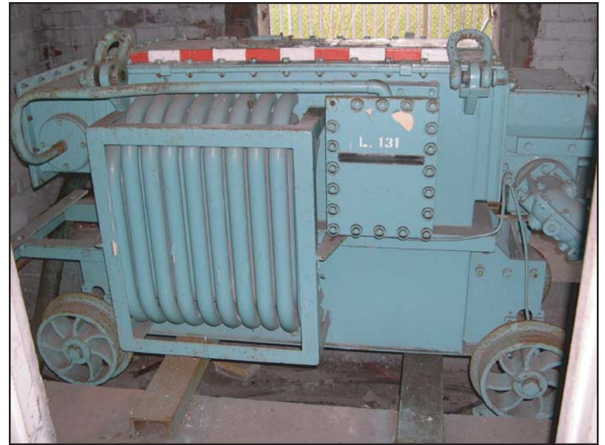
Plate 22: South-east face of transformer
