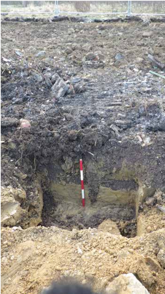
Plate 4: Foundation pad removed showing the exposed level of natural clay and the hard core rubble laid directly over this
