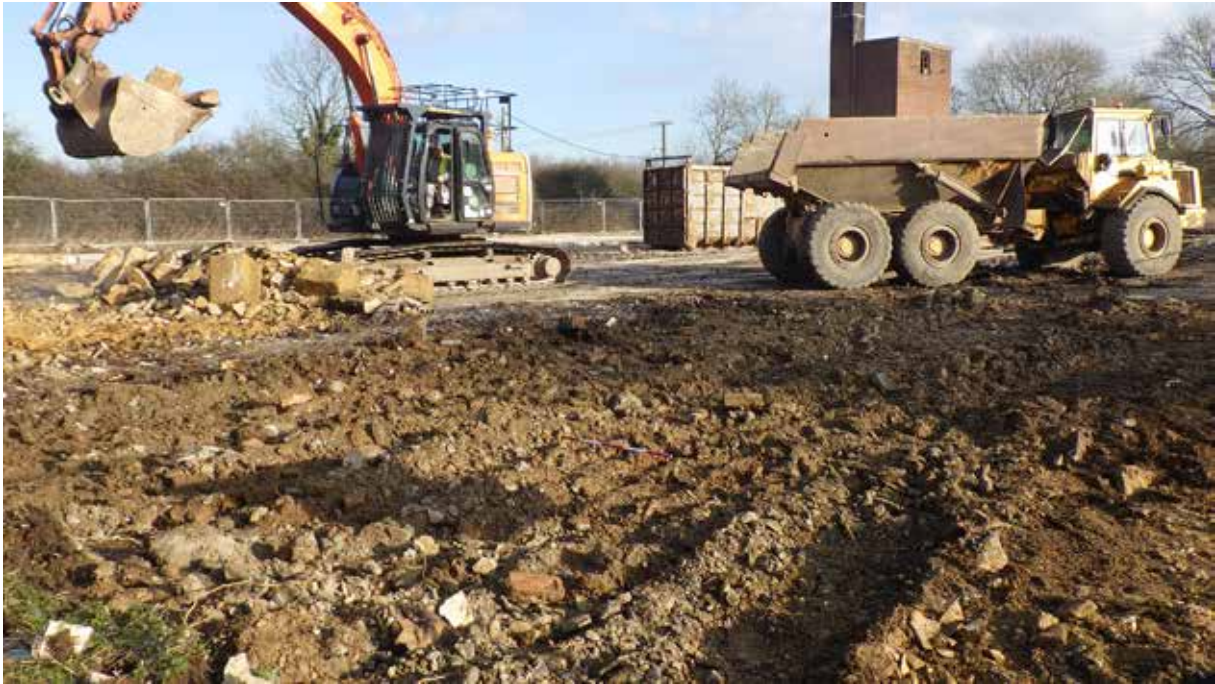
Plate 2: Rodney House concrete slab removal showing underlying hard core rubble and the limitation of plant to existing hard standing areas. View north
