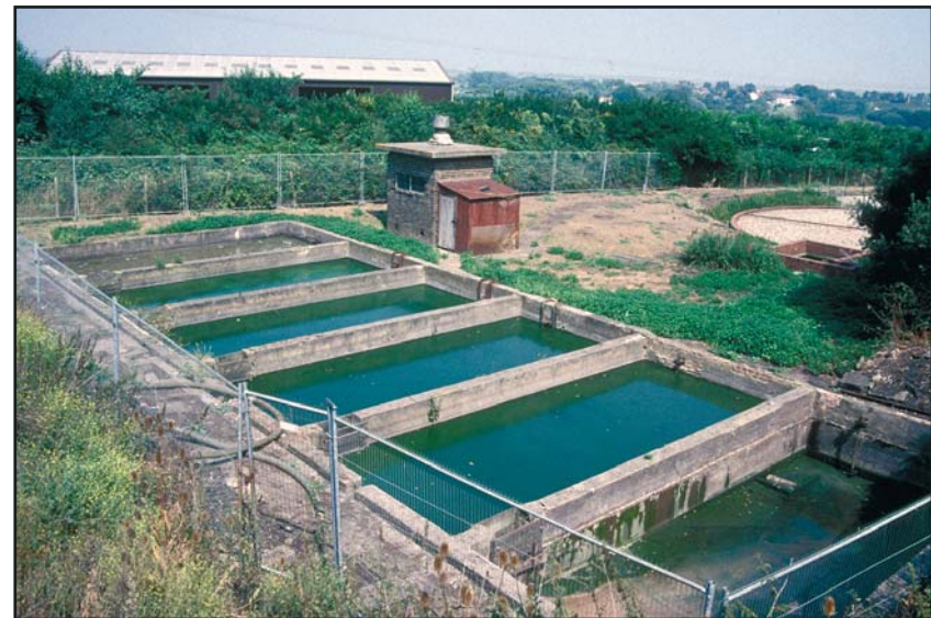
Plate 6: Settling tanks in the sewerage works
