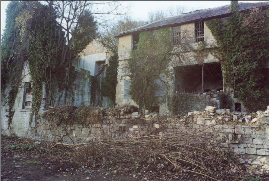
Plate 2: View from south with the platform of Building 3 in foreground (Building 4 to left) and Building 2 in the background
