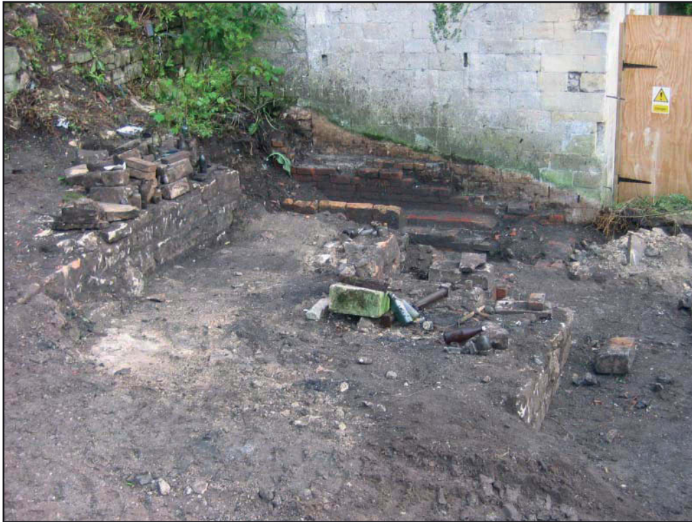
Plate 6: Structure 1 seen from the west. The stone walls and robbed floors of the terracing are evident in the foreground and the brick steam cabinet base in the background. The pre-excitation ground surface is still shown by the mark on the wall of Building 2 in the background
