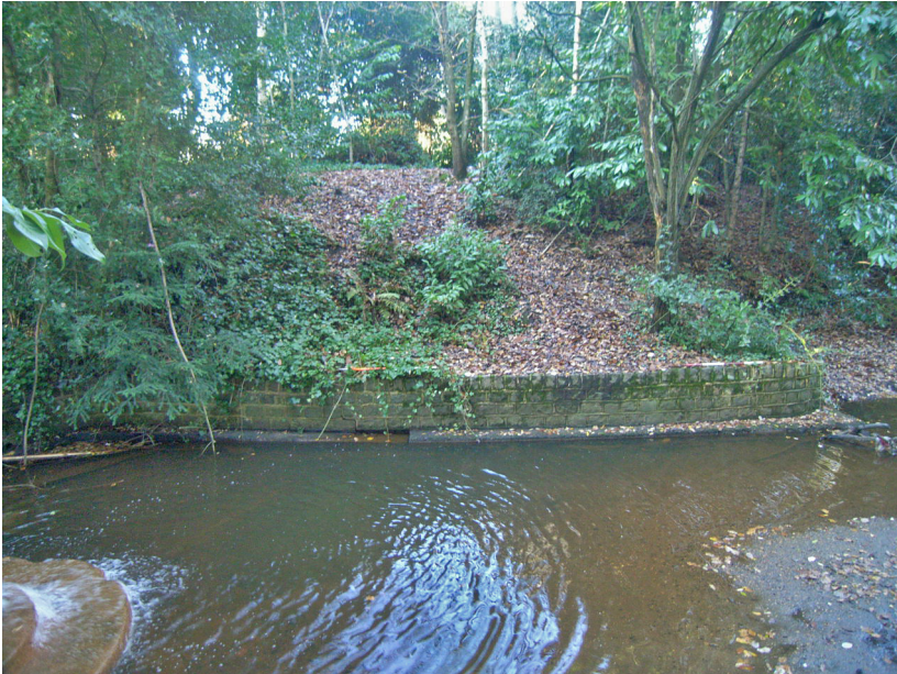
Plate 2: West wall of Southern inlet, showing subsidence
