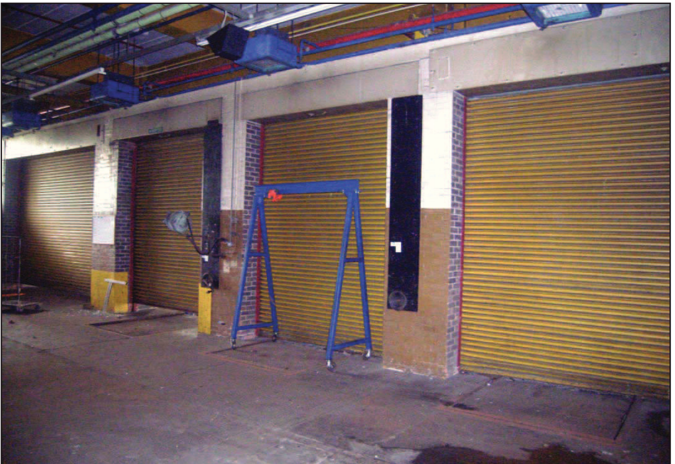
Plate 10: Loading bay at south end of ground floor despatch area (Block B)
