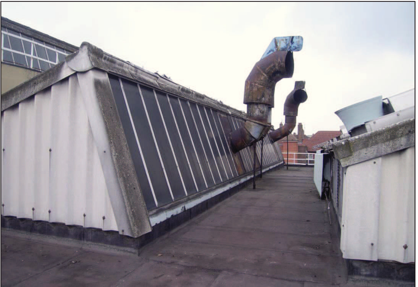
Plate 6: Roof lights above foundry showing extract ducts from zinc pots
