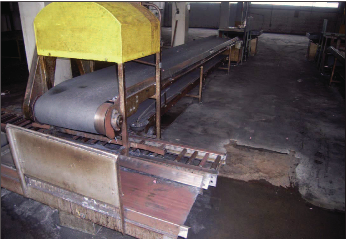
Plate 18: Conveyor in Fettling Dept (1st floor Block B)
