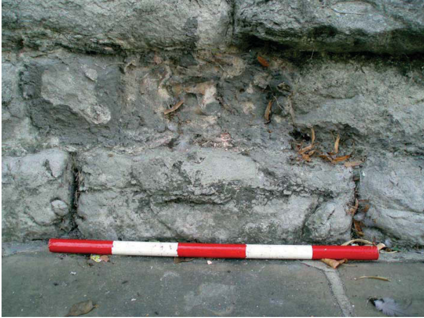
Plate 5: All Saints Vestry, Kingston: East elevation - rubble infill at base of elevation
