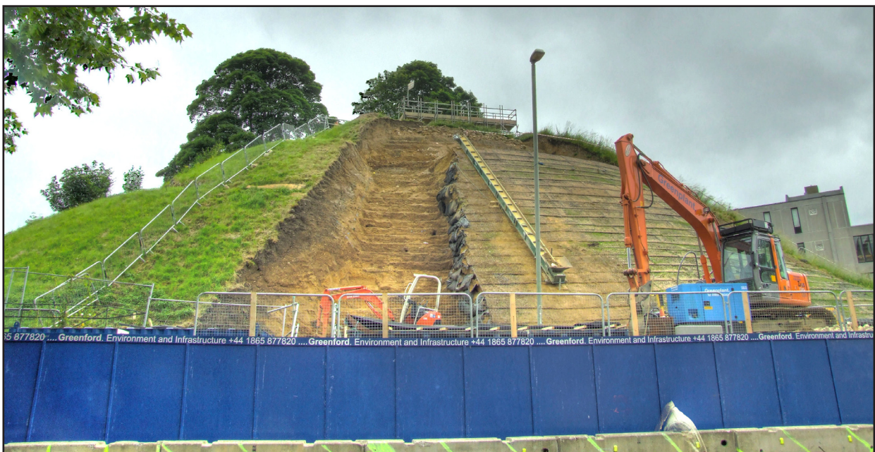
Plate 6: View of Gabions in place and their construction, wall visible at the top
