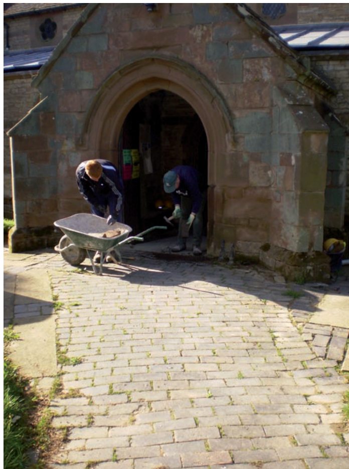
Plate 28: View south-east towards north porch, prior to the removal of the path (300)
