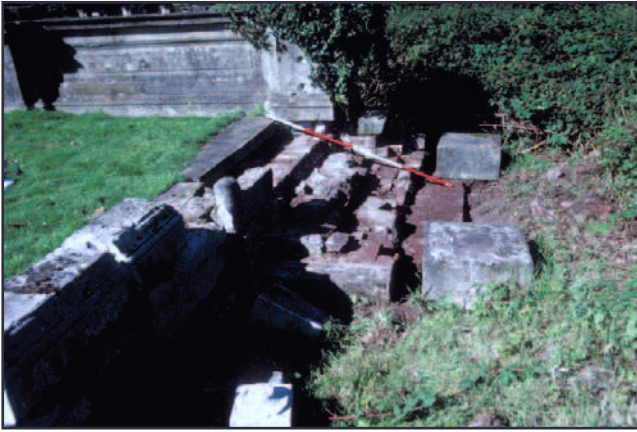
Plate 55 - Trench 102, shows current surviving state of step foundations S11 in East Parterre gardens. Looking north.
