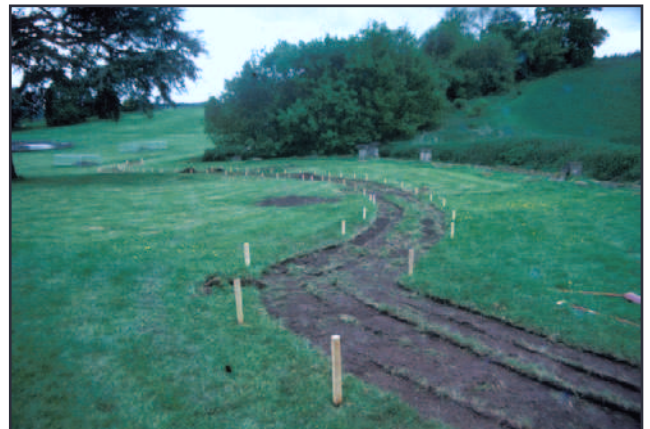
Plate 4 - Turf stripping commenced on new disabled access path at north west corner of South Parterre garden. Looking south east.
