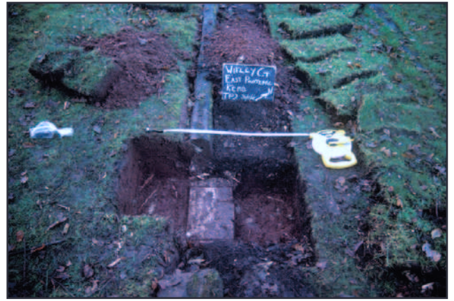
Plate 68 - Trial Pit 1 (East Parterre), examination of construction and survival of bed kerbing in east parterre. Looking north west.
