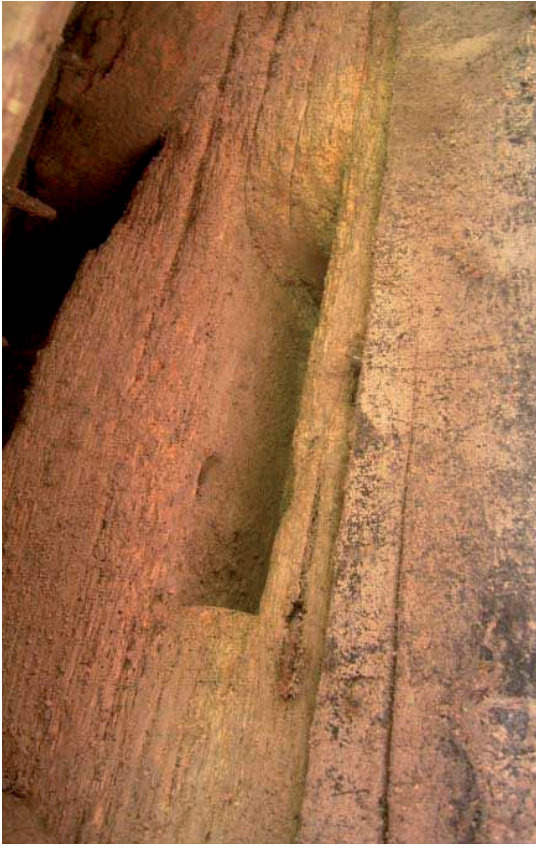
Plate 21: Chase mortise in face of wall plate, under eaves, from former projecting oriel
