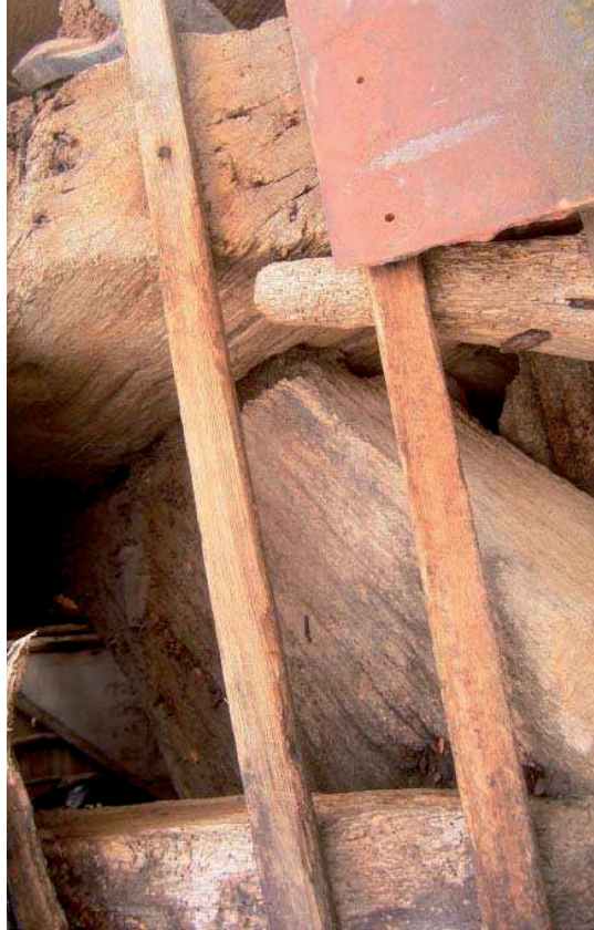
Plate 22: Curved corner brace and end of tie beam at E end of barn
