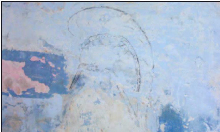
Figure 24: Graffiti on the western wall
