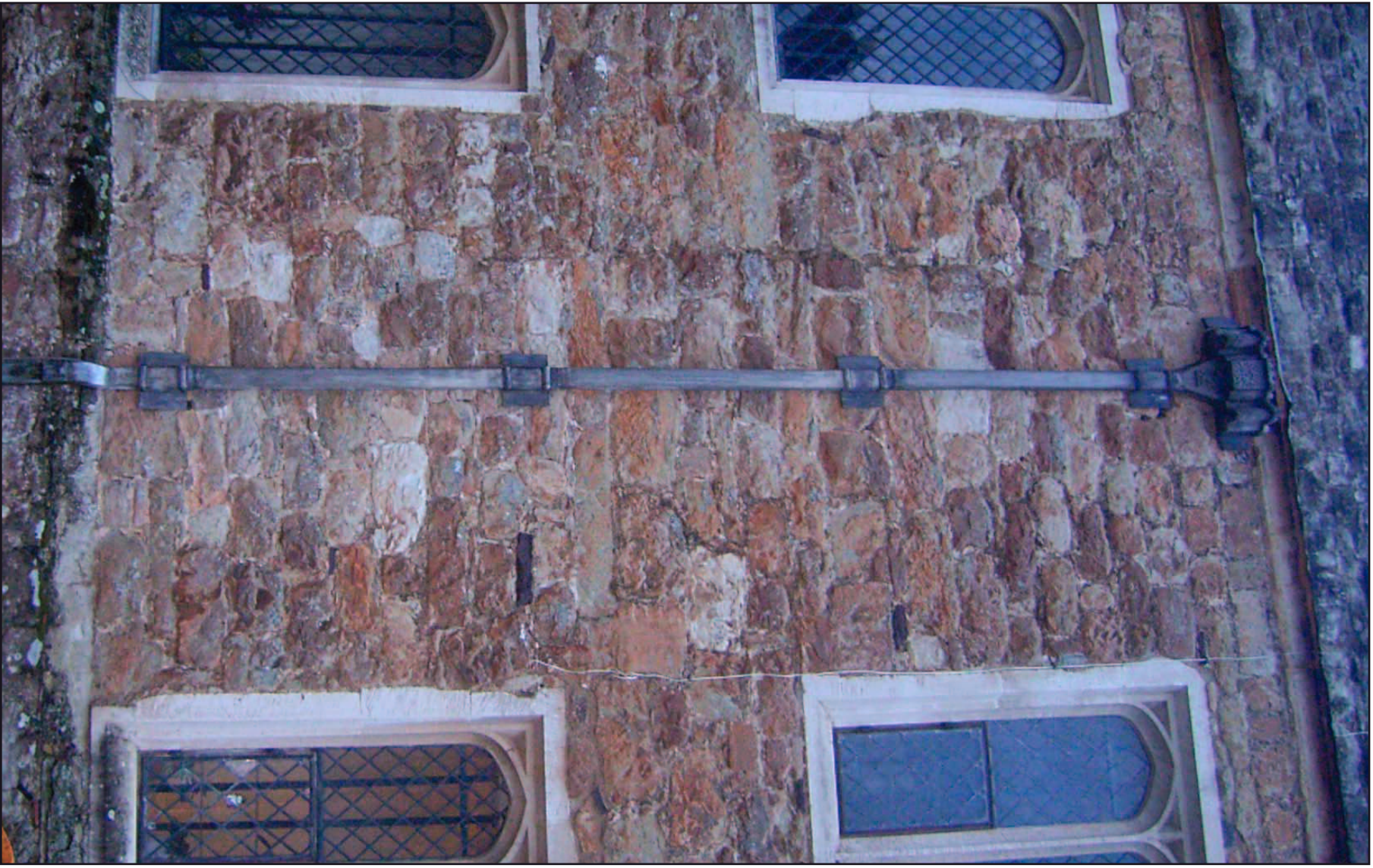
Plate 38. Vertical scar of a break in the east wall of the western range in Green Court
