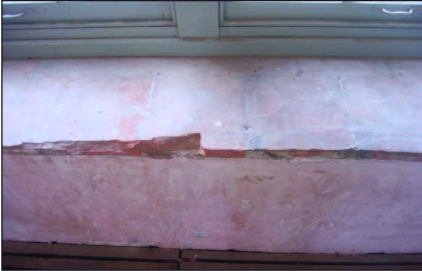
Figure 22: Sill of a window with some broken and some repaired tiles. South wall
