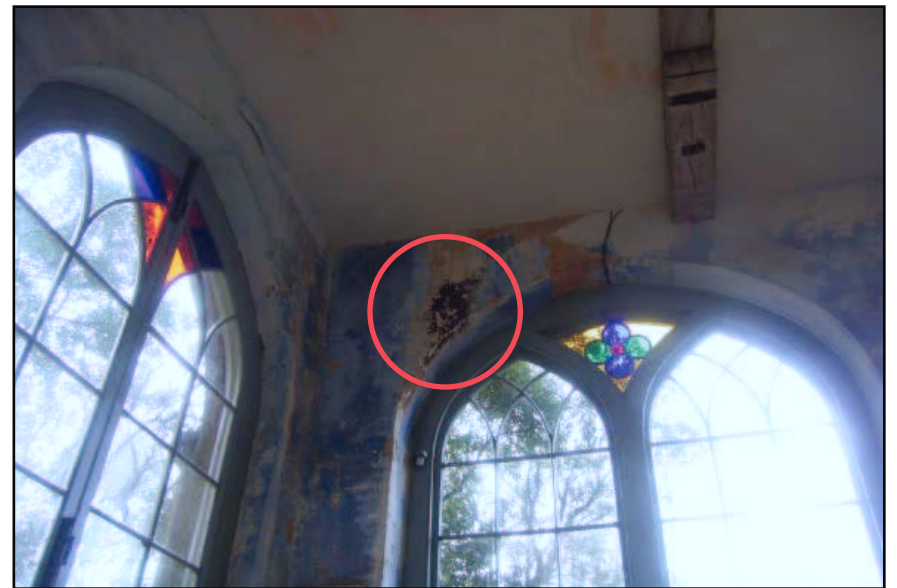
Figure 21: Black stain , probably due to fire in the inner arch of the easternmost window of the south wall
