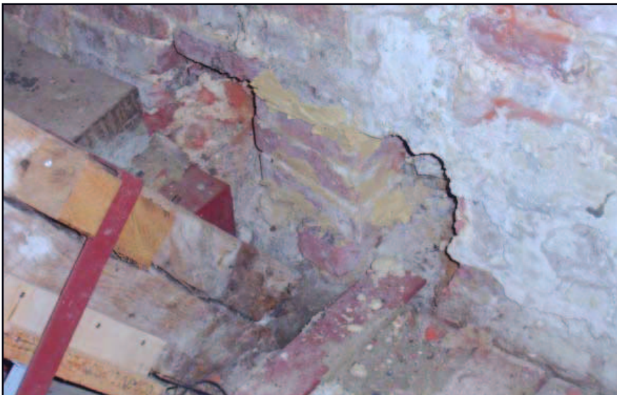
Figure 28: Recent metallic bracing for the tie beams and sockets in the wall
