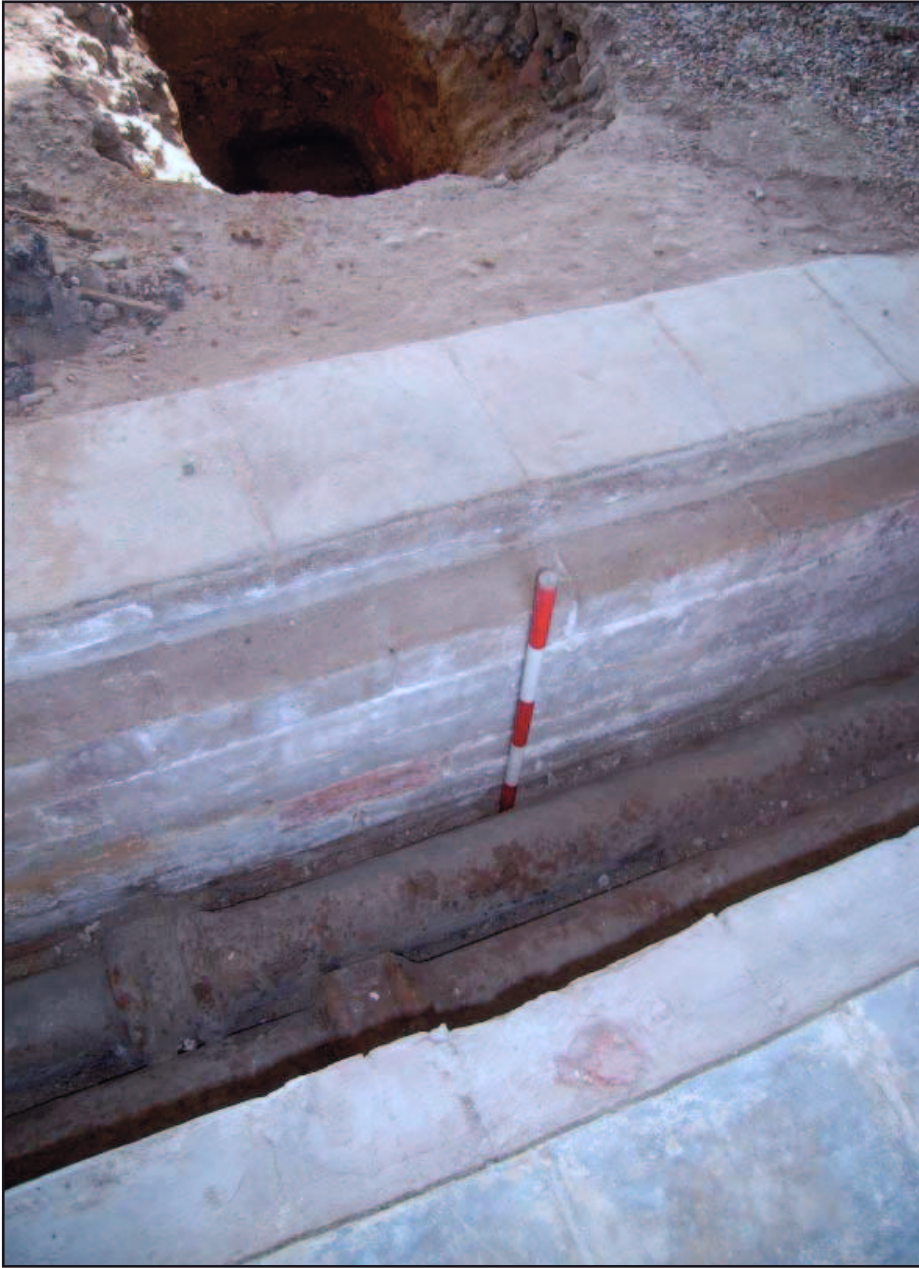
Plate 41: Heating pipes within duct/trench along north wall of Orangery
