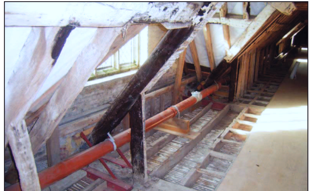
Plate 33: Blackened timbers due to fire
