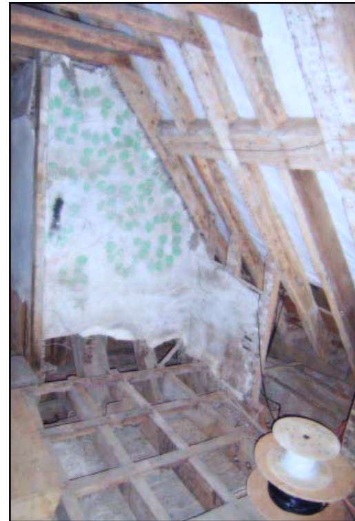
Figure 27: Remains of the decorated plaster on the west wall
