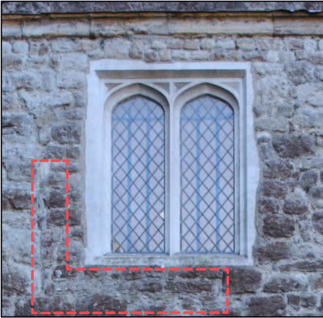
Plate 8a: Straight joints in the eastern end of the north facade (first floor) suggesting alterations to the fenestration. Easternmost window
