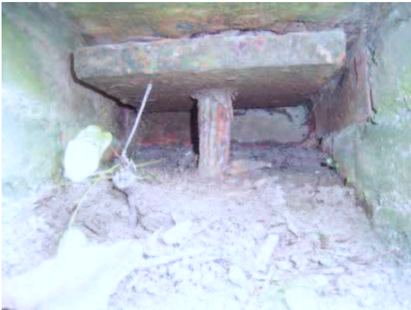
Plate 7: Bolt within access void beneath lower stone in north face of wall
