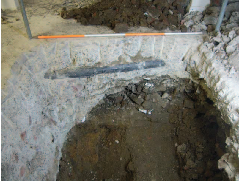
Plate 4: Test Pit 4 - Brick filled void beneath concrete slab
