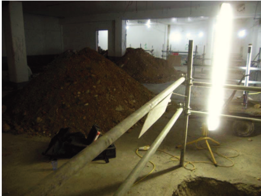
Plate 4: General view of test pit works in the basement of 18 Hanover Square, looking west
