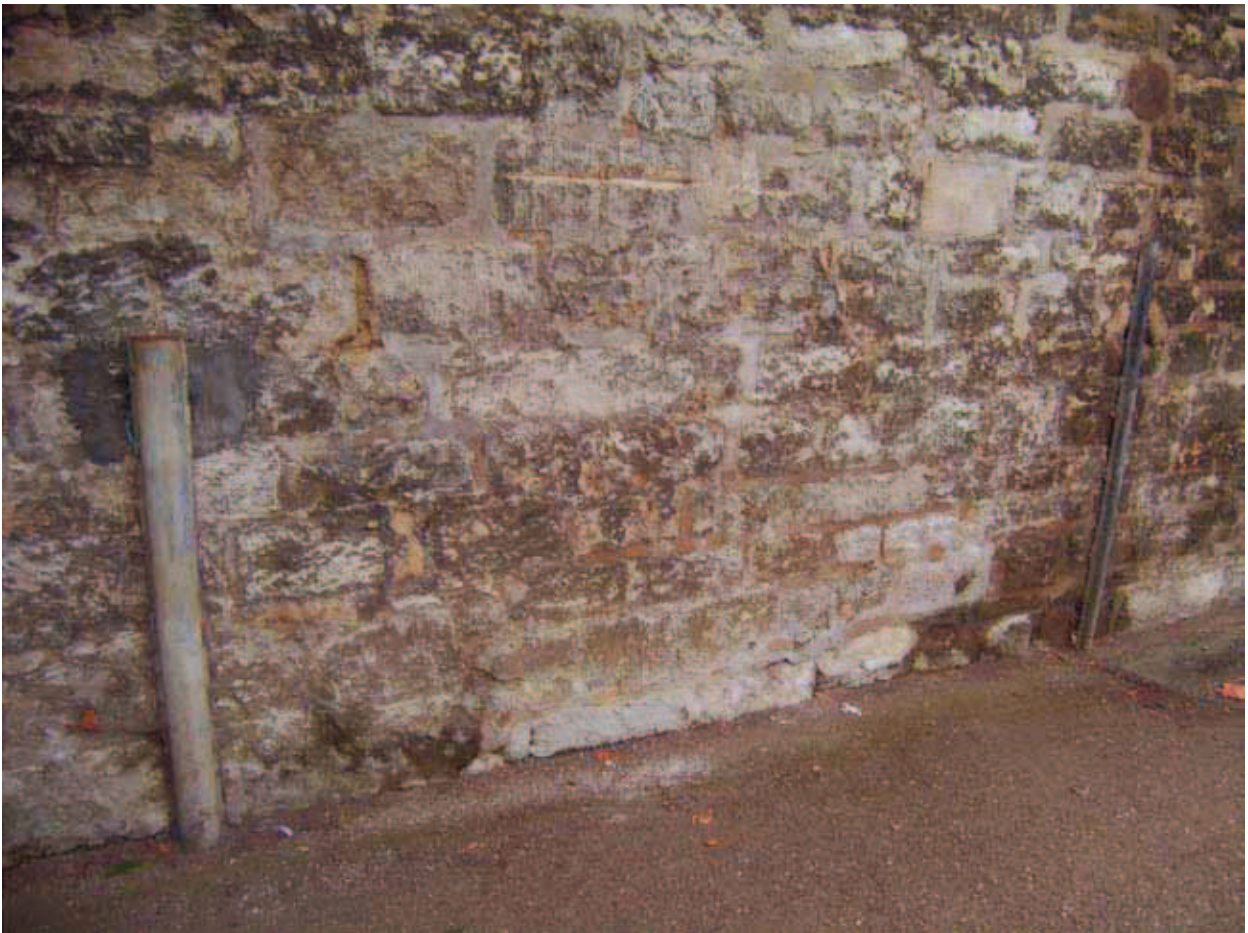
Plate 4: President's Lodgings Wall, Magdalen College: Steel supports on north face, looking south
