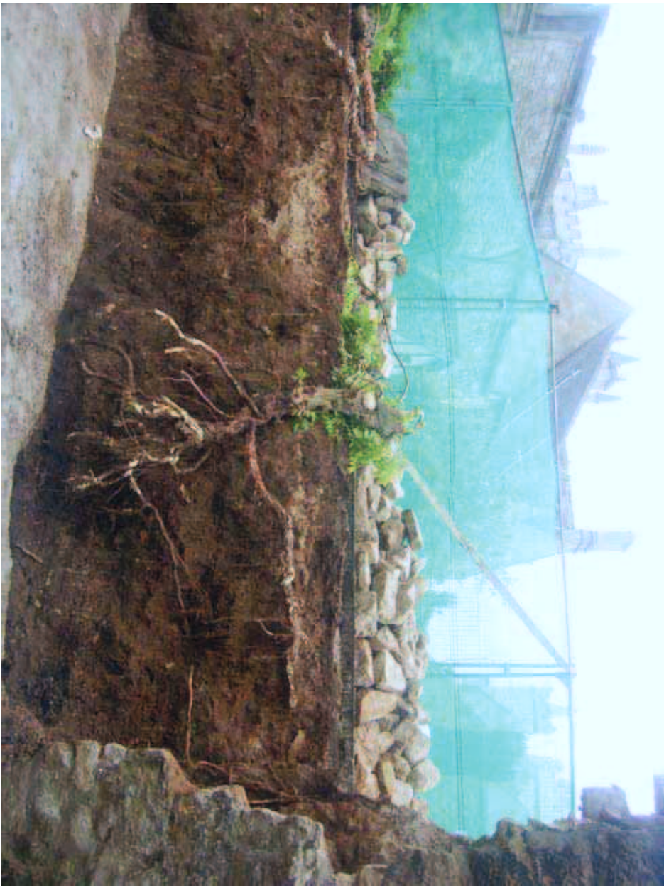
Plate 11 : President's Lodgings Wall, Magdalen College: area of wall after dismantling, looking south
