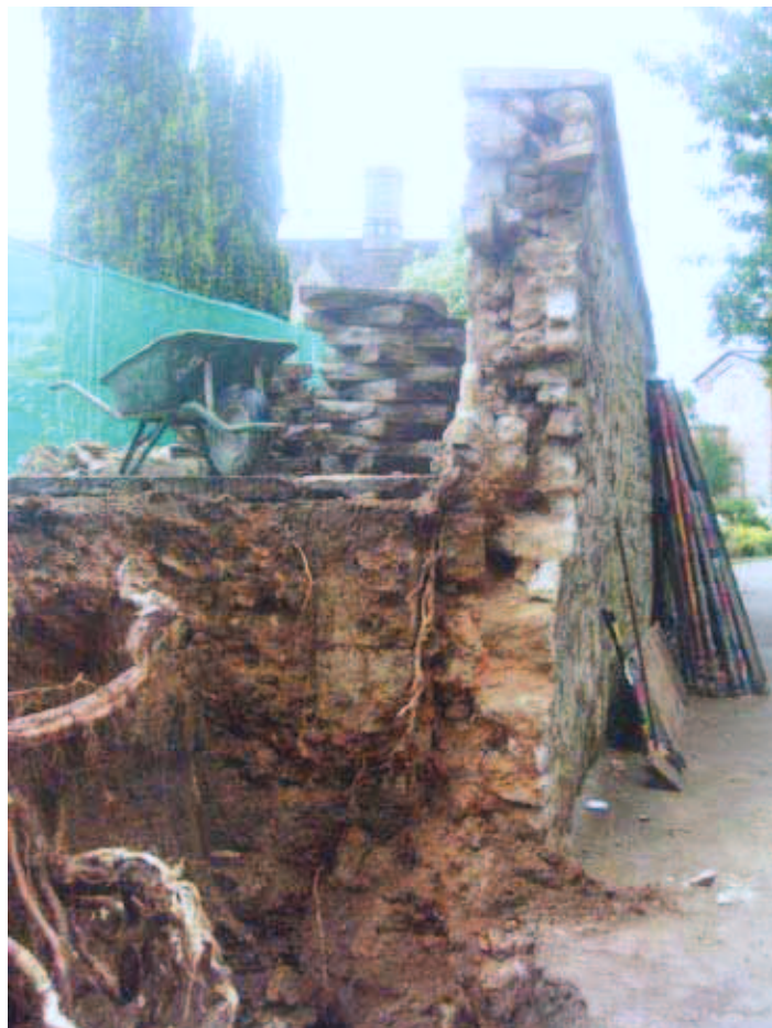
Plate 10: President's Lodgings Wall, Magdalen College: Section of wall after dismantling, looking west
