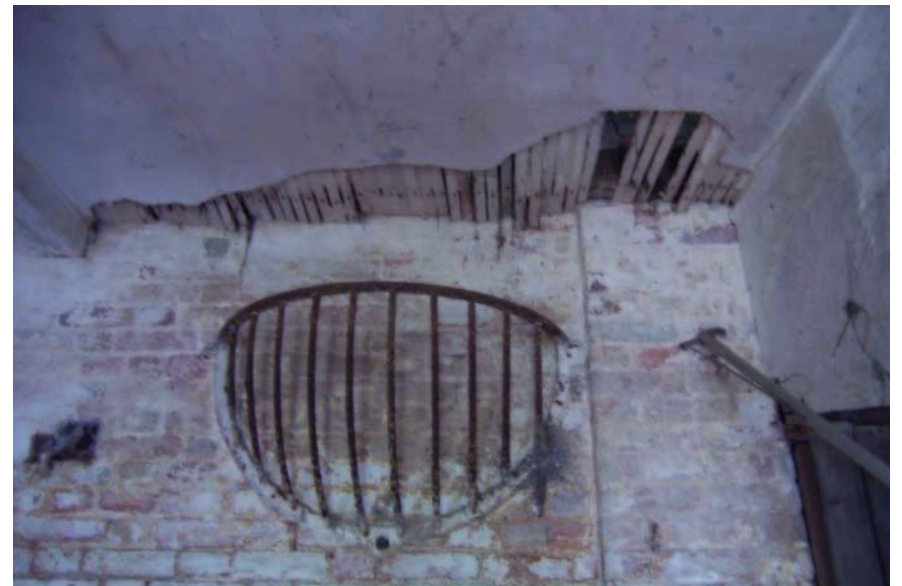
Plate 92: Exposed plaster and lathes in roof of stable
