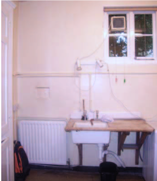
Plate 25: Butler sink, utility room
