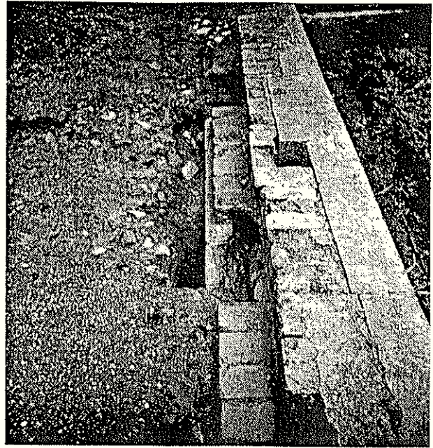
Figure Twenty: Hole showing position of removed vertical pipe in Trench G
