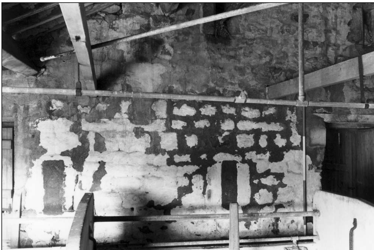
Photo 19: Blocked vents in south gable of aisled barn, now facing into south extension
