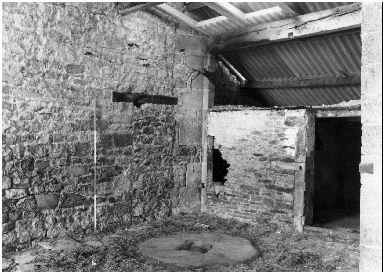
Photo 22: Interior view of west cart entry to aisled barn, with millstone embedded in threshing floor
