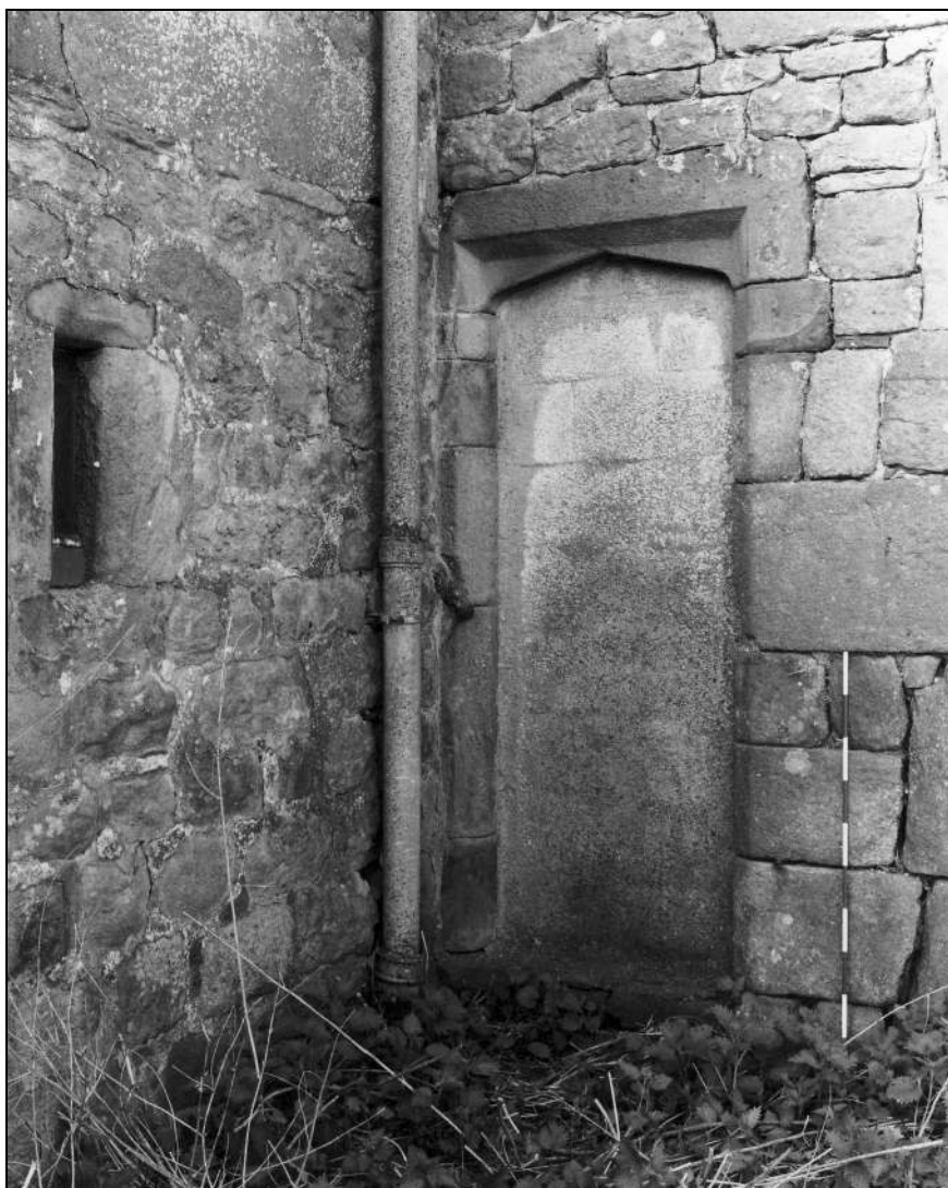
Photo 6: Blocked pedestrian doorway next to east cart entry
