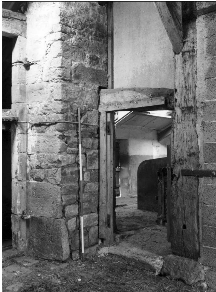
Photo 30: Lower part of arcade post and end of aisle tie, by west cart entry
