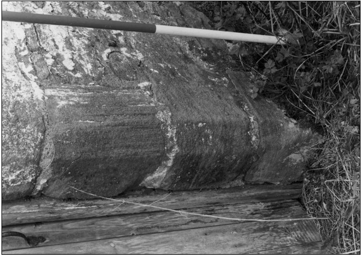
Photo 15: Detail of chamfer and stop to doorway in north elevation (film 1, frame 13)
