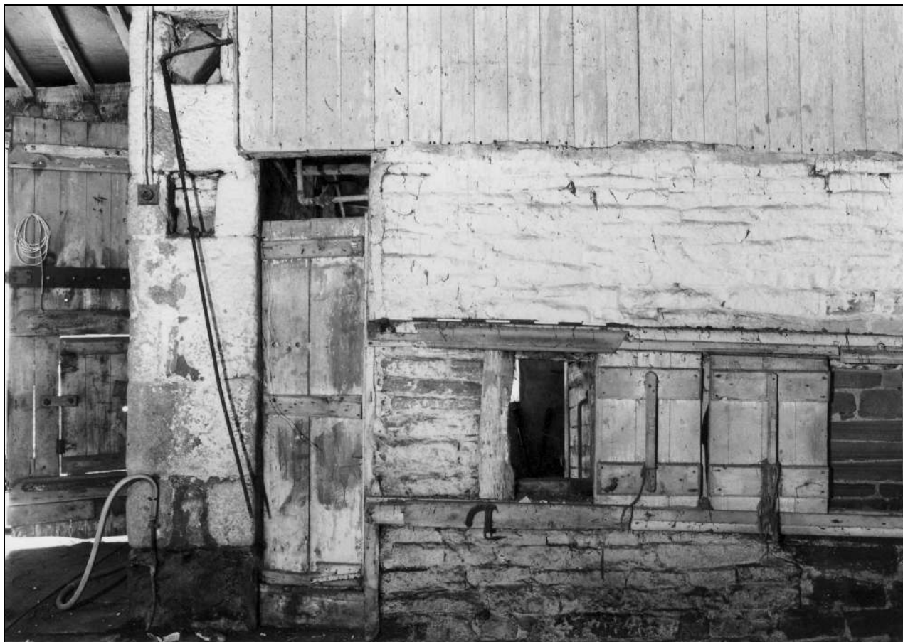
Photo 22: Stone wall and partition to south-west outshut, from the north (film 4, frame 4)
