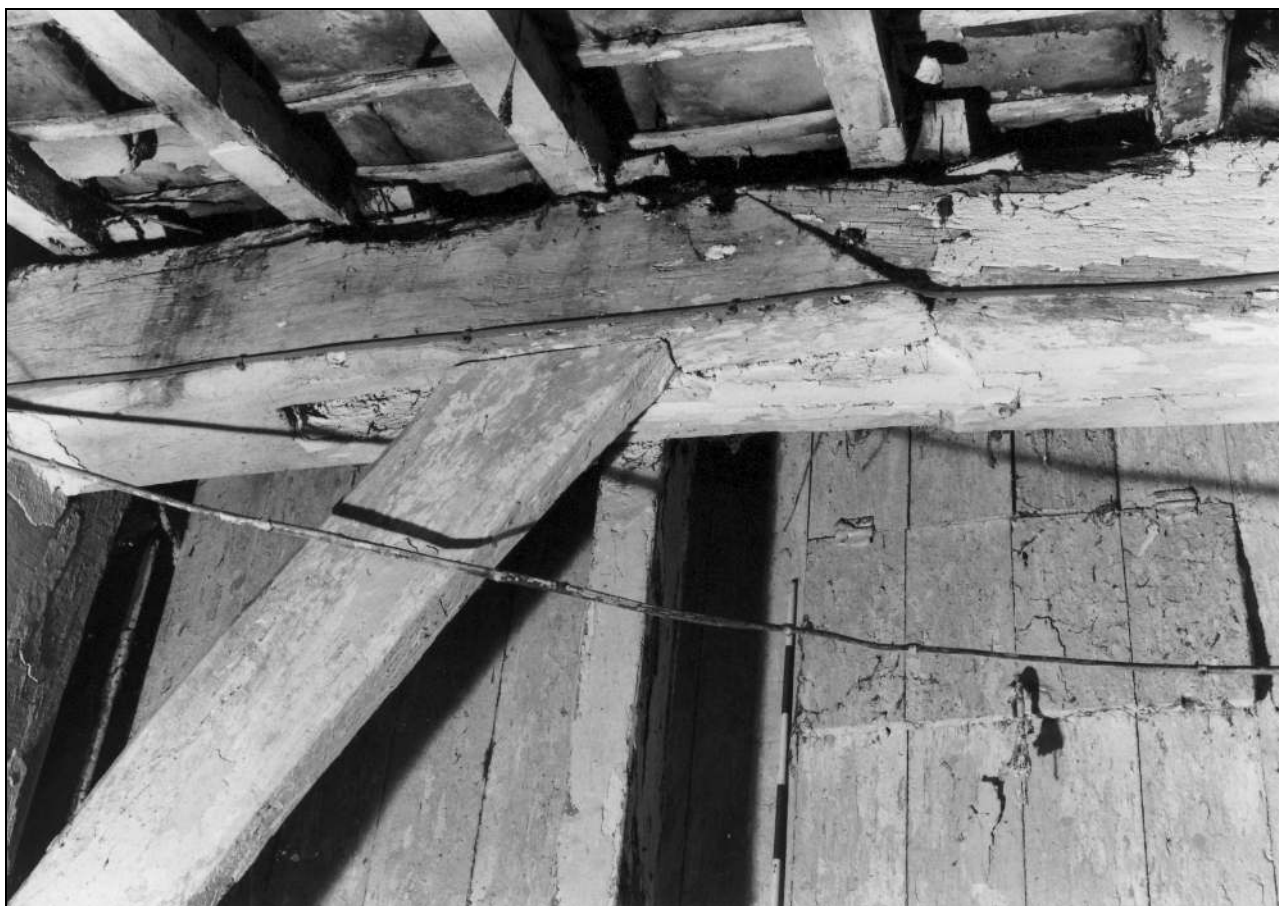
Photo 45: Scarf joint in arcade plate, east of arcade post, from the south (film 3, frame 4)
