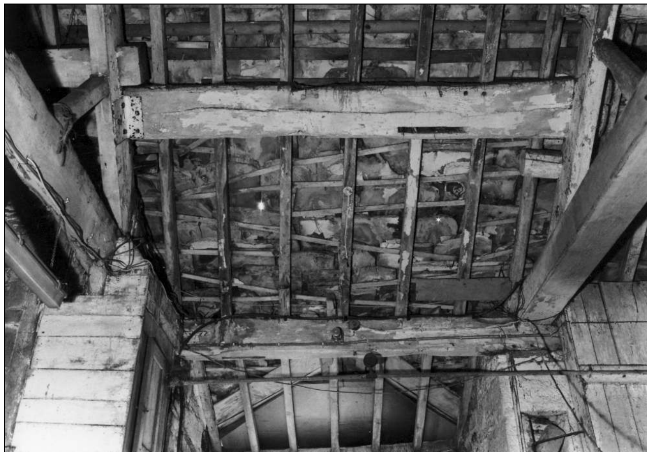
Photo 53: Purlin and arcade plate over entrance bay, from the north (film 4, frame 6)
