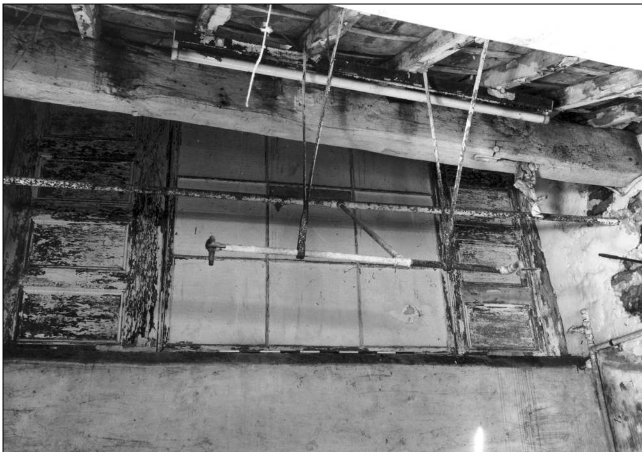
Photo 35: Plank partition to north side of south-west outshut, and arcade plate overhead (film 2, frame 2)
