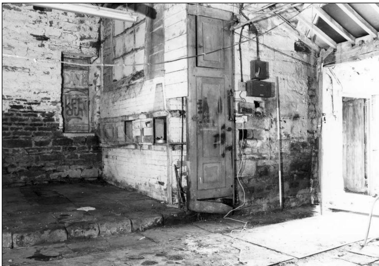
Photo 23: Interior of the barn, from the north-west, showing brick wall to south-east outshut (film 3, frame 11)
