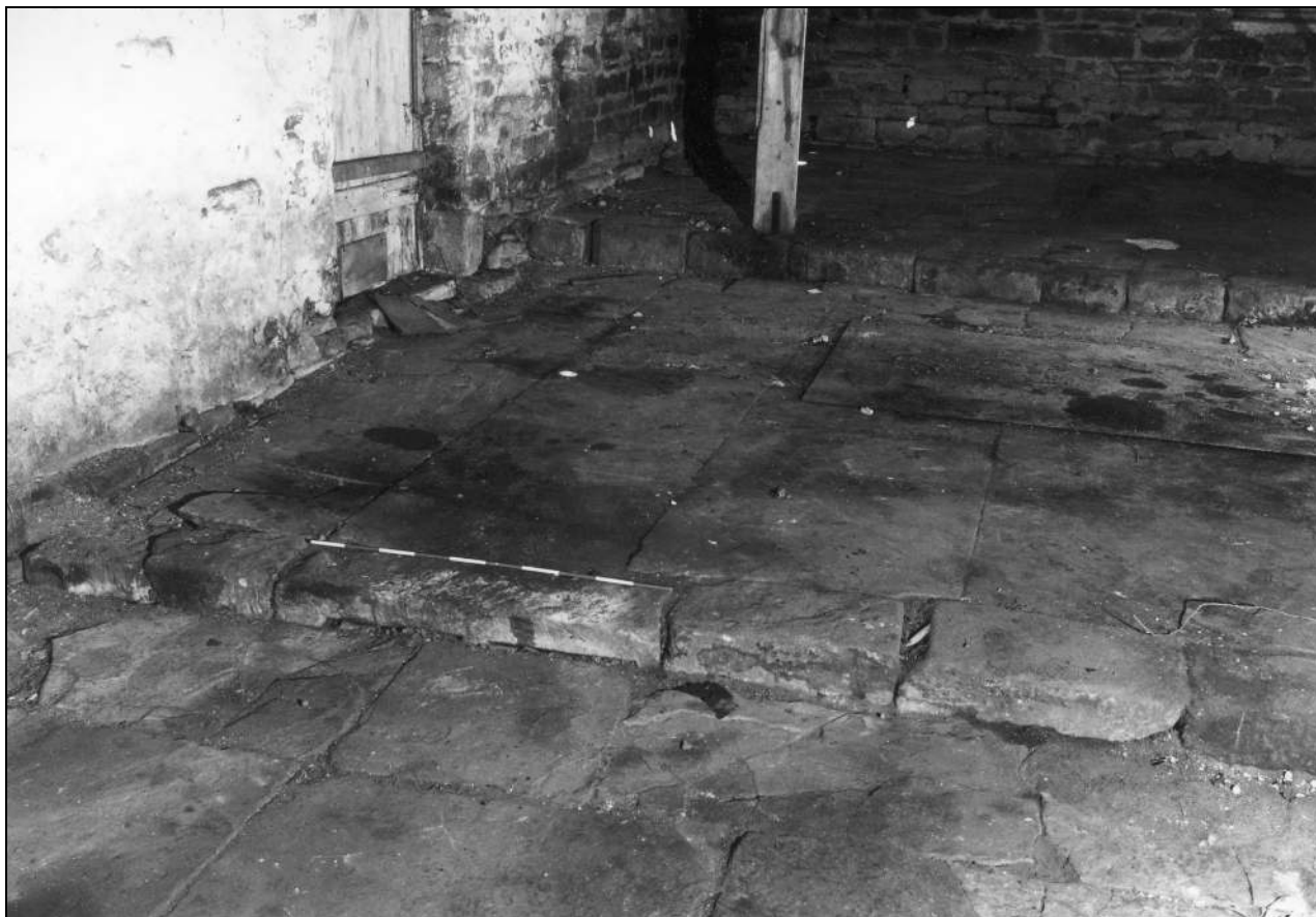
Photo 20: Flagged floor of barn, with re-used sill or lintel in kerb (film 4, frame 11)
