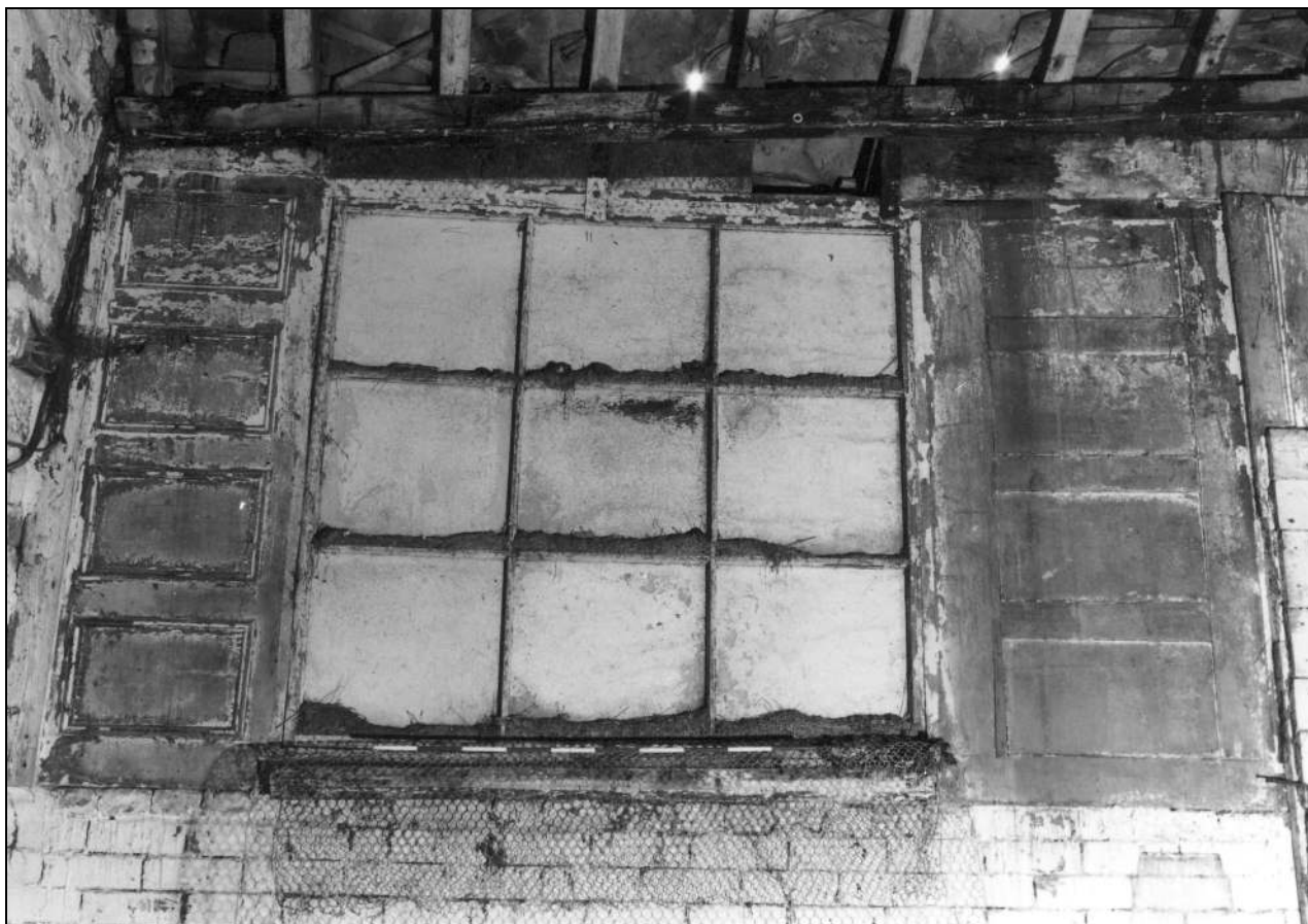
Photo 25: Re-used panelling forming partition to south-east outshut, from the north (film 3, frame 12)
