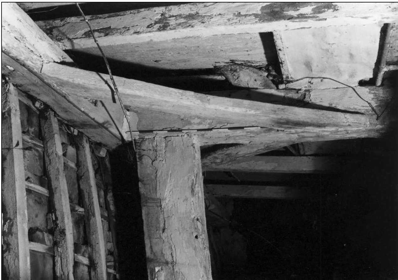
Photo 44: End of aisle rafter and east arcade brace, from the east (film 2, frame 18)
