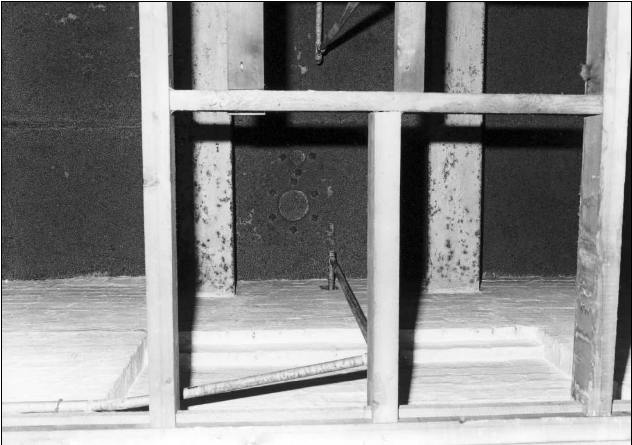
Photo 51: Bay 3: base of tank, with gas pipes for lighting (film 4, frame 6)
