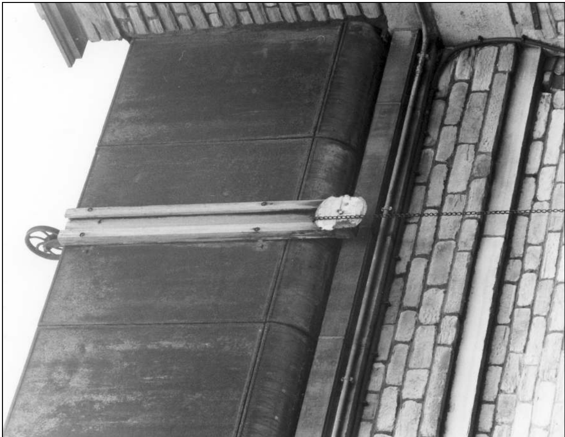
Photo 71: Level gauge on west side of tank (film 1, frame 17)
