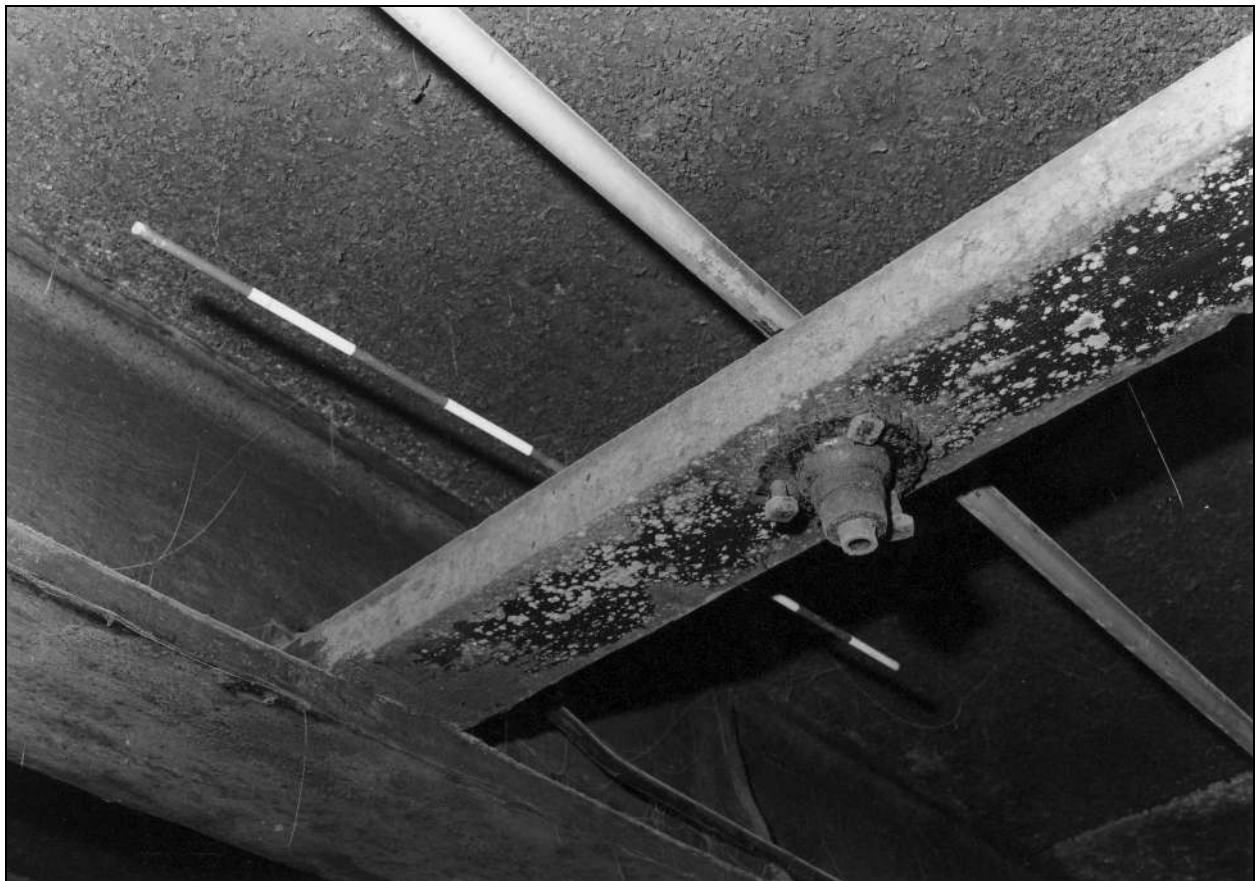
Photo 50: Bay 4: gas light fitting, below base of tank (film 8, frame 4)
