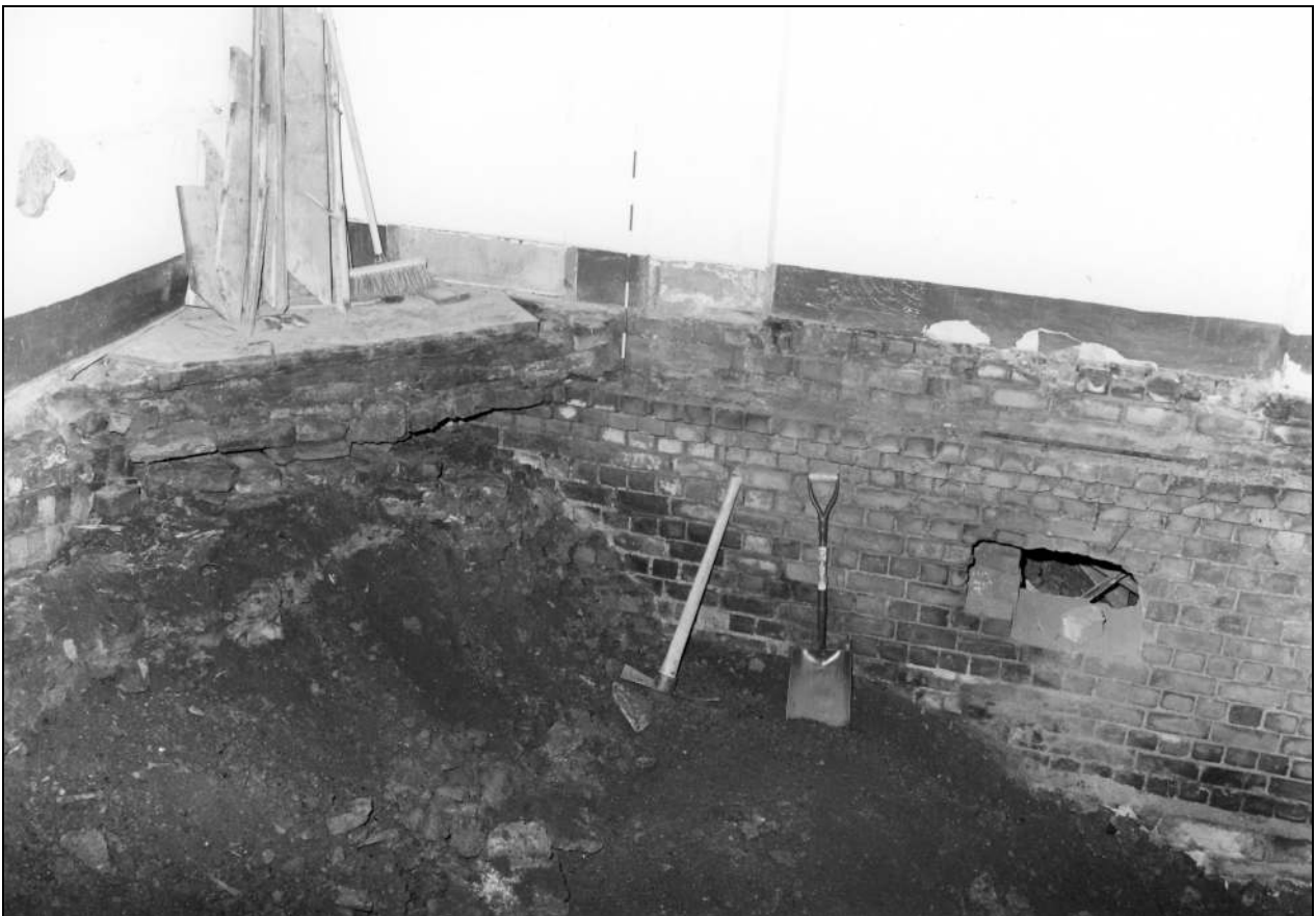
Photo 24: Bay 2: north-west corner, showing hearth for corner fireplace, during refurbishment (film 5, frame 9)
