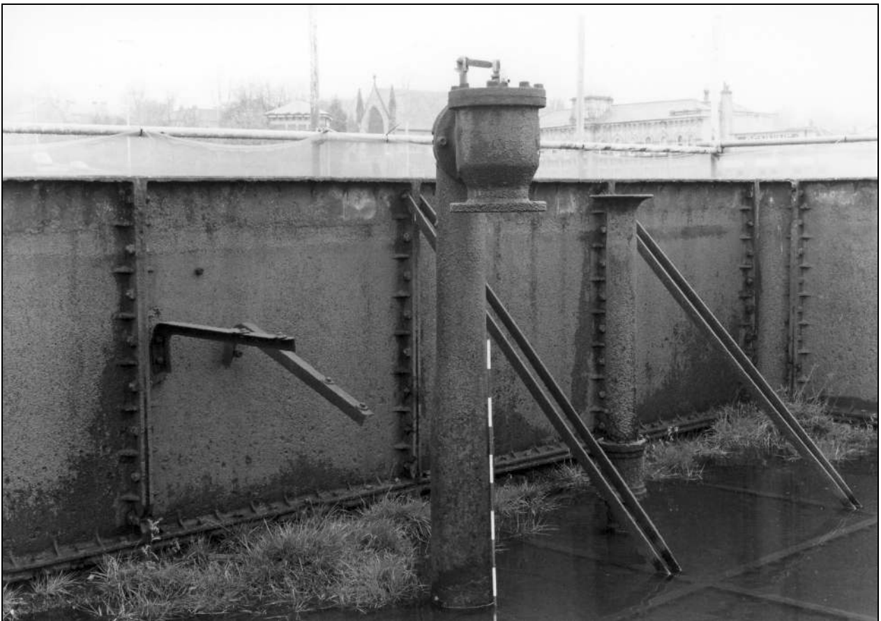
Photo 68: Later feed, and overflow pipes, within tank, from the south-east (film 7, frame 2)
