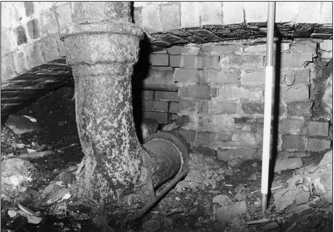
Photo 44: Bay 4: later feed pipe, emerging from west side below ground floor level (film 4, frame 5)
