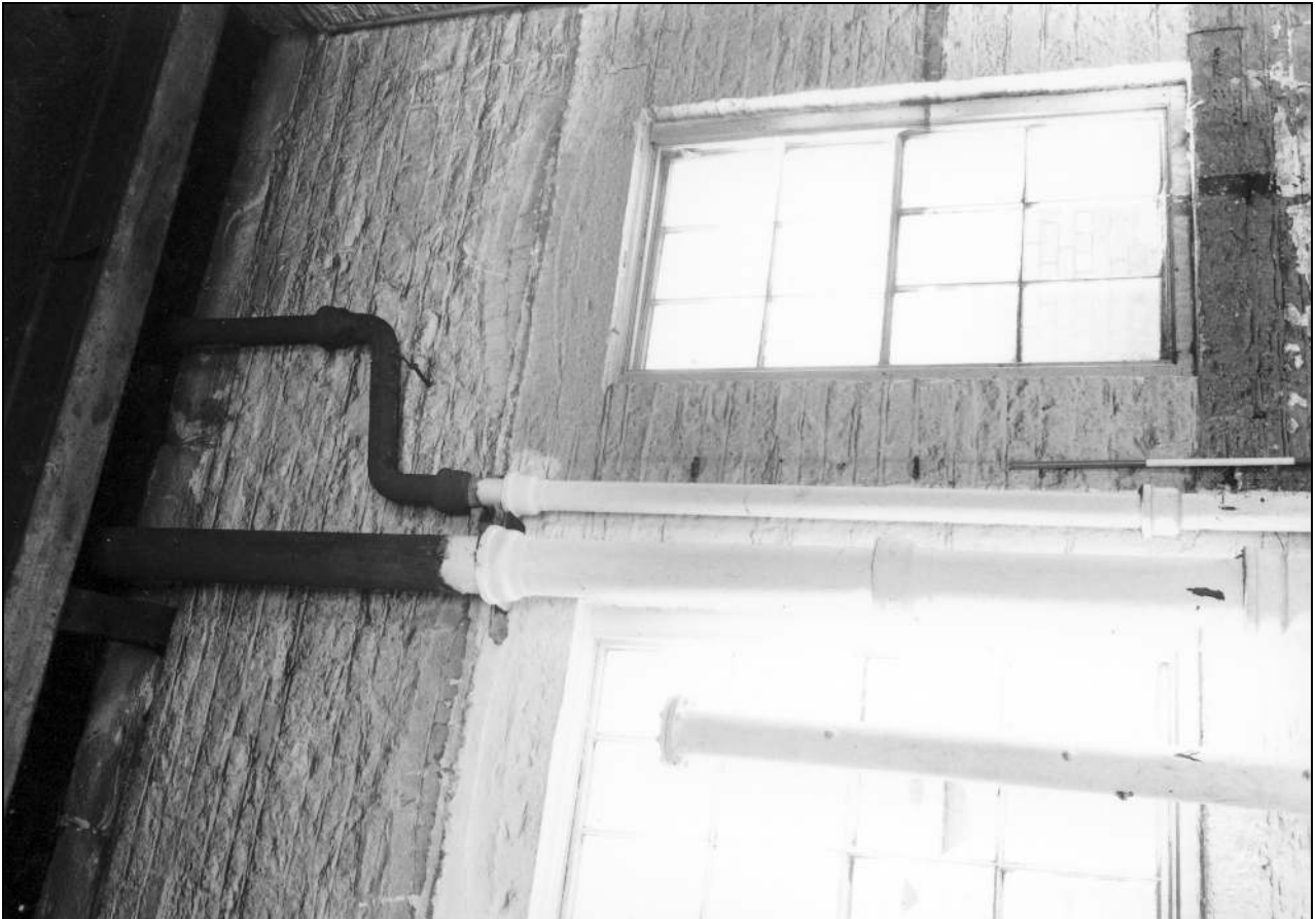
Photo 39: Bay 4: pipes in west side (overflow and later feed, nos 1, 2 & 3) (film 4, frame 3)
