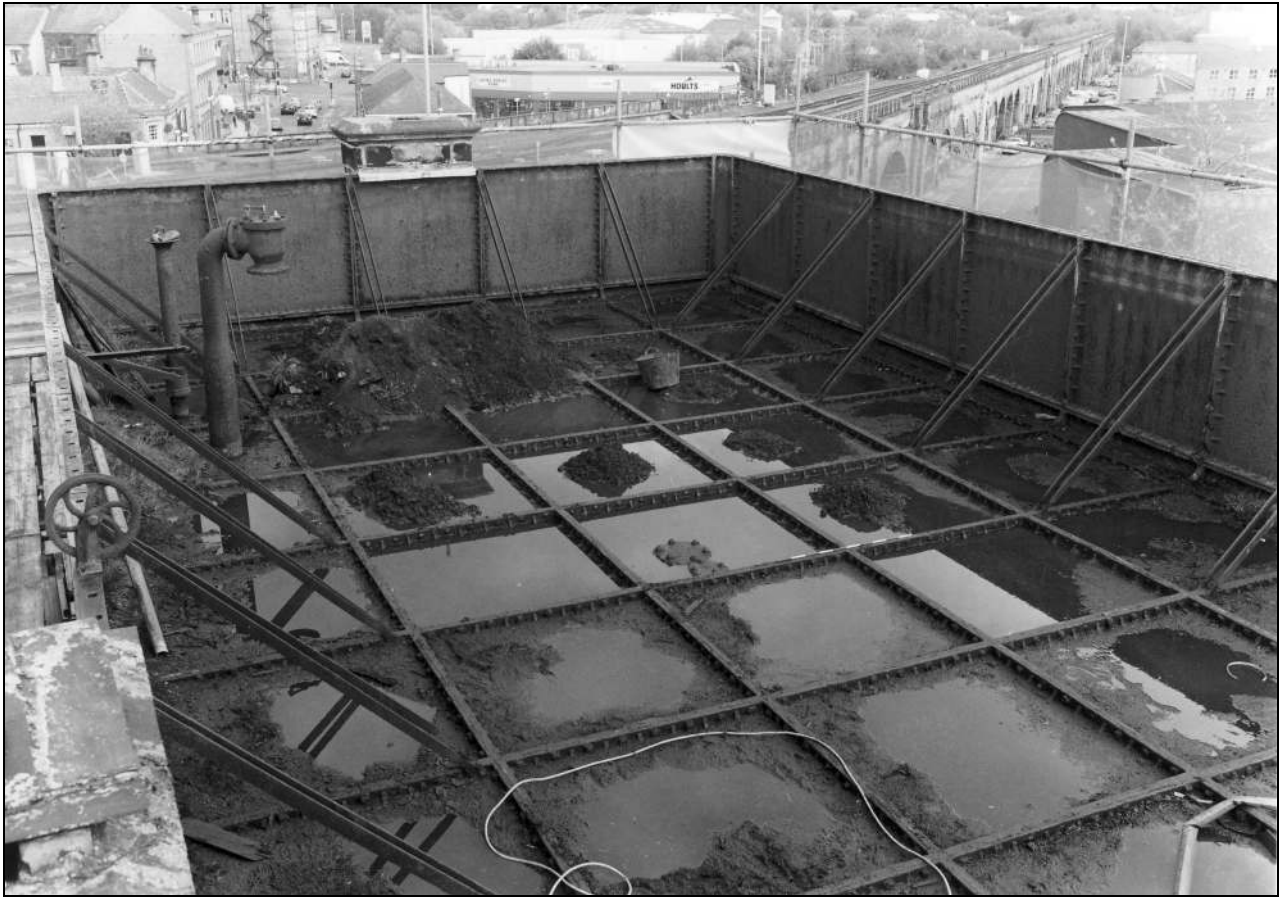
Photo 63: General view of the tank, from the south-west, during repairs (film 8, frame 7)
