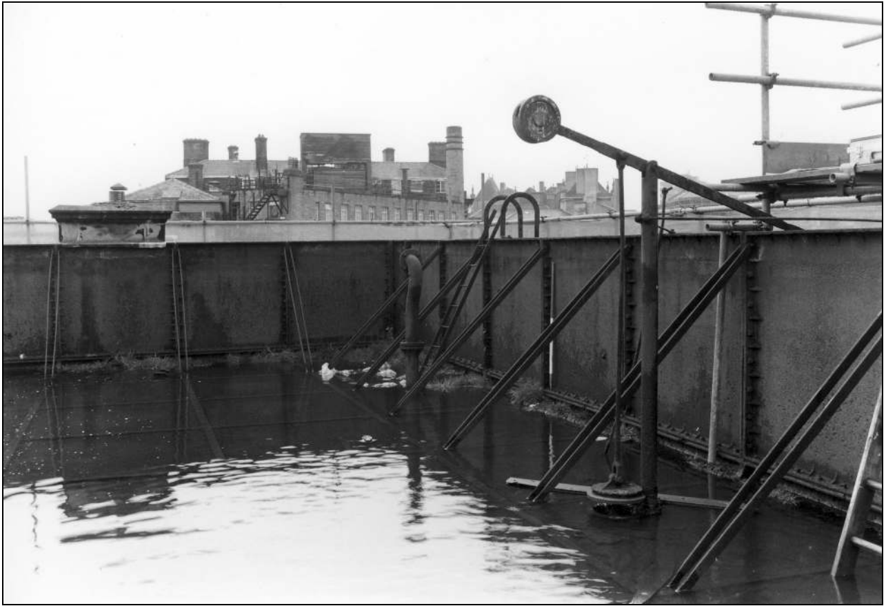
Photo 75: Detail of outlet pipe at base of tank, with stopper (film 6, frame 12)
