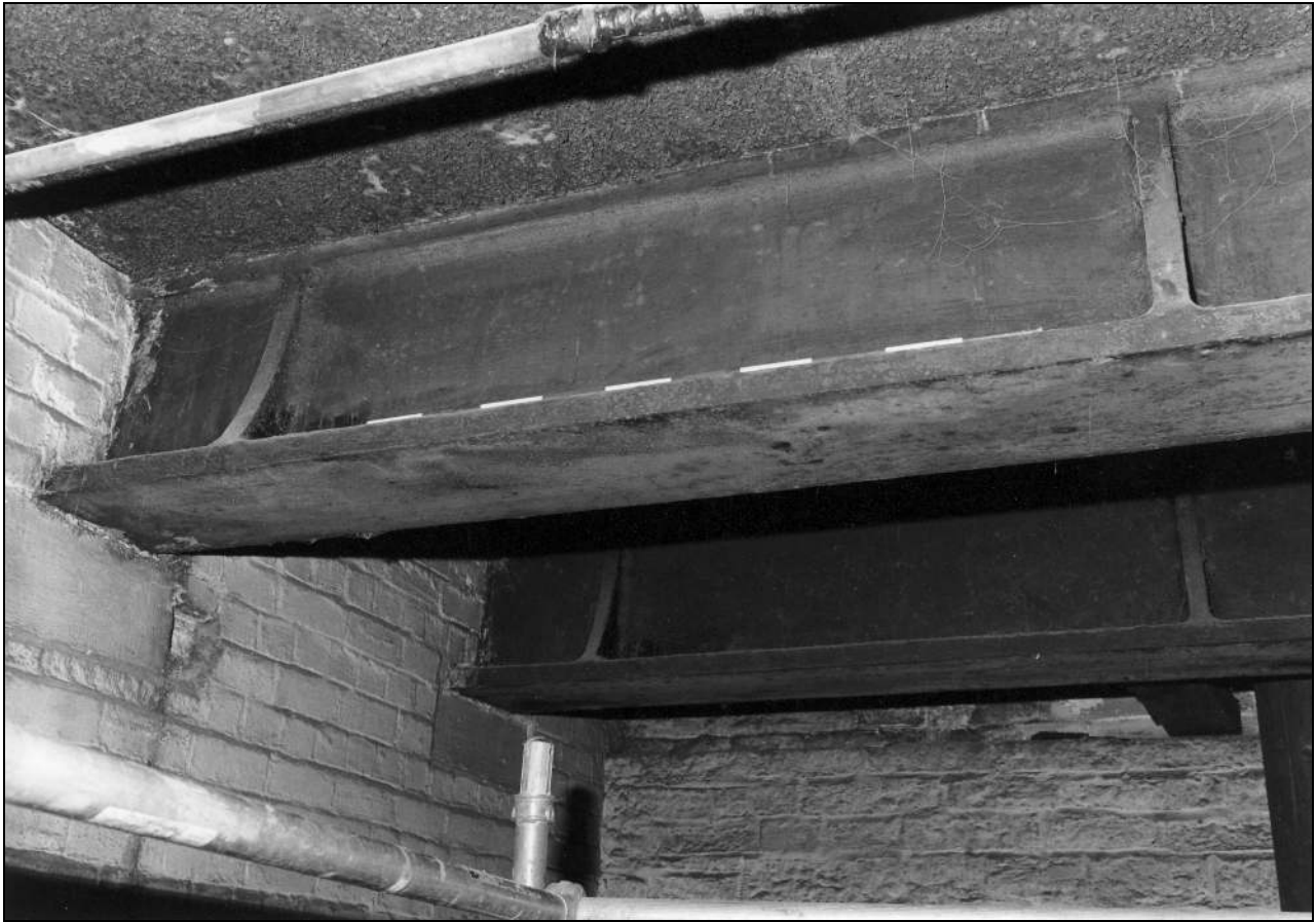
Photo 47: Bay 4: detail of cast iron beam supporting tank (film 8, frame 5)
