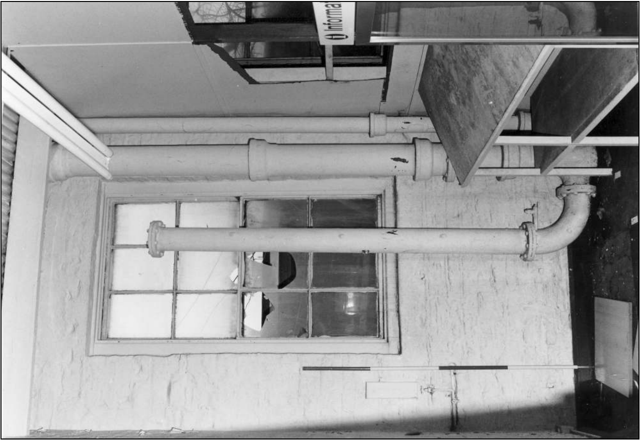
Photo 38: Bay 4: pipes in west side (overflow and later feed, nos 1, 2 & 3) (film 3, frame 2)
