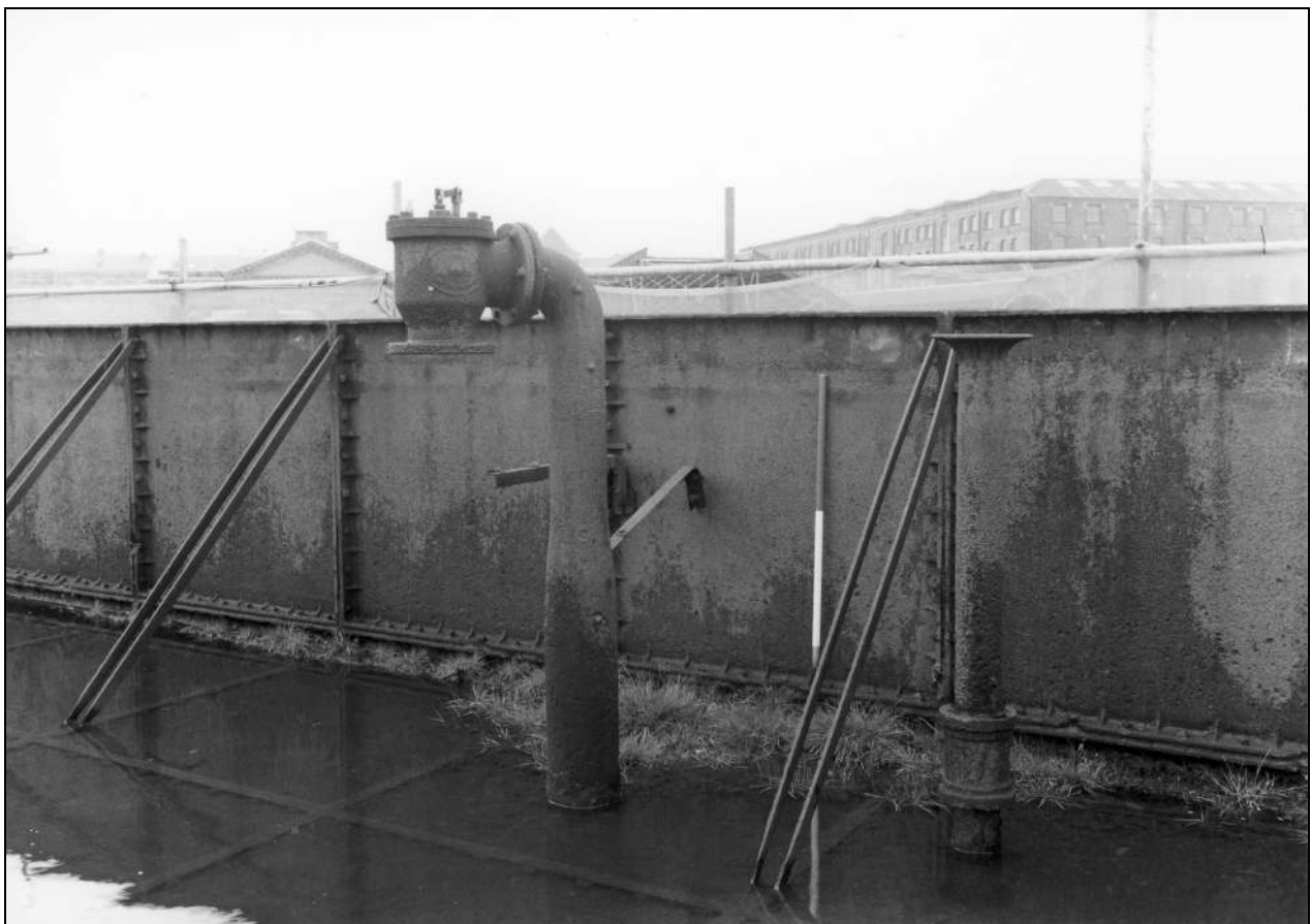
Photo 64: Later feed, and overflow pipes, within tank, from the north-east (film 6, frame 9)
