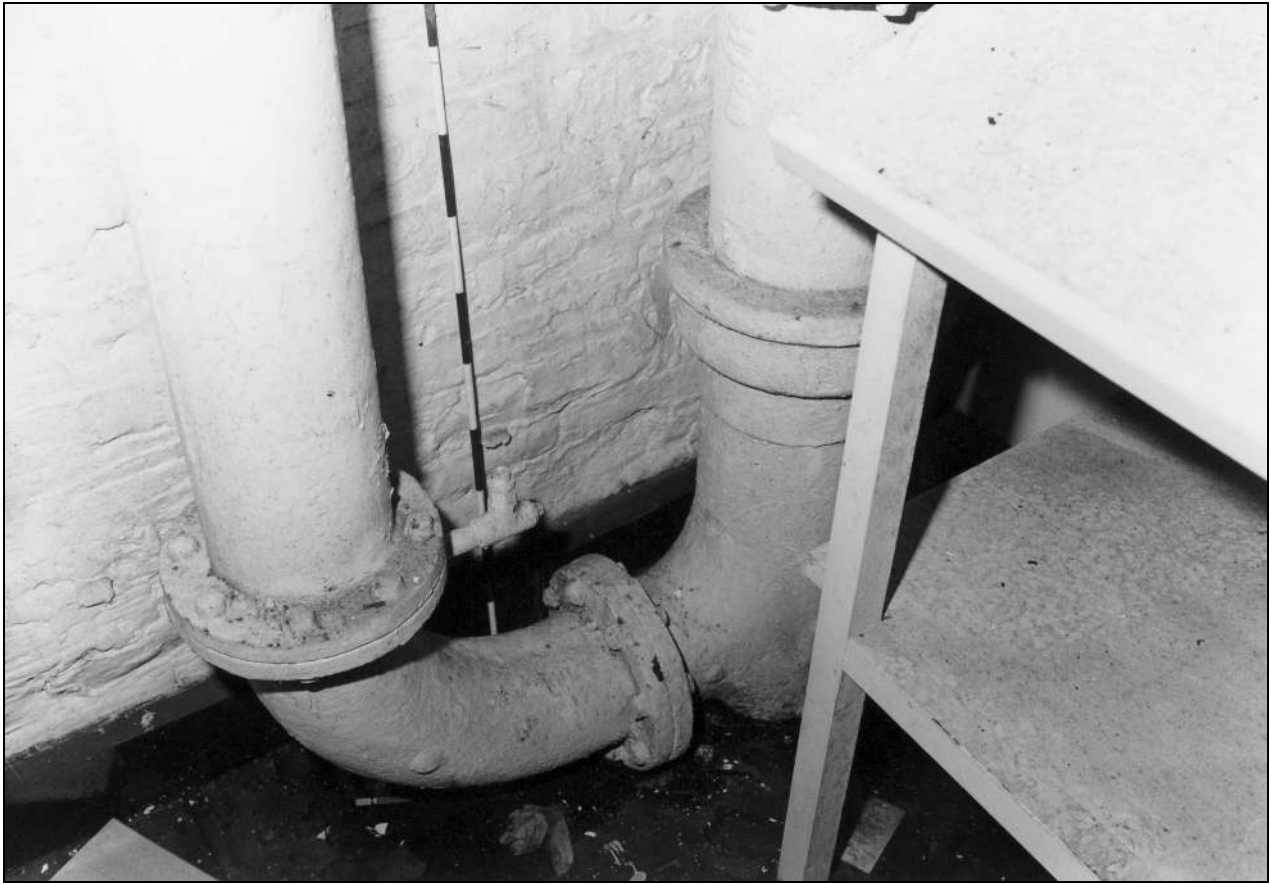
Photo 43: Bay 4: later feed pipe, with junction and drain cock (film 3, frame 9)
