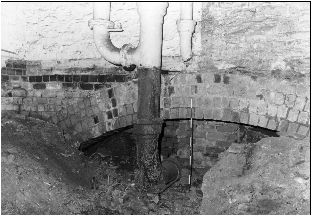
Photo 42: Bay 4: pipes in west side, below ground floor level (overflow and later feed, nos 1 & 2) (film 5, frame 3)
