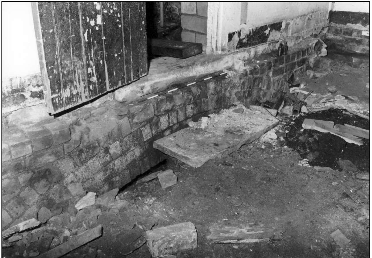
Photo 32: Bay 3: arch to west side of basement, from the south-west (film 5, frame 7)
