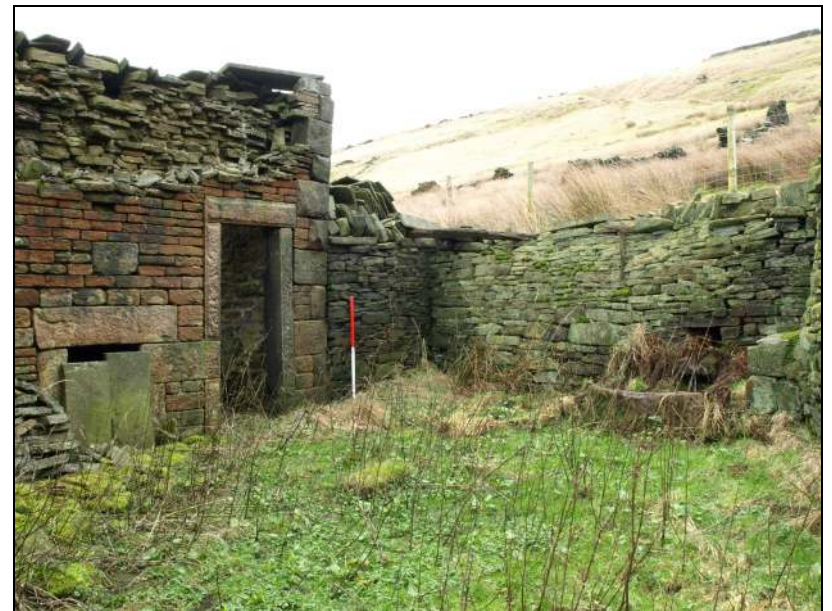
Photo 48: Pig sty, earth closet and water trough with spring
