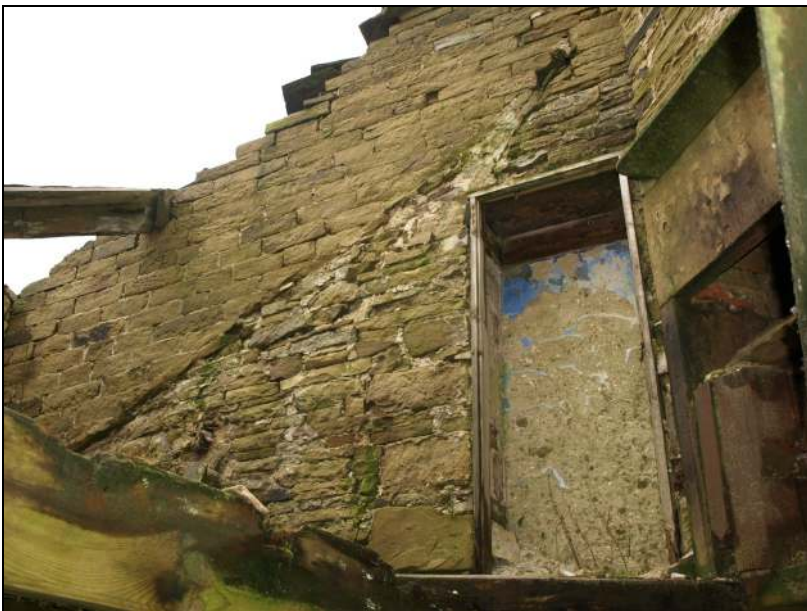
Photo 35: First floor in cottage, showing line of flue and blocked doorway in cross wall, from the south-west
