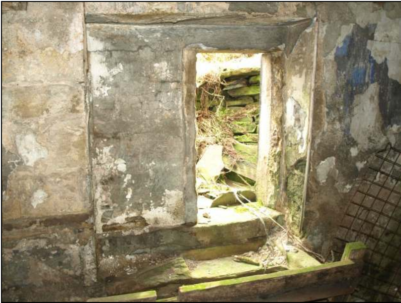
Photo 34: Remains of sink by rear window in scullery of cottage
