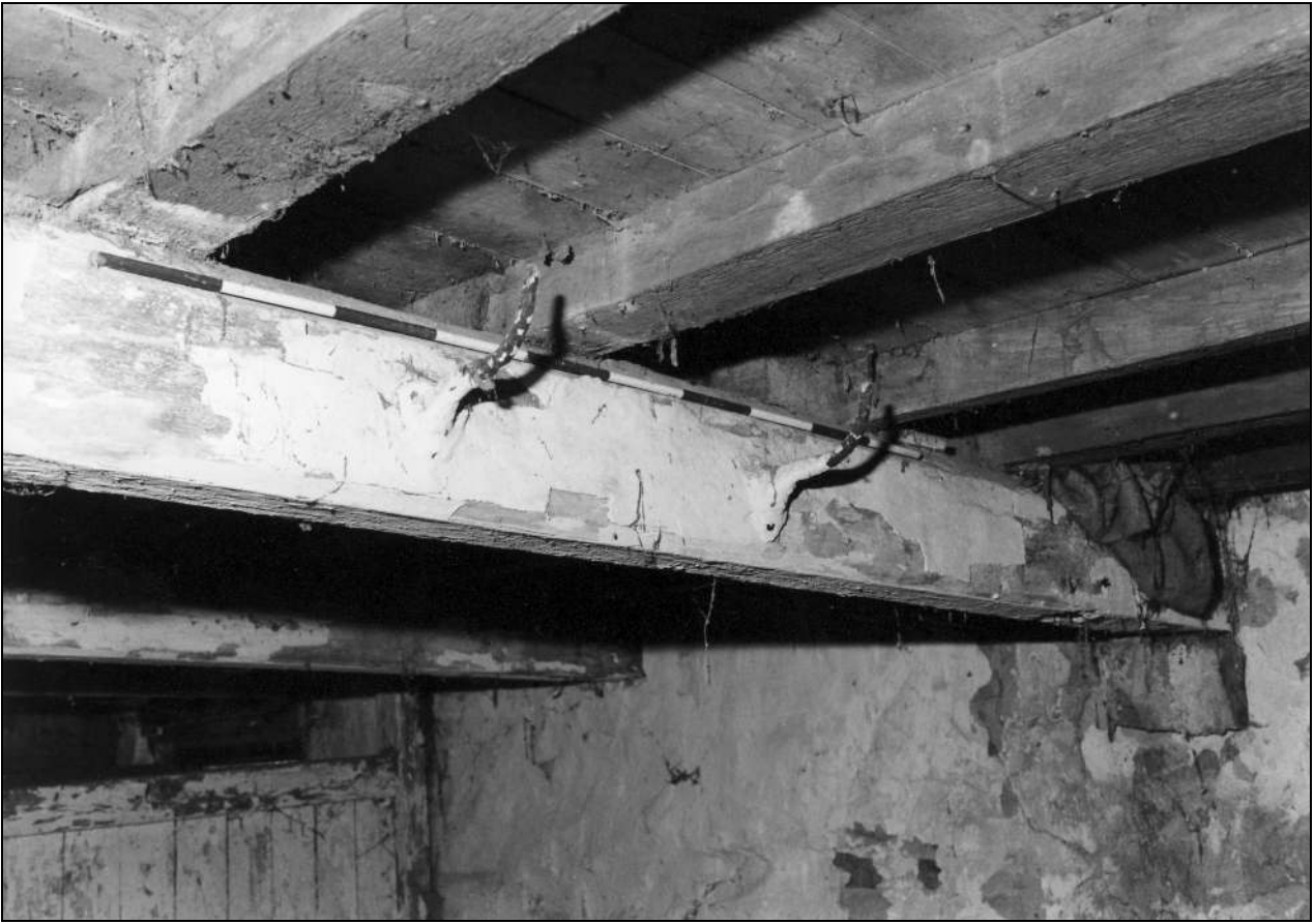
Photo 14: Ground floor: harness pegs fastened to beam by horse/pony stalls, from the north-west
