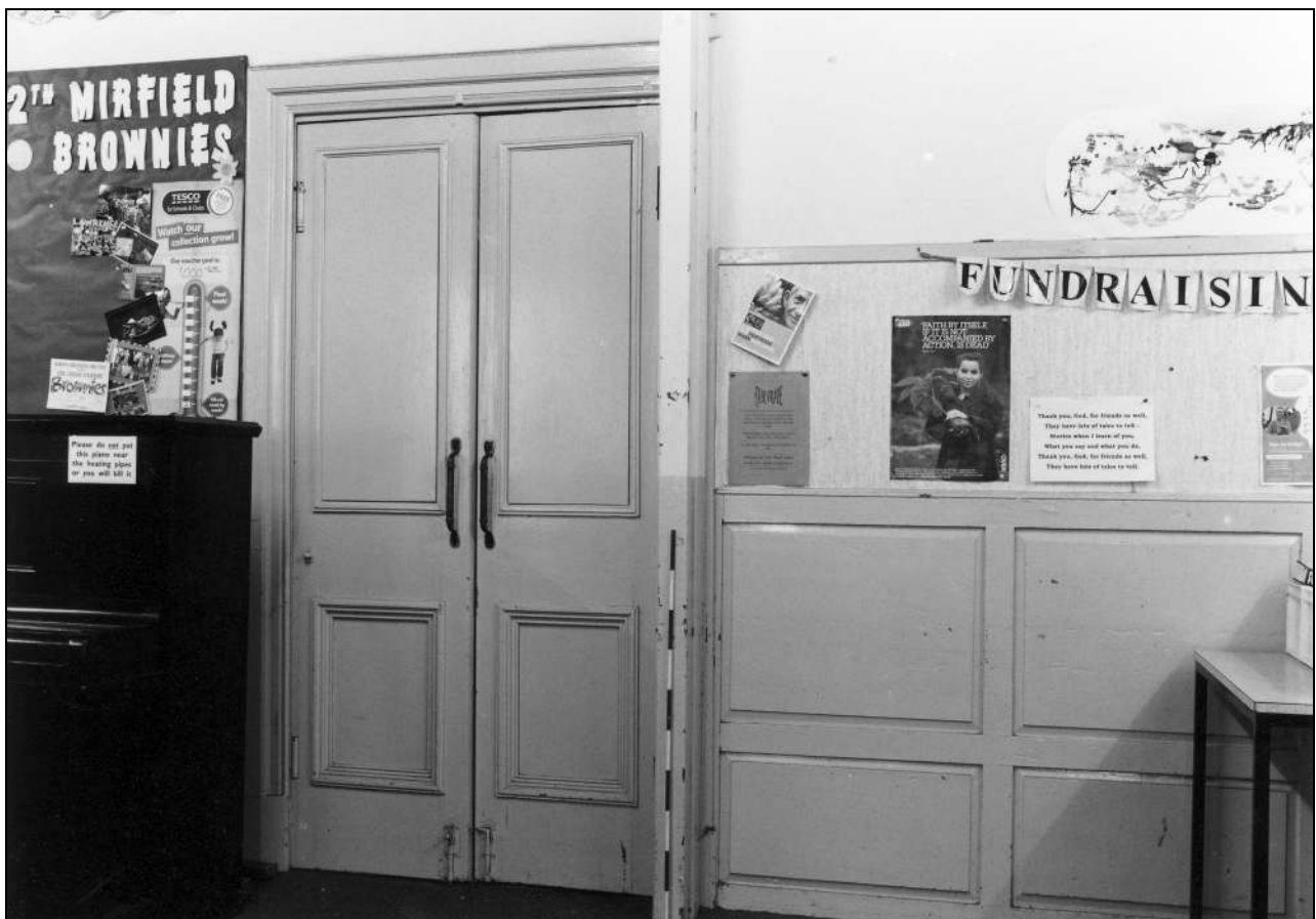
Photo 89: Original doorway to lecture room in church basement, from the west (film 8, frame 7)
