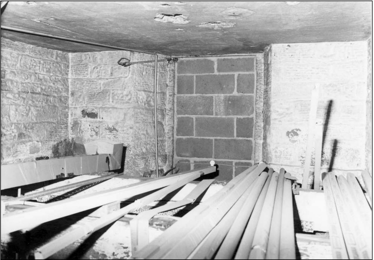
Photo 74: Blocked window, west side of church boiler room (film 7, frame 4)
