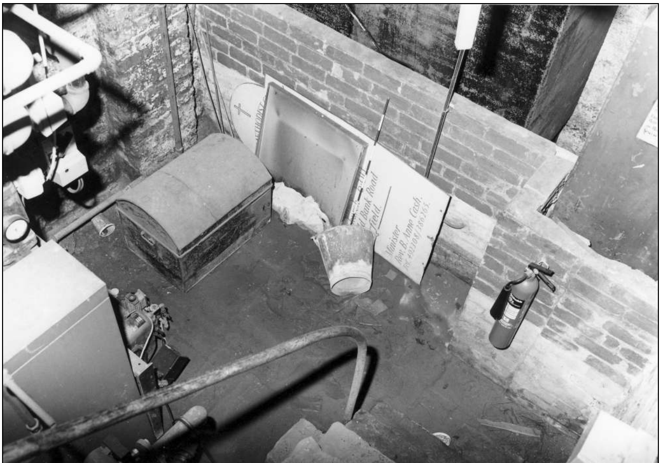
Photo 75: Boiler room in church, from the north-east (film 7, frame 5)
