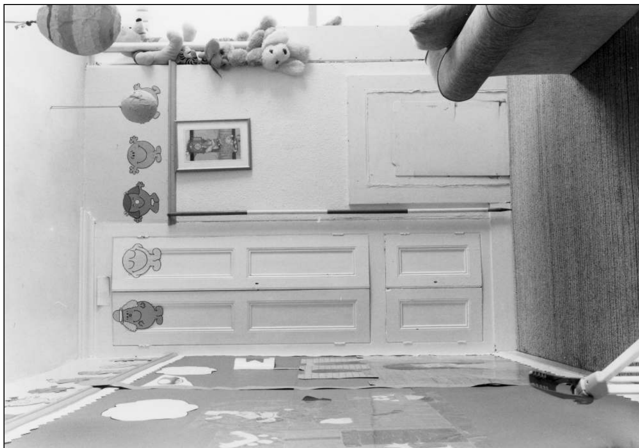
Photo 131: Cupboard and blocked fireplace in south room below Sunday school gallery, from the west (film 4, frame 3)
