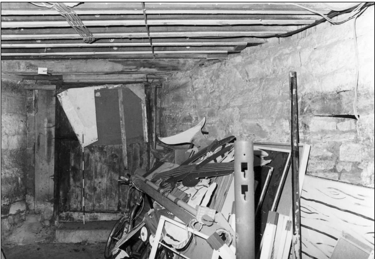
Photo 93: Store in north-west corner of church basement, from the east (film 8, frame 2)
