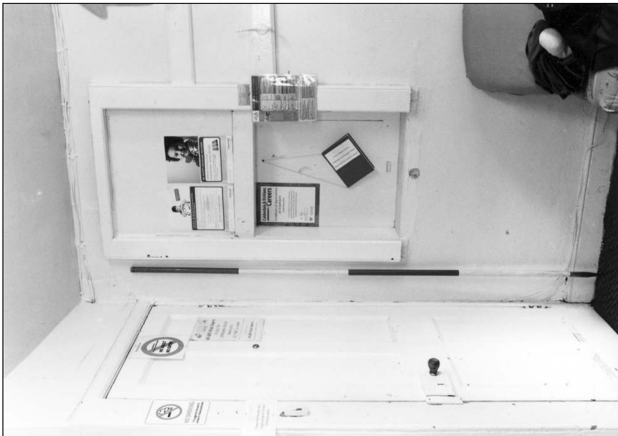
Photo 132: Hatch in north room below Sunday school gallery, from the south (film 4, frame 16)
