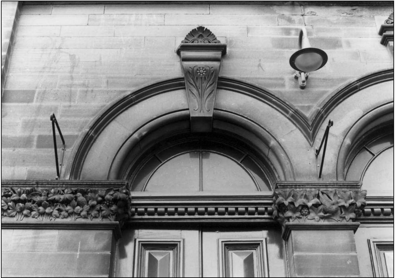
Photo 8: Detail of fanlight, key-stone and impost band over front entrance (film 9, frame 16)
