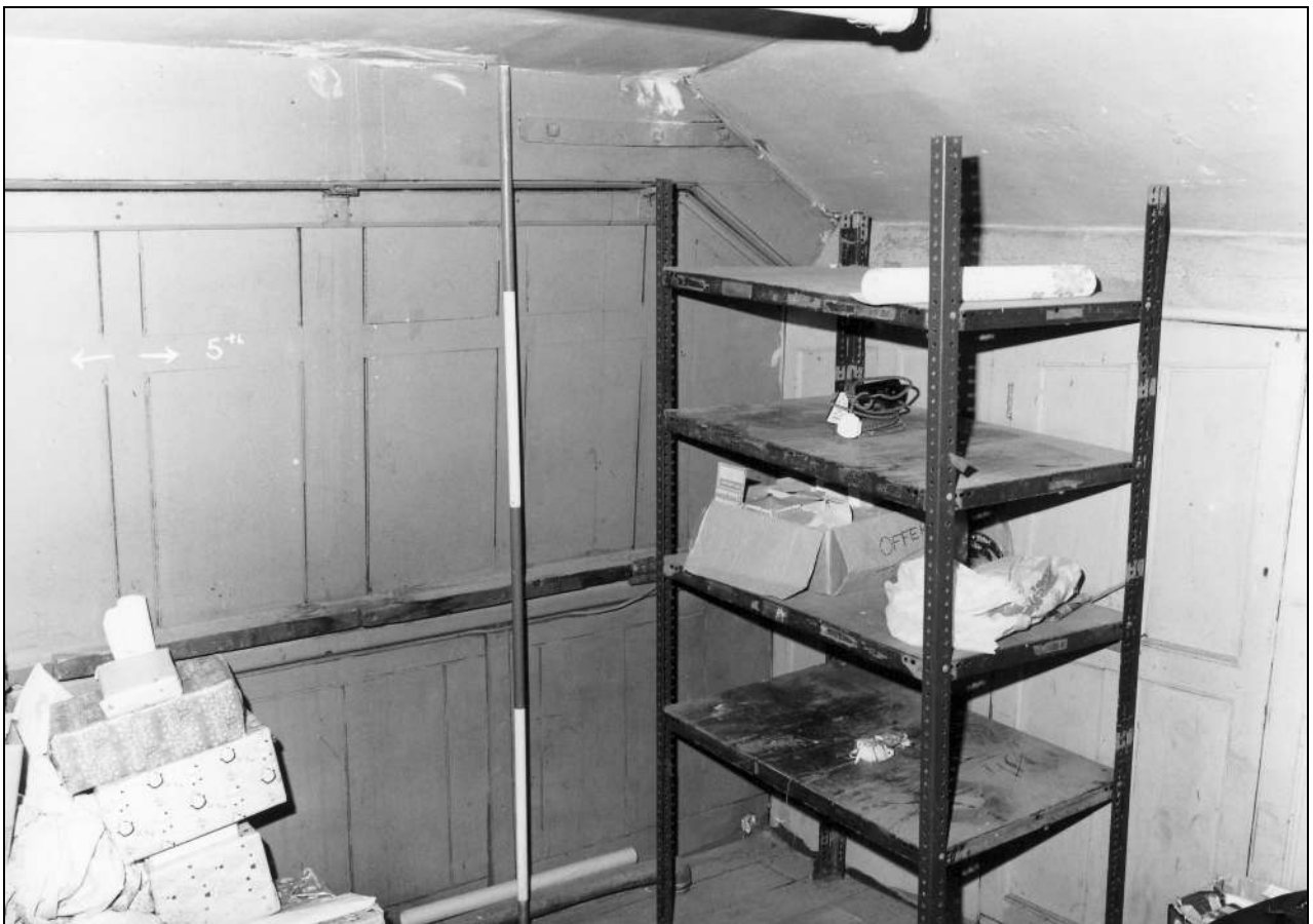
Photo 136: Sunday school gallery with panelled parapet and shutters over, from the south-east (film 5, frame 1)
