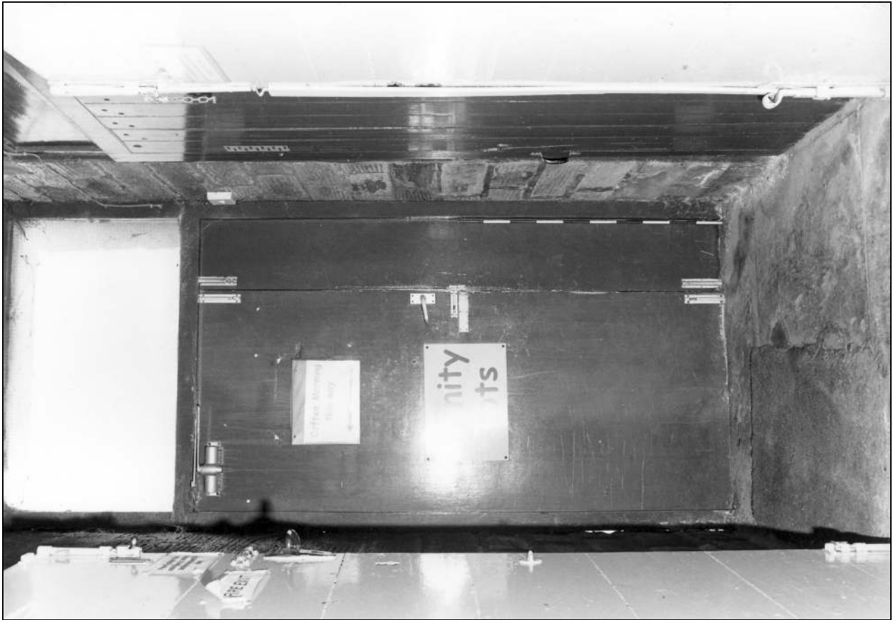
Photo 73: New outer basement door and entrance to wood store (right) (film 7, frame 6)
