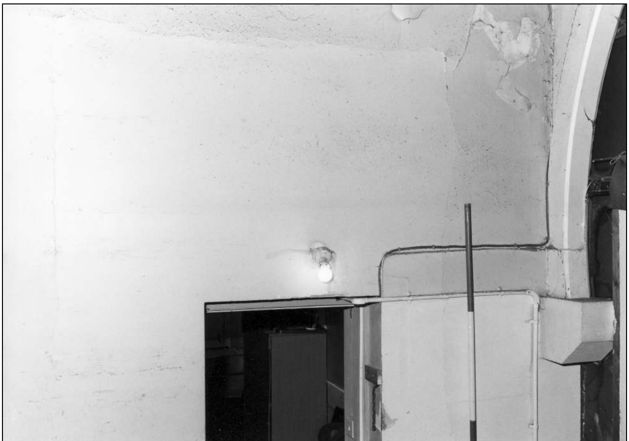
Photo 144: Window in north side of Sunday school, blocked for modern link to church (film 5, frame 10)
