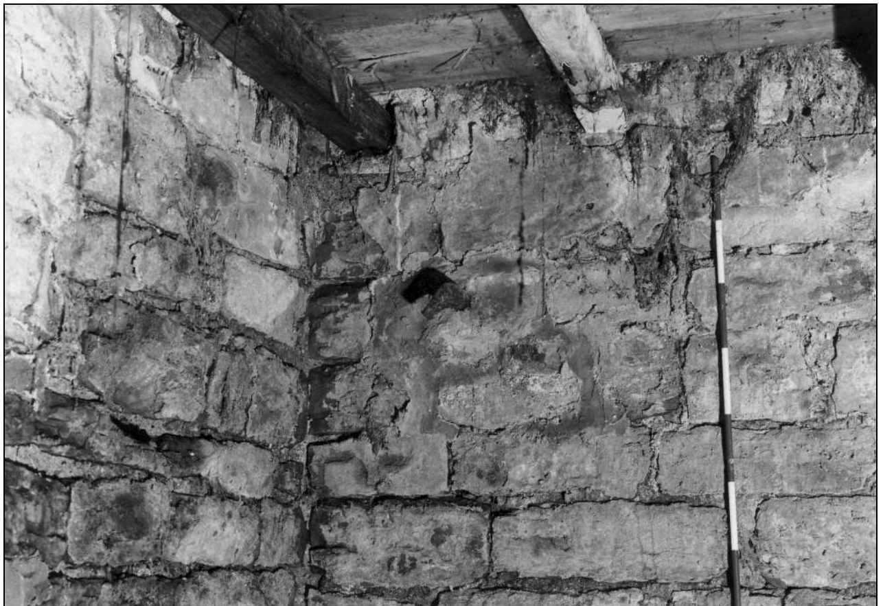
Photo 25: Building 1a: small pipe projecting into north end of ground floor (film 3, frame 10)
