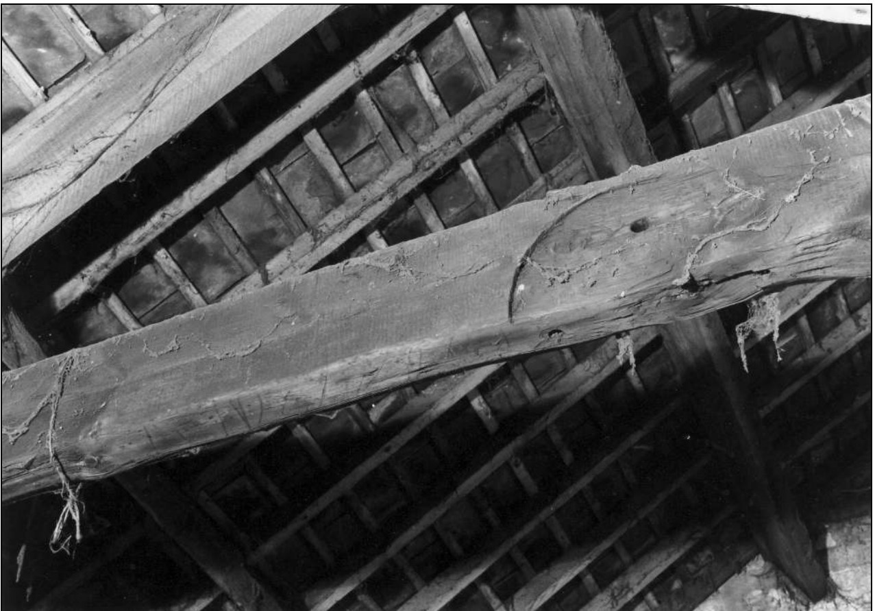
Photo 44: Building 1b: possible location of former line shaft, from the south-east (film 4, frame 8)
