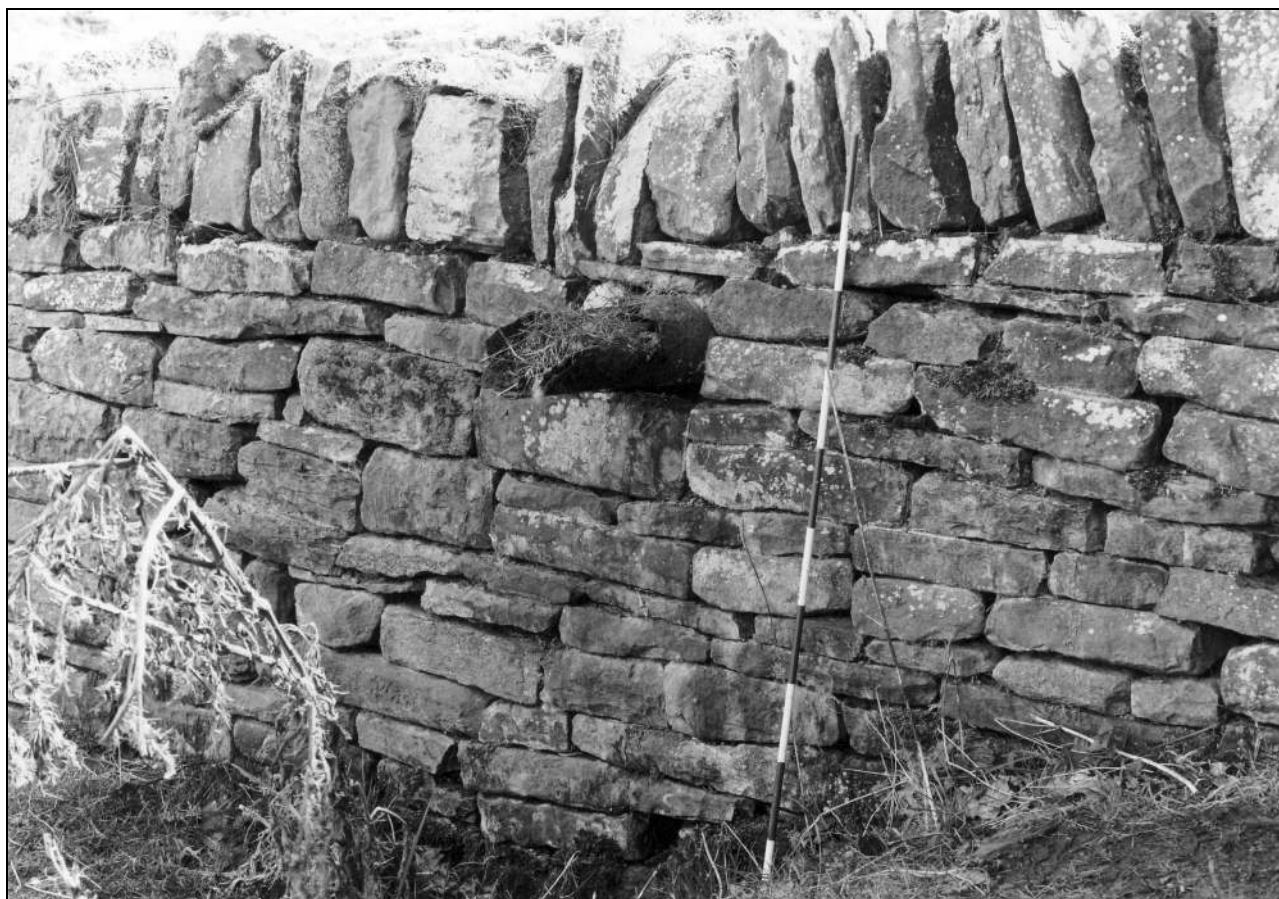
Photo 60: Cast iron water pipe emerging from south retaining wall to east of building 1b, from the north (film 4, frame 17)
