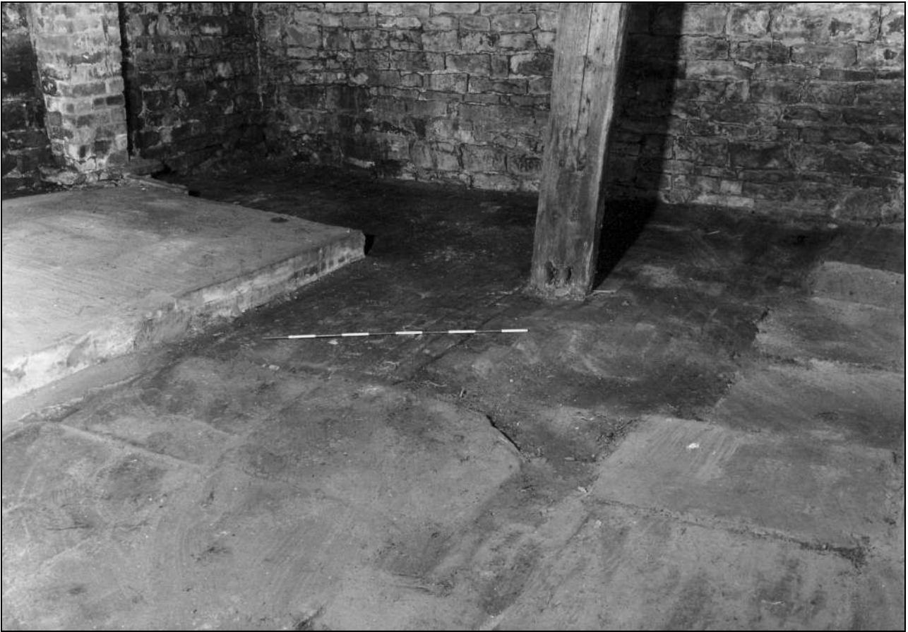
Photo 24: Building 1a: detail of floor surfaces in ground floor, from the south-east (film 3, frame 14)
