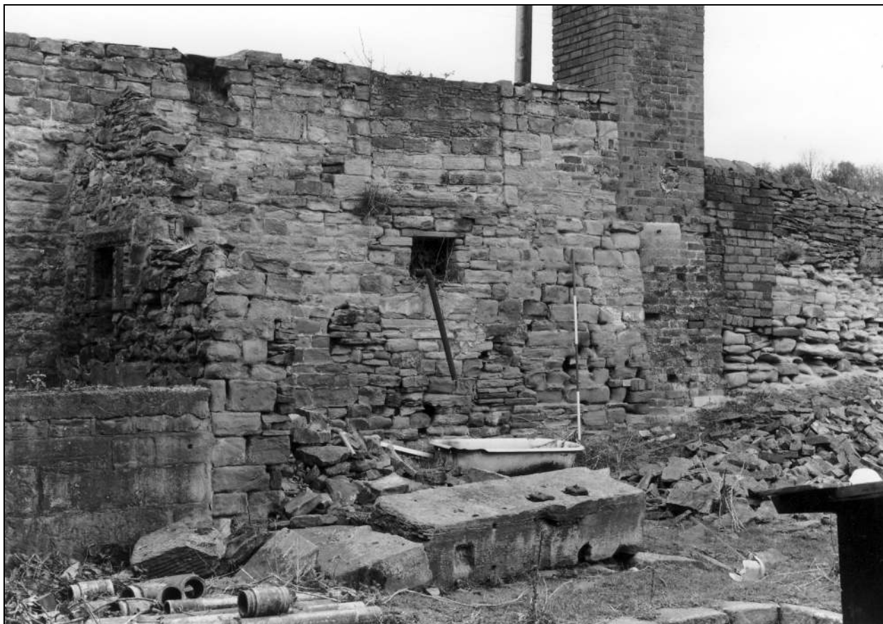
Photo 56: Remains of building (engine house?) at foot of chimney, from the south-west (film 1, frame 18)
