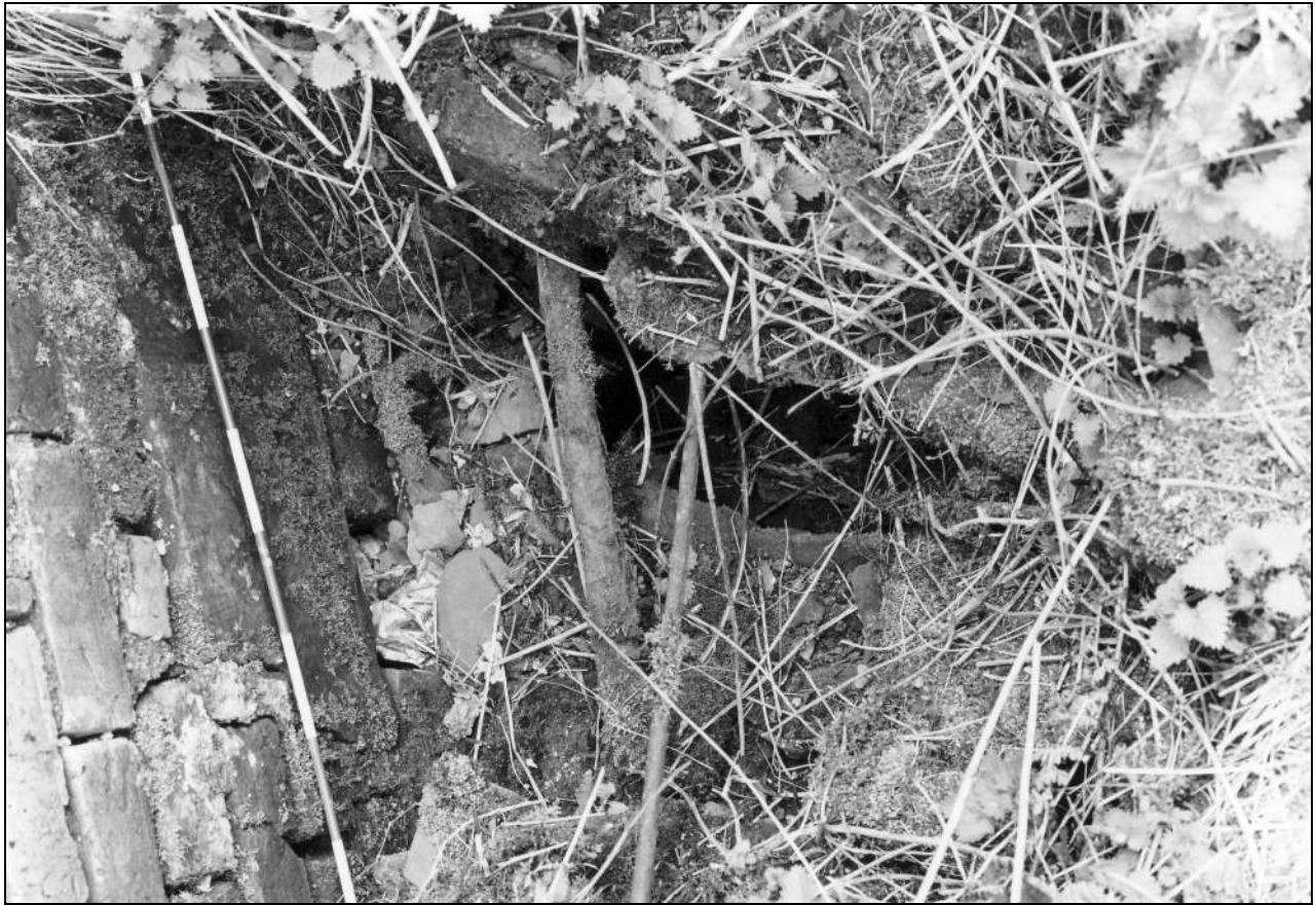
Photo 37: Cast iron water pipe running below south end of building 1b, from the west (film 4, frame 18)
