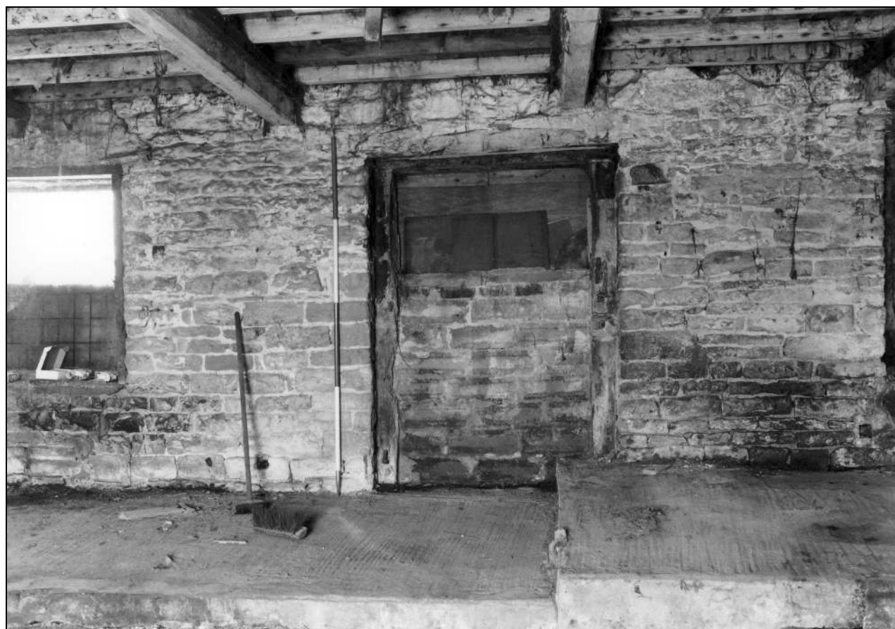
Photo 23: Building 1a: internal view of blocked doorway in west side of ground floor (film 3, frame 16)
