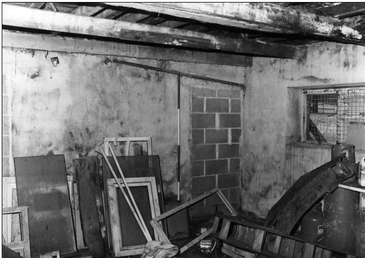
Photo 20: North range: modern room in west end of ground floor (film 3, frame 5)
