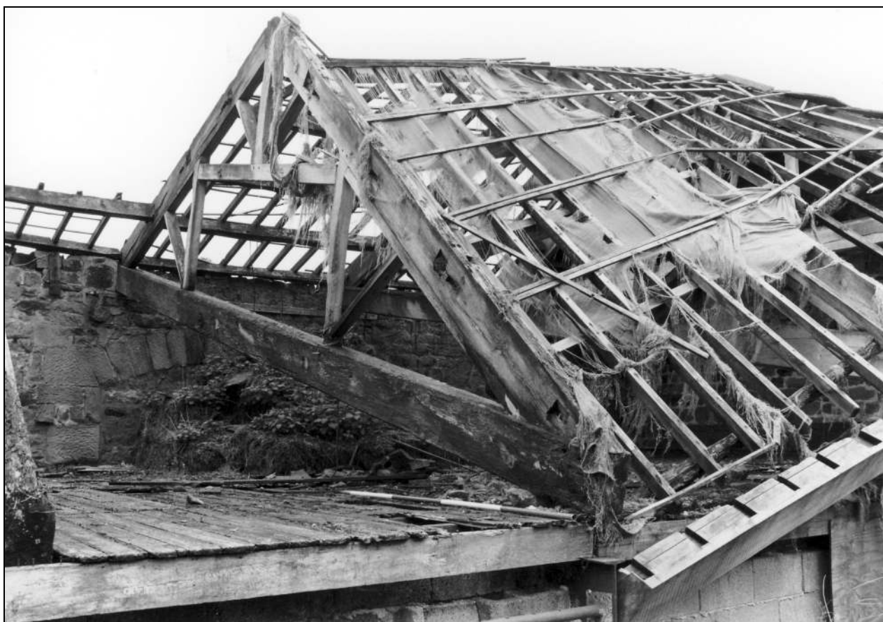
Photo 13: Barn: roof truss to north of central bay, from the north-west (film 2, frame 12)
