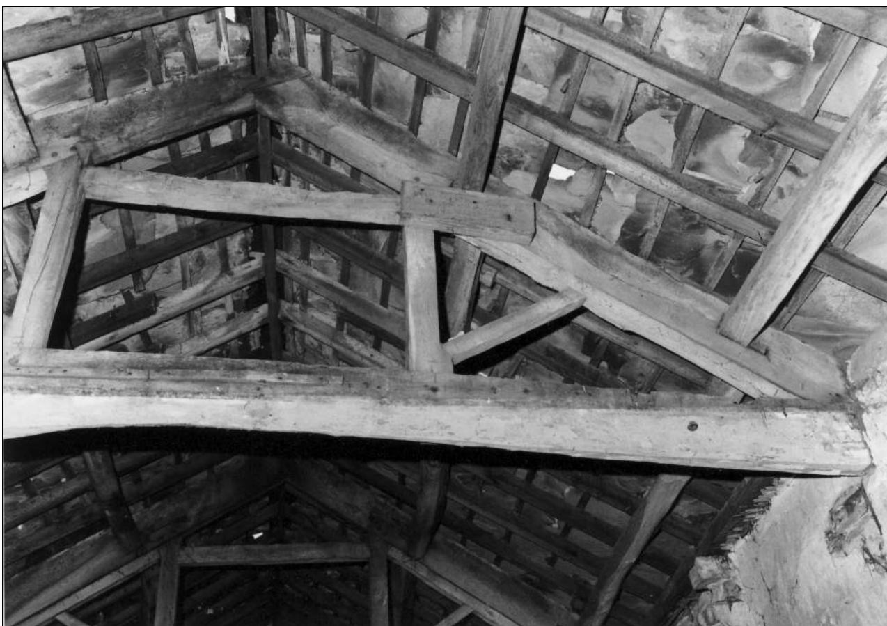
Photo 34: North range: roof truss in east part, from the west (film 3, frame 16)
