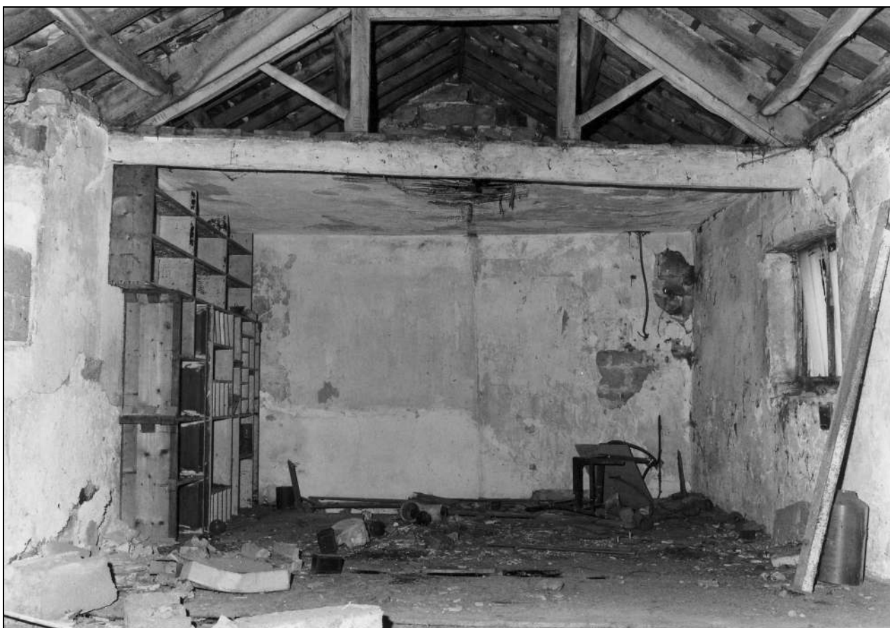
Photo 32: North range: first floor in east part, from the west (film 3, frame 17)
