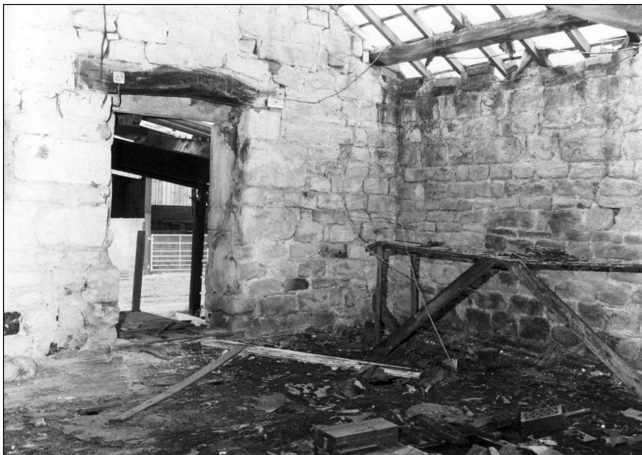
Photo 23: North range: first floor in west part, from the south-east (film 3, frame 9)
