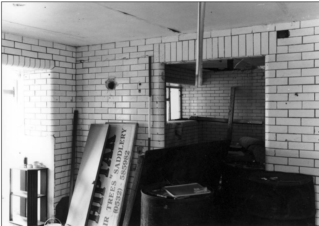
Photo 31: North range: modern room (dairy) in east end of ground floor (film 3, frame 7)
