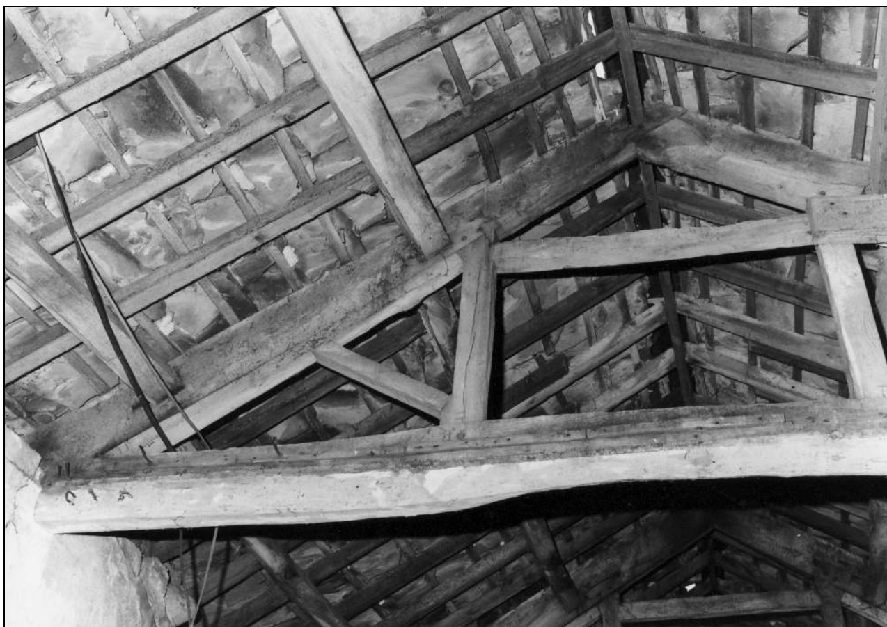
Photo 33: North range: roof truss in east part, from the west (film 3, frame 15)
