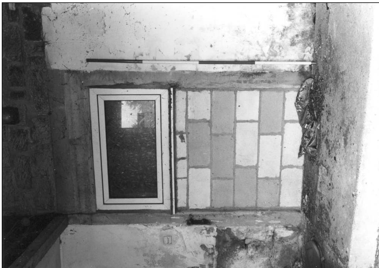
Photo 27: North range: former doorway (original) in south elevation of east part (film 3, frame 6)
