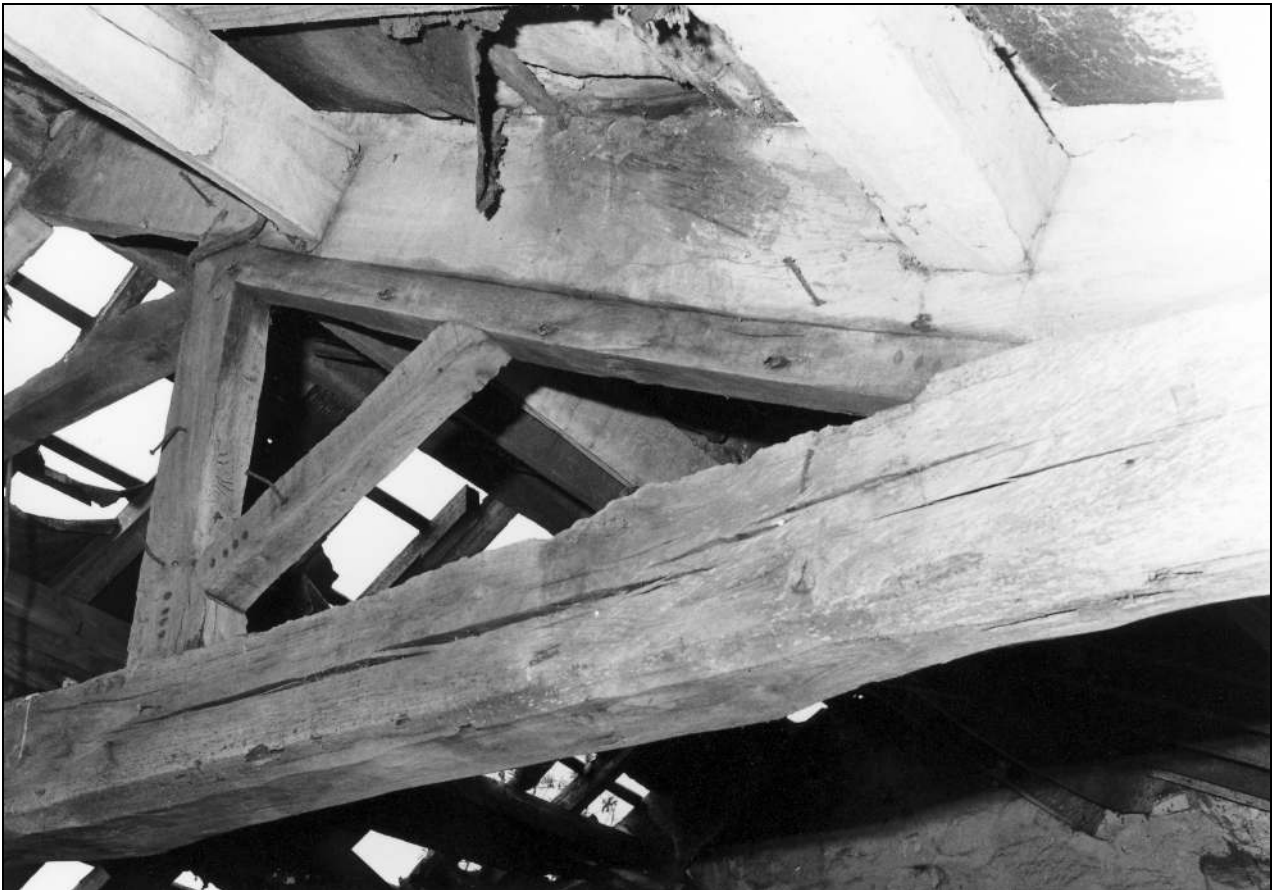
Photo 26: North range: roof truss in west part, from the south-west (film 3, frame 13)
