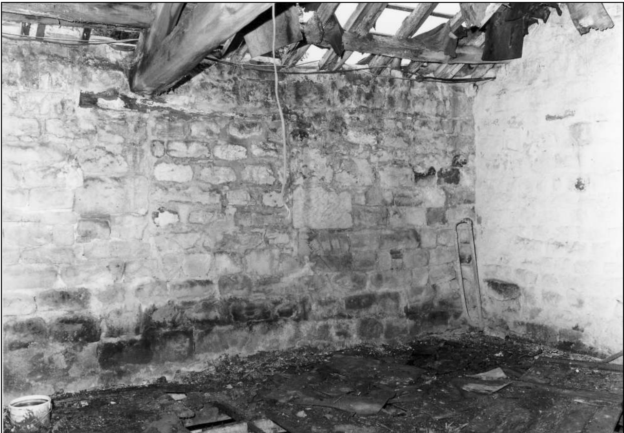
Photo 22: North range: first floor in west part, from the south-west (note blocked opening below tie beam) (film 3, frame 10)
