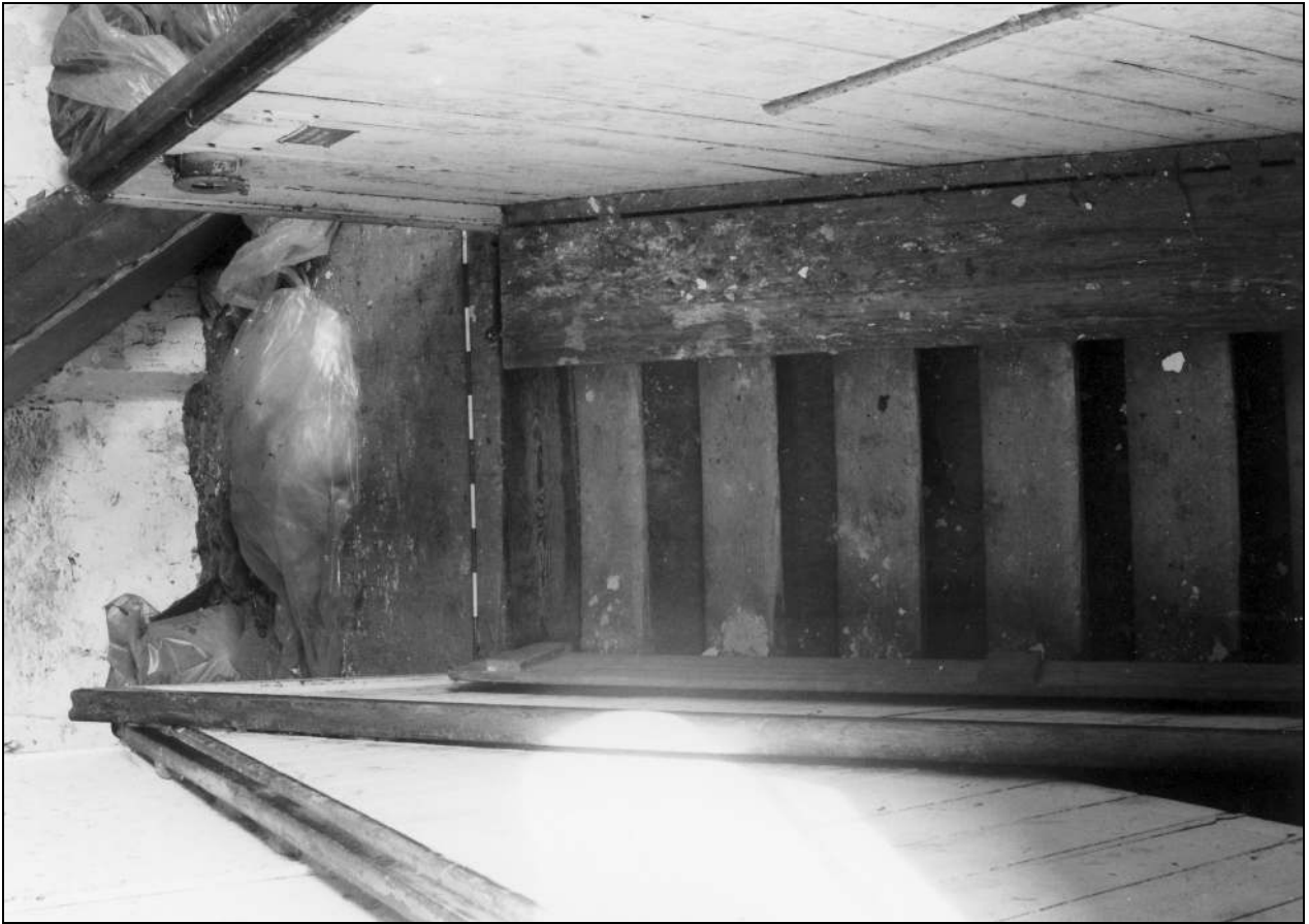
Photo 25: Stairs up to first floor of spinning mill, from the south (film 3, frame 13)
