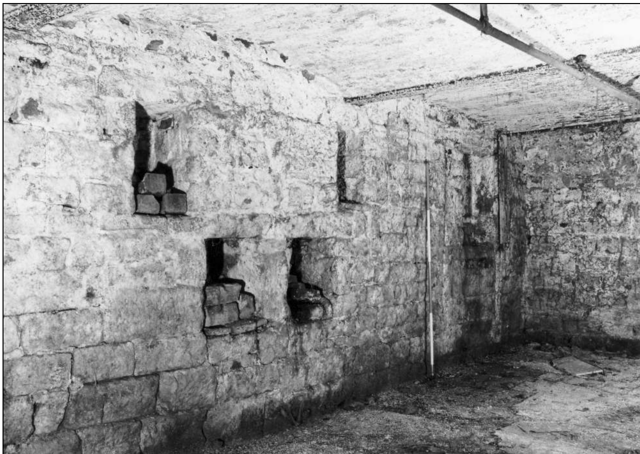
Photo 29: Fireproof room in east end of spinning mill (ground floor), from the north-west (film 7, frame 5)
