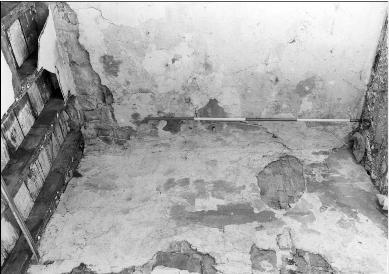
Photo 45: Second floor of spinning mill, from the north-east, showing underside of third floor (film 4, frame 6)
