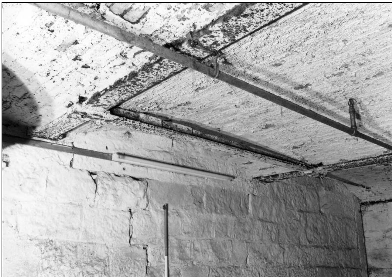
Photo 30: Fireproof room in east end of spinning mill (ground floor): detail of brick jack arches etc (film 7, frame 7)
