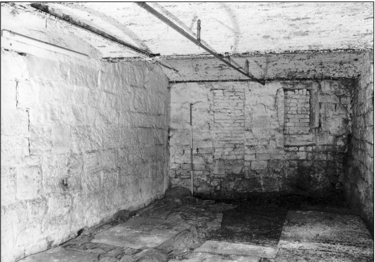
Photo 26: Fireproof room in east end of spinning mill (ground floor), from the south-east (film 7, frame 3)
