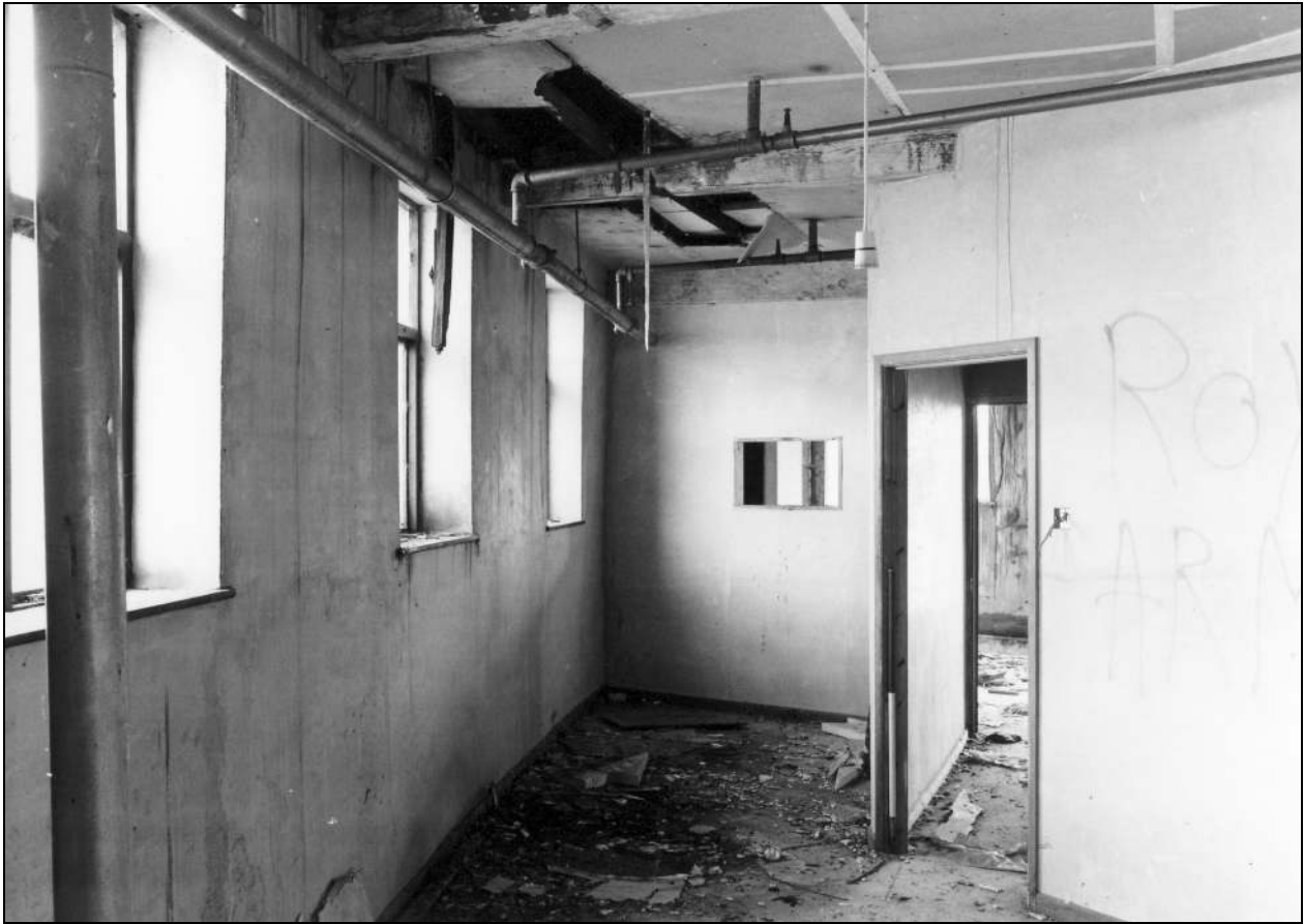
Photo 43: Second floor of spinning mill, from the south-west, showing modern partitions (film 4, frame 7)
