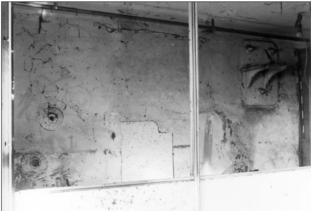
Photo 35: First floor of spinning mill: west wall, showing shaft bracket etc (film 3, frame 11)
