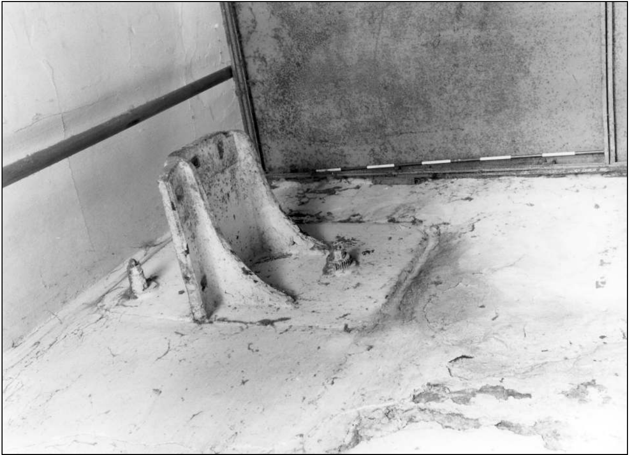
Photo 37: First floor of spinning mill: detail of shaft bracket in west wall (film 3, frame 7)
