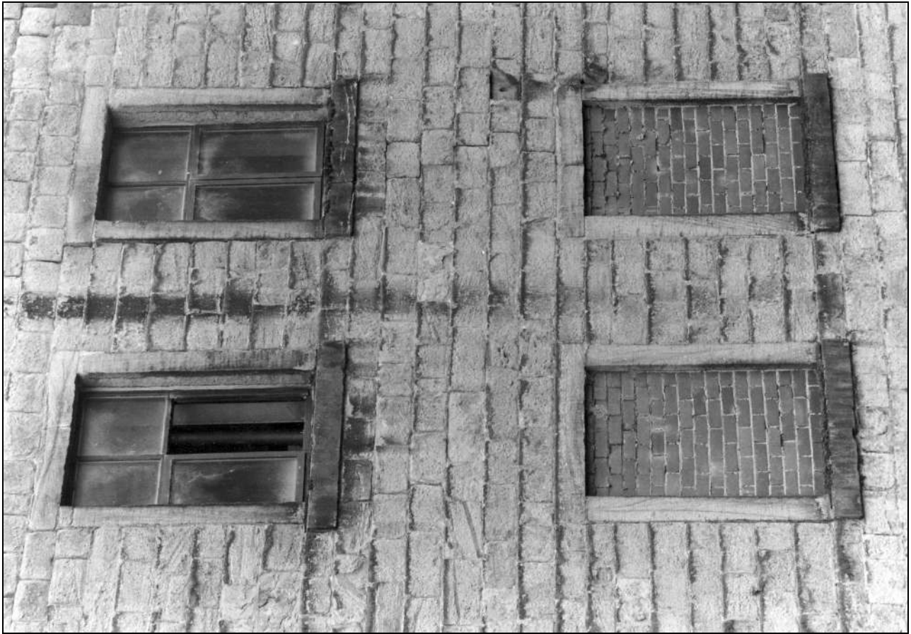
Photo 8: Detail of first and second floor windows in spinning mill, north elevation (film 8, frame 8)
