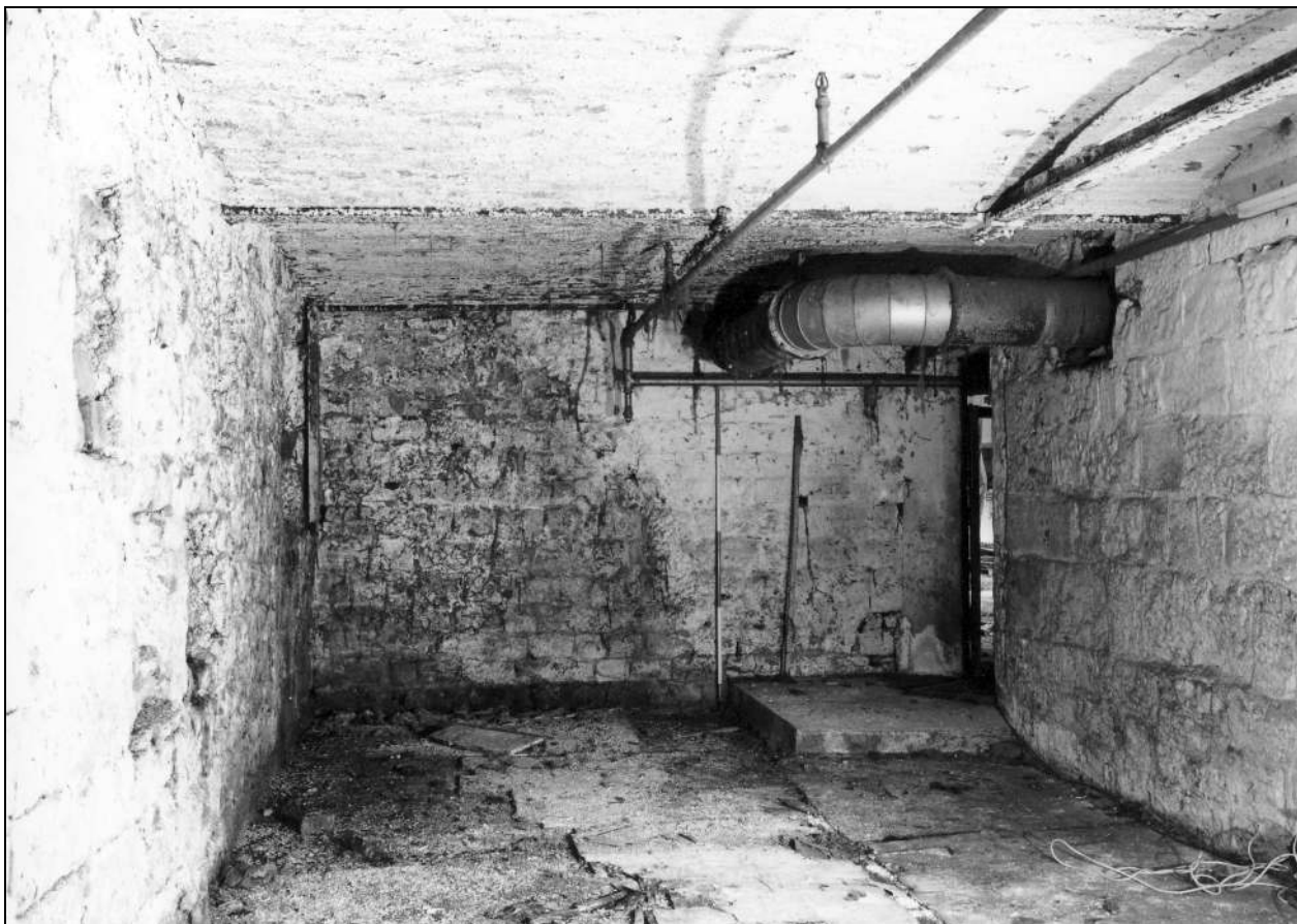
Photo 27: Fireproof room in east end of spinning mill (ground floor), from the north-east (film 7, frame 6)
