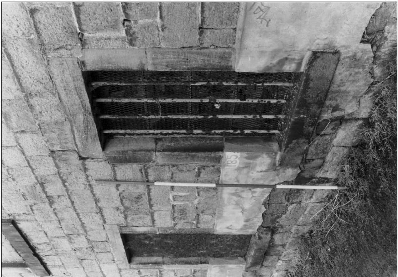
Photo 7: Detail of ground floor windows in spinning mill, north elevation (film 5, frame 10)
