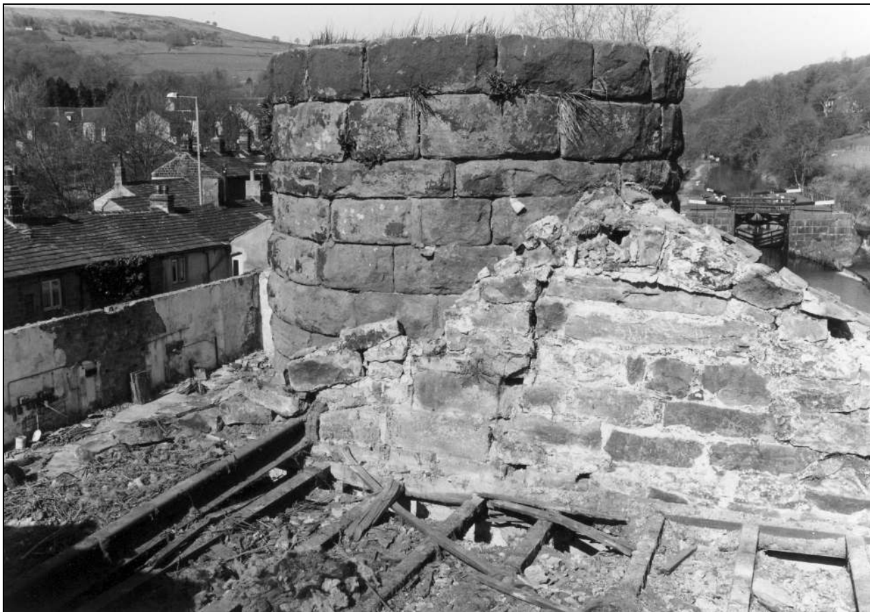
Photo 71: Top of engine house following removal of roof, from the east (film 10, frame 4)
