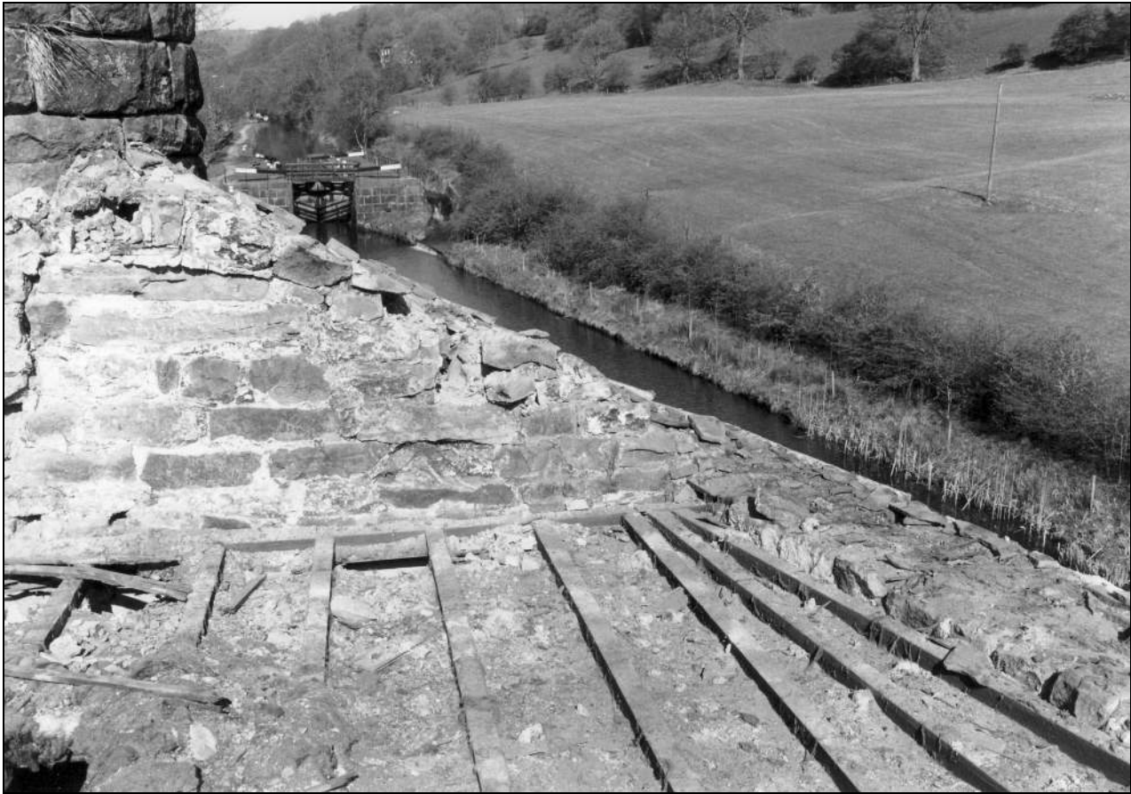
Photo 72: Top of engine house following removal of roof, from the east (film 10, frame 5)
