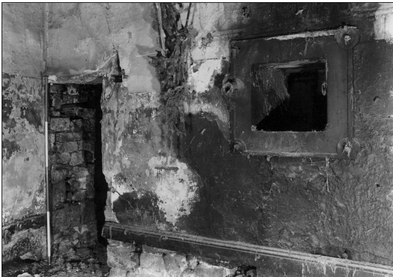
Photo 63: Interior of engine house: north-east corner, showing doorway and wall box for shaft to mill (film 5, frame 12)
