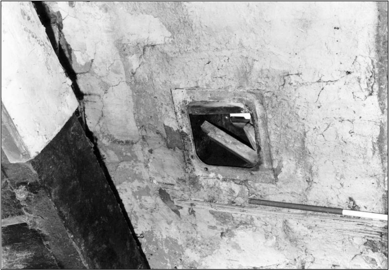
Photo 83: Detail of wall box in south side of boiler house, from the south (film 1, frame 16)
