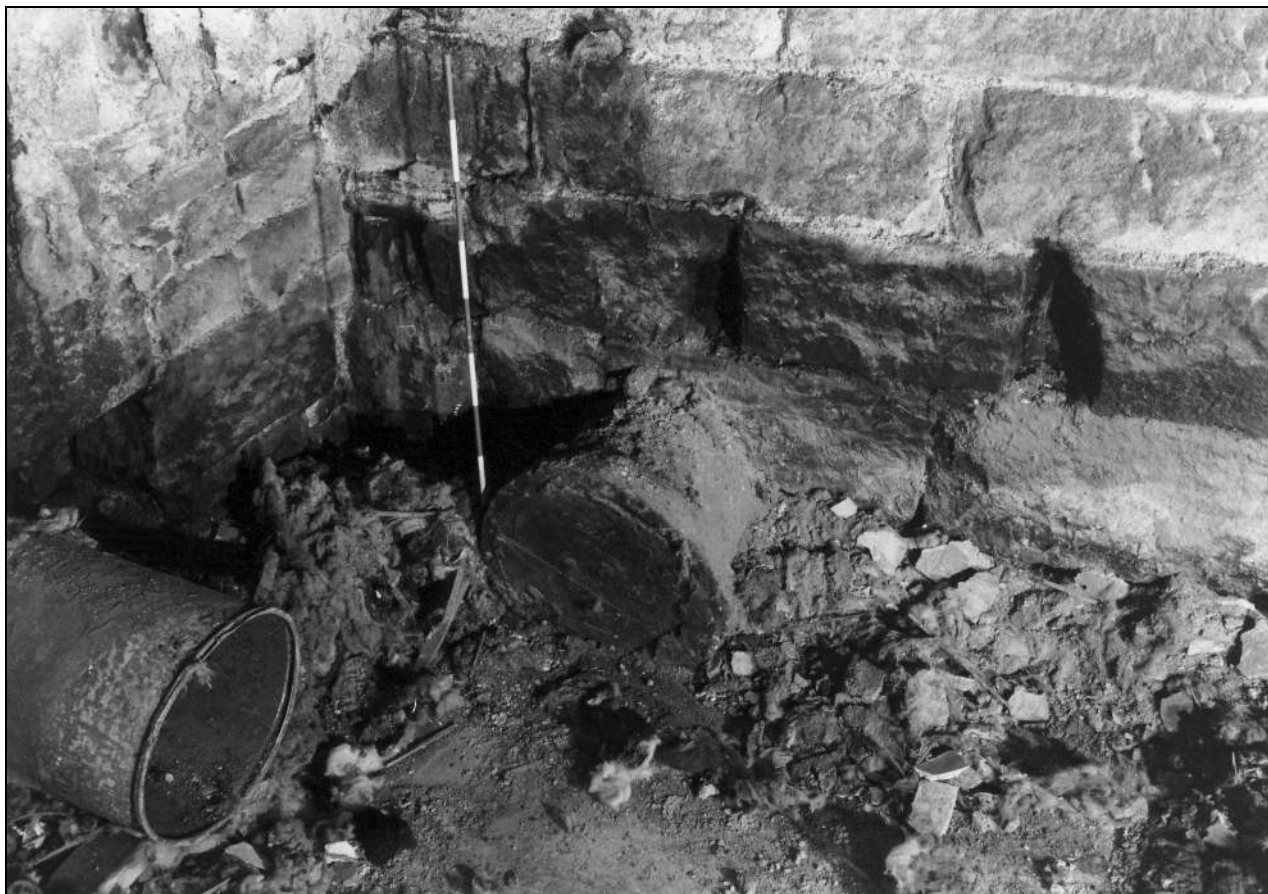
Photo 62: Interior of engine house: south-west corner, showing pipe in line with chimney (film 6, frame 4)
