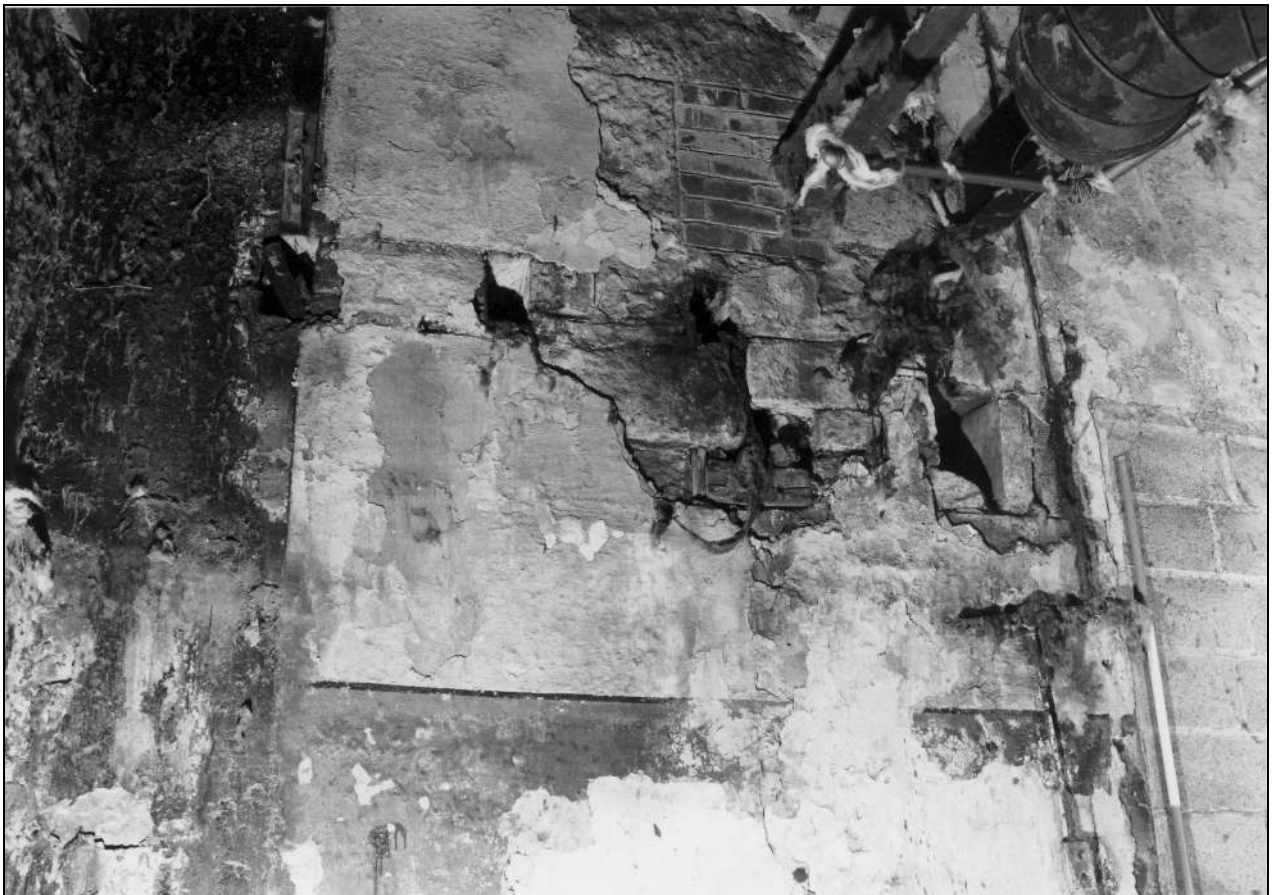
Photo 61: Interior of engine house: west side, showing position of former gallery (film 6, frame 6)
