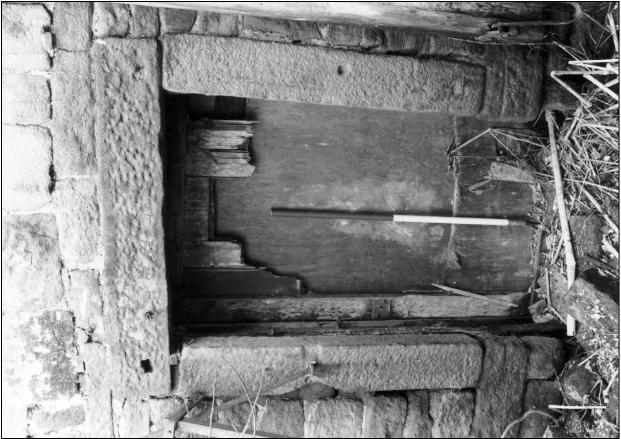
Photo 81: North side of doorway from boiler house to weaving shed (film 4, frame 15)
