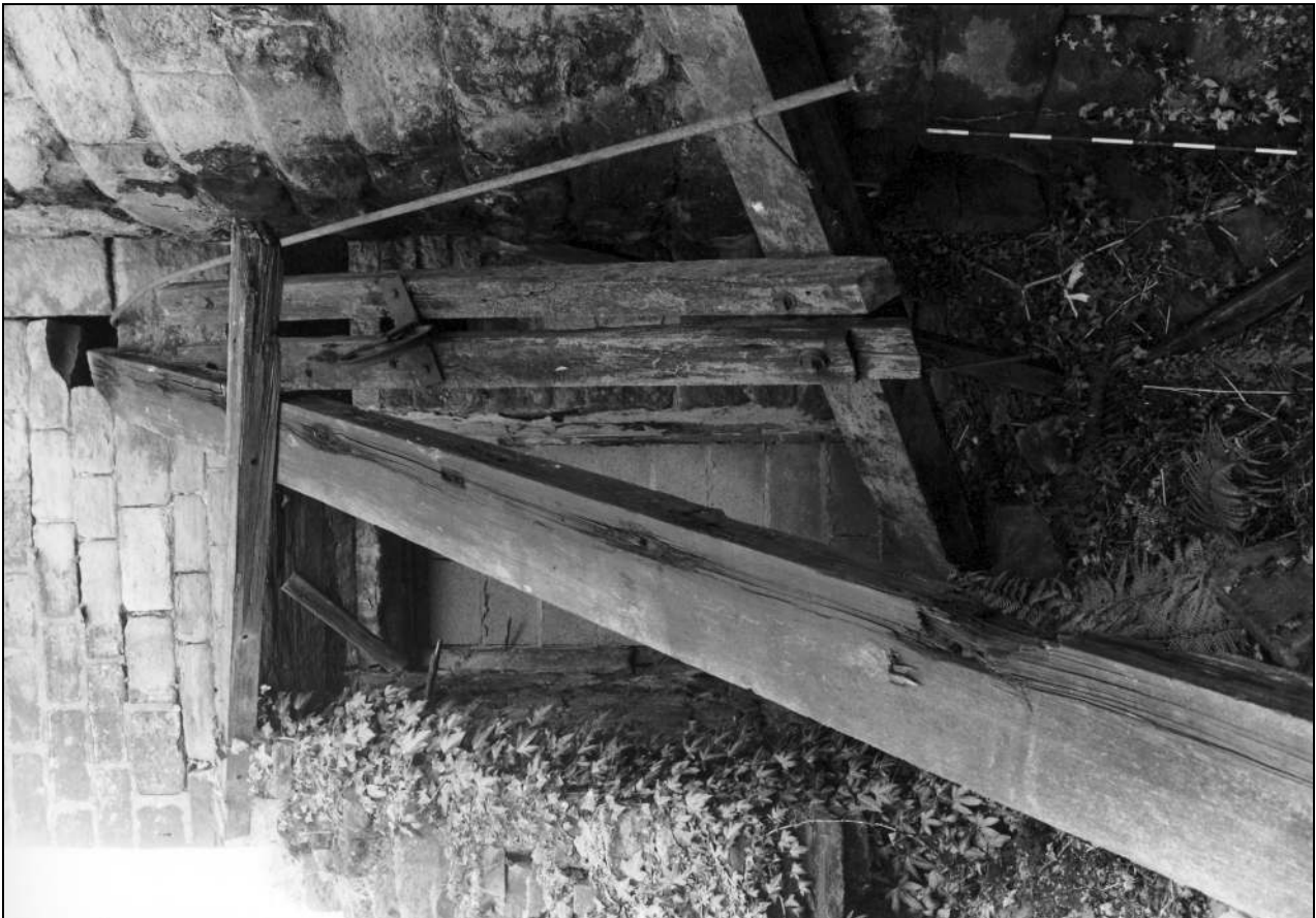
Photo 82: Remains of hoisting timbers in east end of boiler house (film 5, frame 5)
