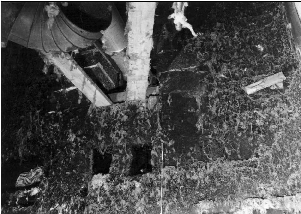
Photo 52: Interior of engine house: south side, showing flywheel bearing and openings for fastening rods (film 6, frame 1)
