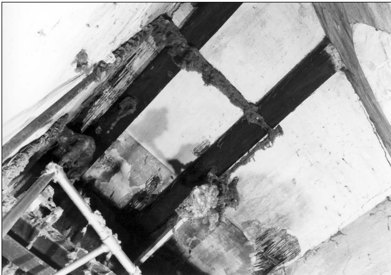
Photo 70: Interior of engine house: view of beams in ceiling, from the north-east corner (film 6, frame 12)
