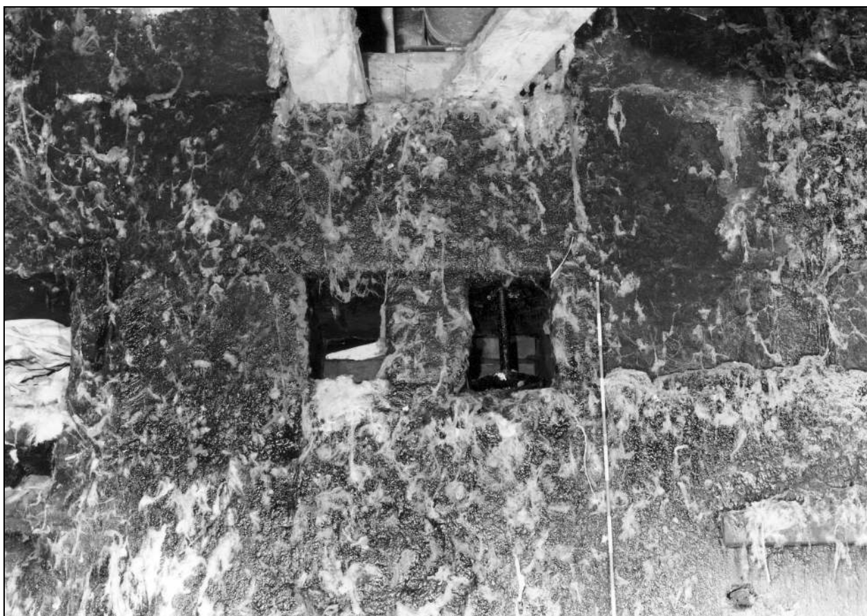
Photo 53: Interior of engine house: south side, showing openings for fastening rods (film 5, frame 18)
