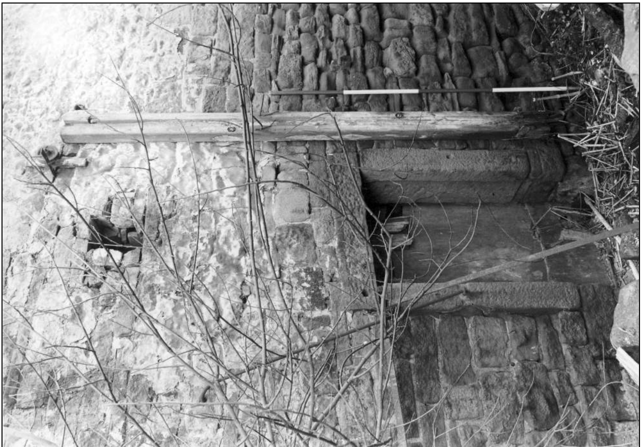
Photo 80: North side of doorway from boiler house to weaving shed (film 5, frame 1)
