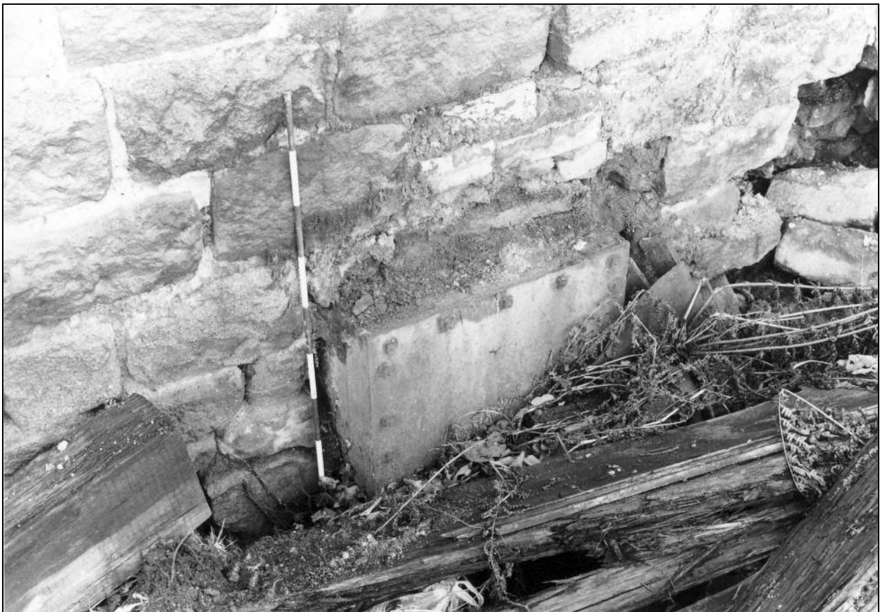
Photo 85: Detail of capped box in south side of boiler house, from the north (film 4, frame 17)
