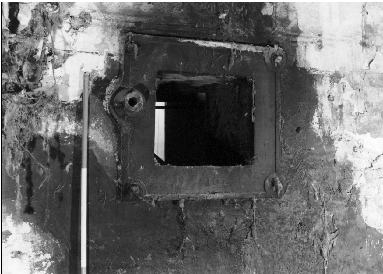
Photo 64: Interior of engine house: detail of wall box for shaft to mill (film 5, frame 13)
