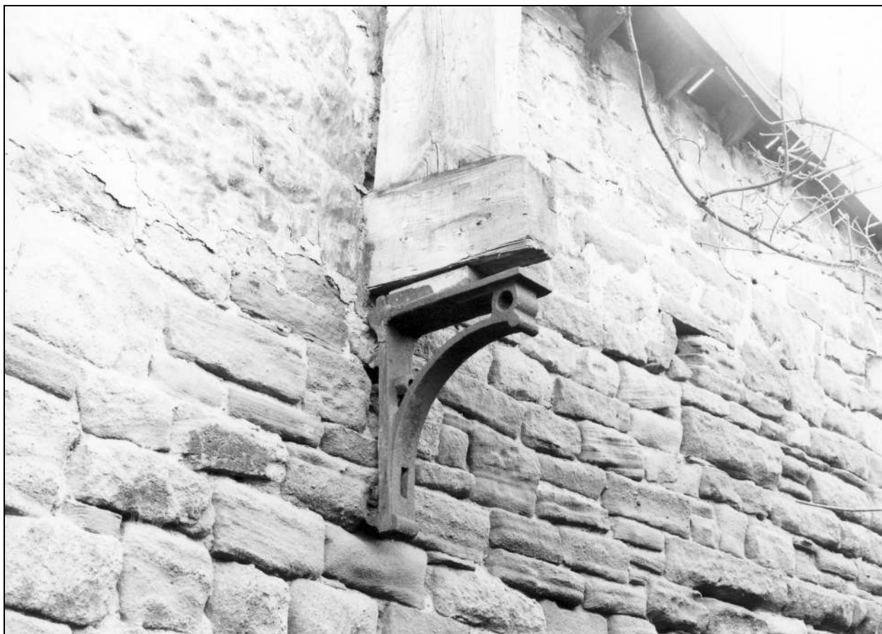
Photo 89: Detail of iron bracket to roof truss over boiler house, from the north-east (film 4, frame 16)
