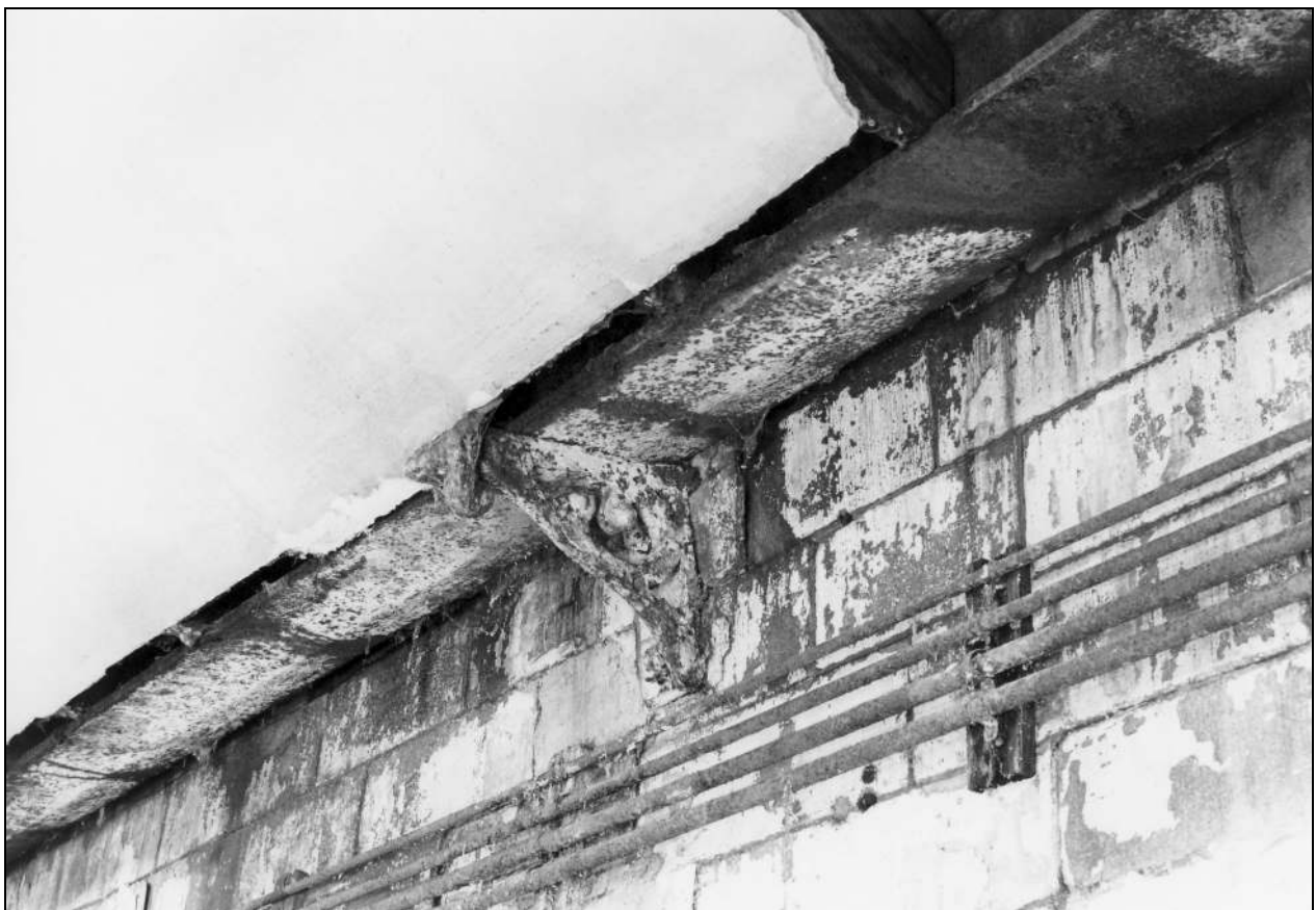
Photo 128: Detail of cast iron valley gutter between store and warehouse (film 3, frame 6)
