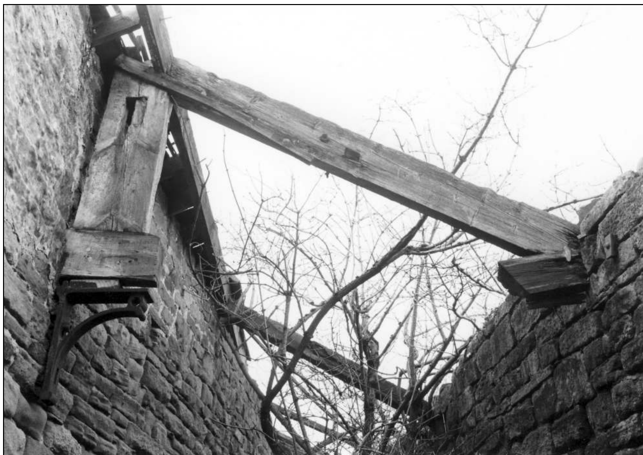
Photo 88: Detail of roof truss over boiler house, from the east (film 4, frame 11)
