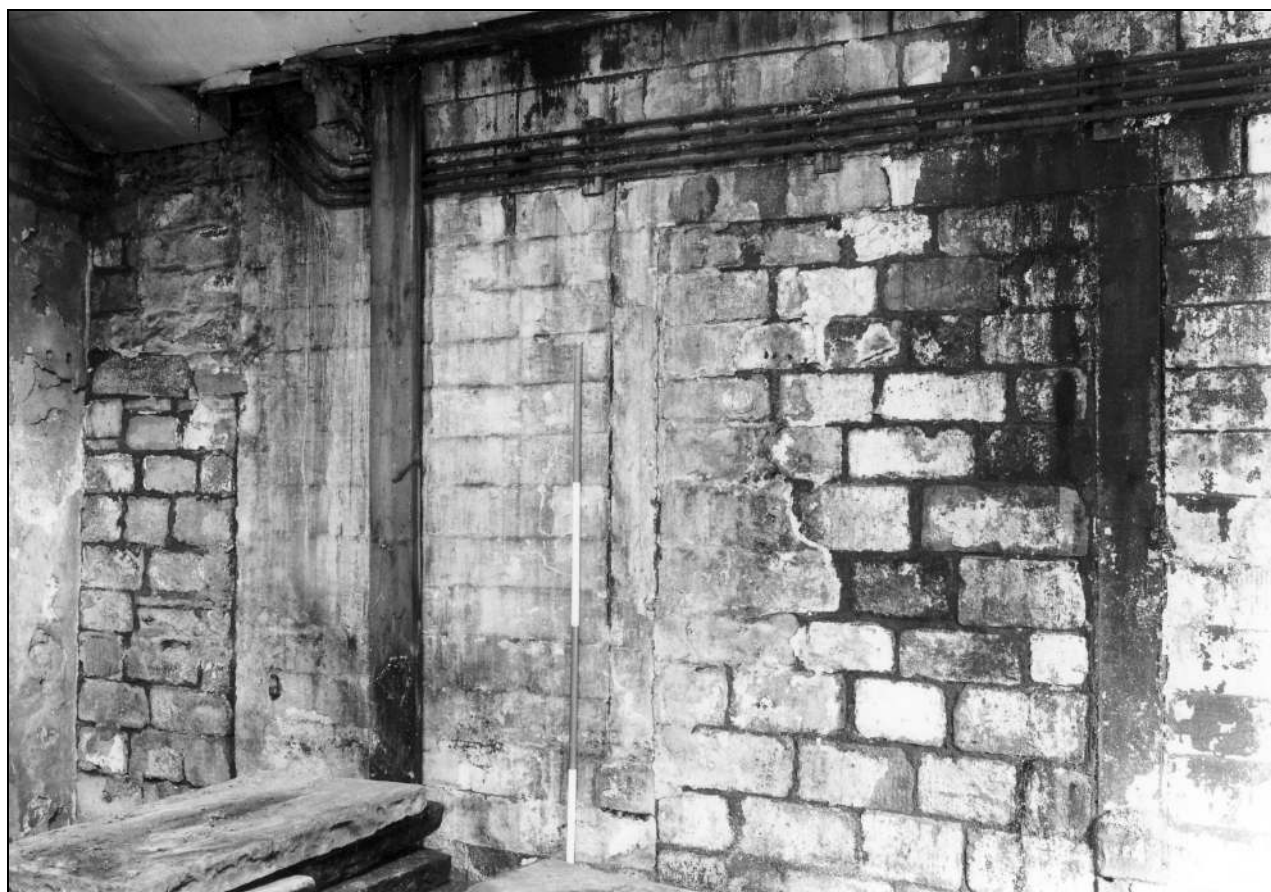
Photo 114: South side of warehouse, within later building, from the south (film 2, frame 18)
