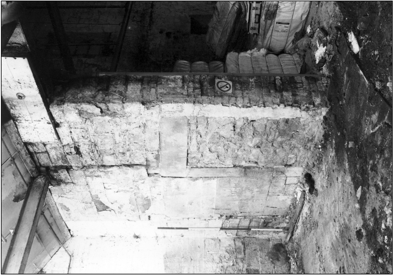
Photo 117: Blocked doorway in south-east corner of warehouse, from the north-west (film 2, frame 11)
