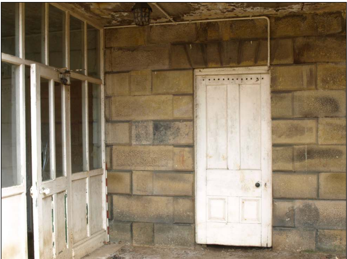
Photo 47: Detail of doorway in west front of the north arm of the service wing
