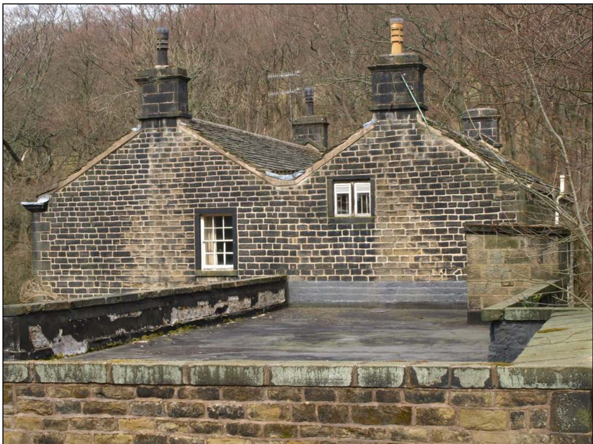
Photo 10: The south elevation, taken across the flat roof of the service wing
