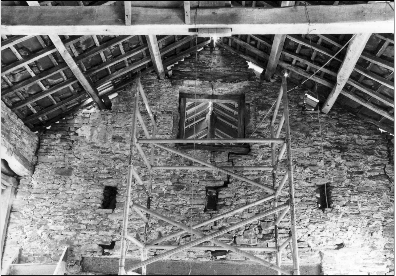
Photo 20: Interior view of upper part of south-west end of original barn, showing forking hole and breathers
