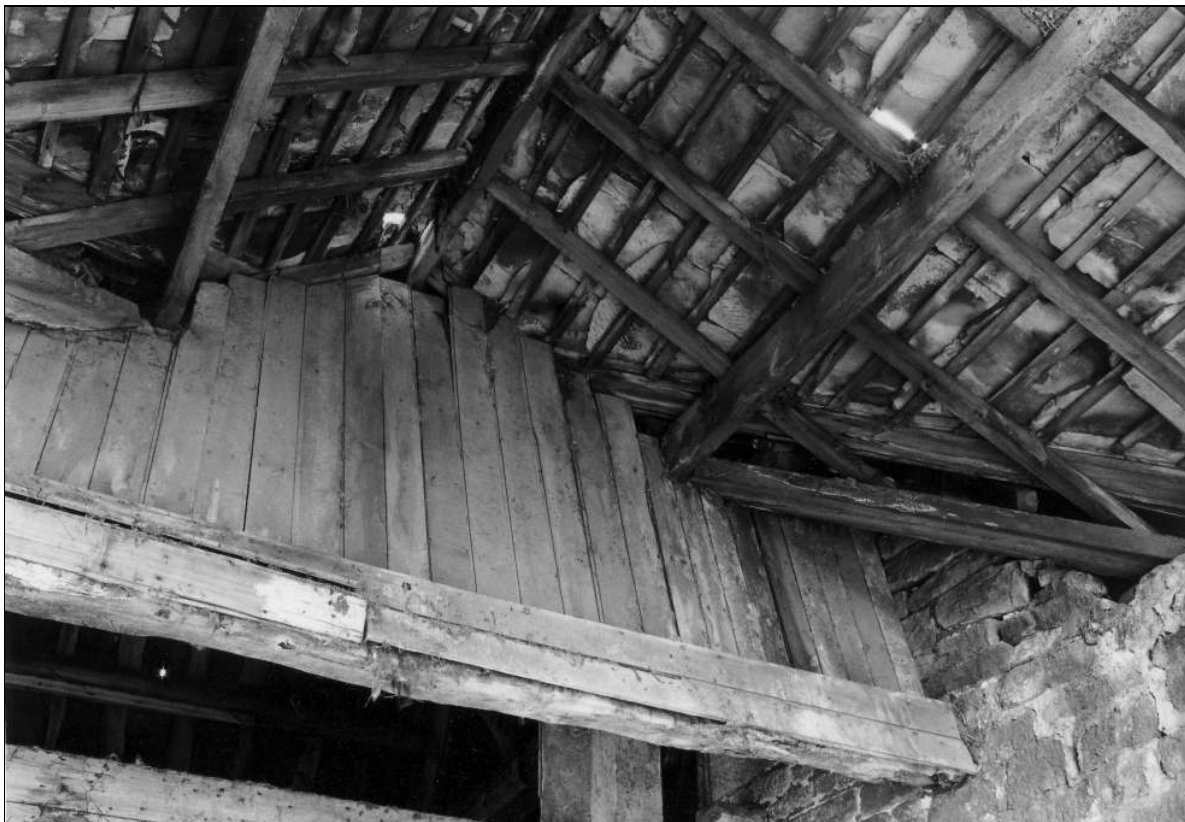
Photo 50: Interior of north-west entry, showing original door lintel and modern roof (film 3, frame 6)
