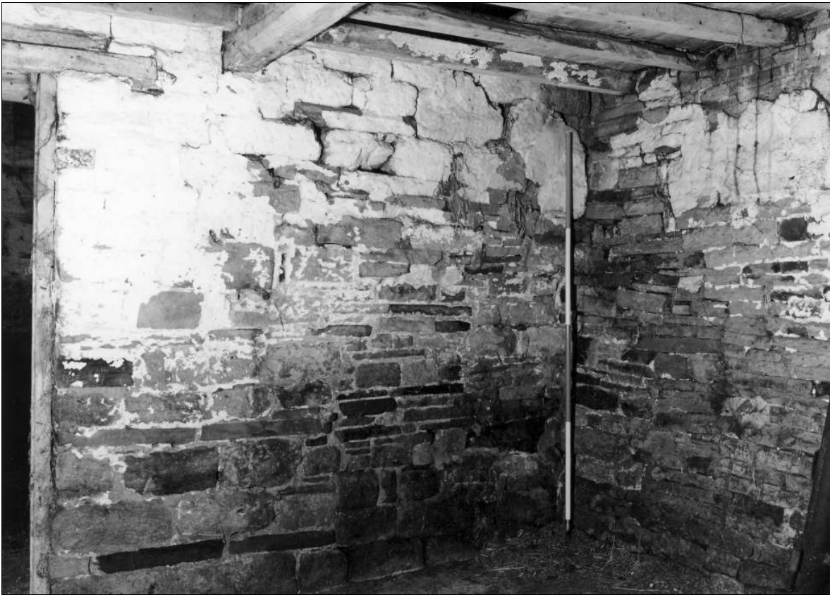
Photo 17: Stable: interior, from the north, showing north-east side of early wing (film 4, frame 3)
