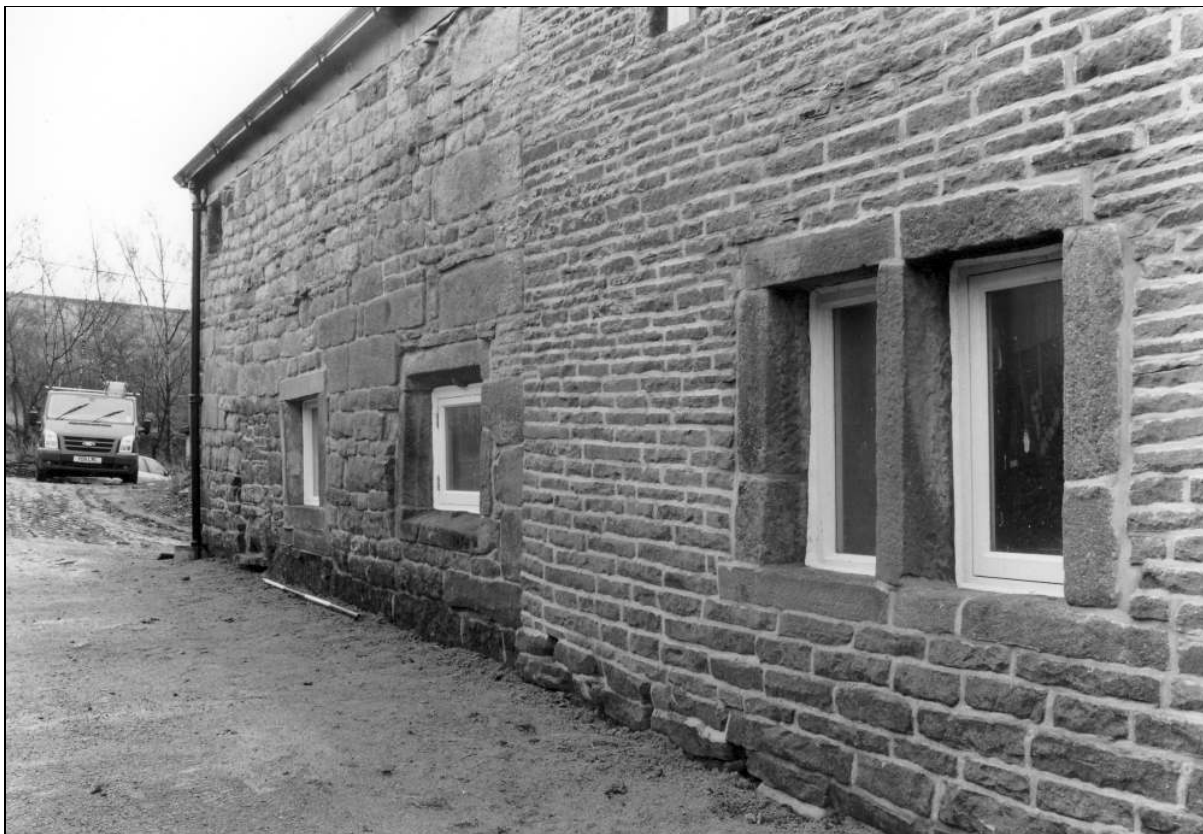
Photo 40: Stable: north-east elevation, after building work and reduction in ground level (film 7, frame 4)
