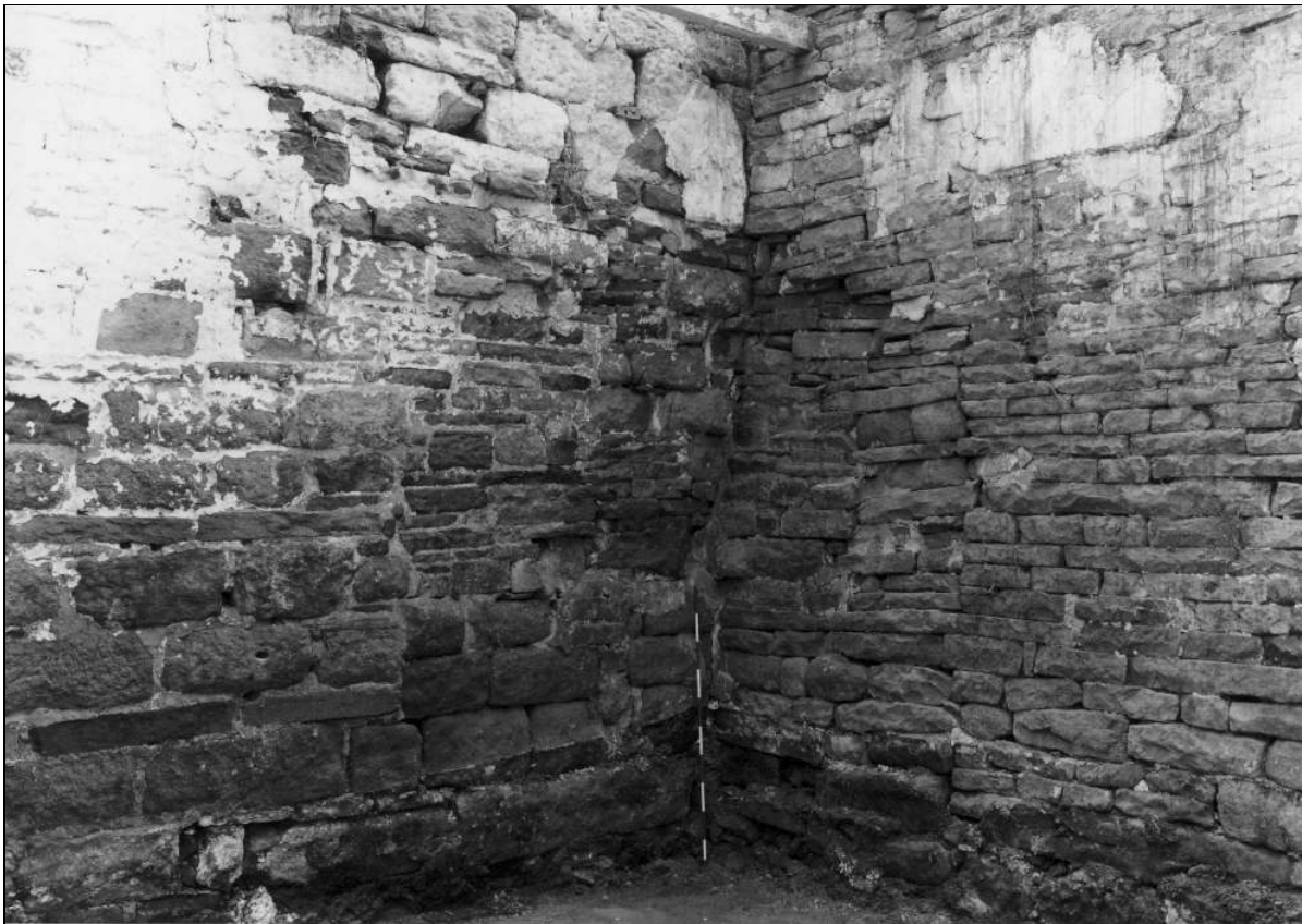
Photo 18: Stable: interior, from the north, showing north-east gable of early wing (during building works) (film 6, frame 13)
