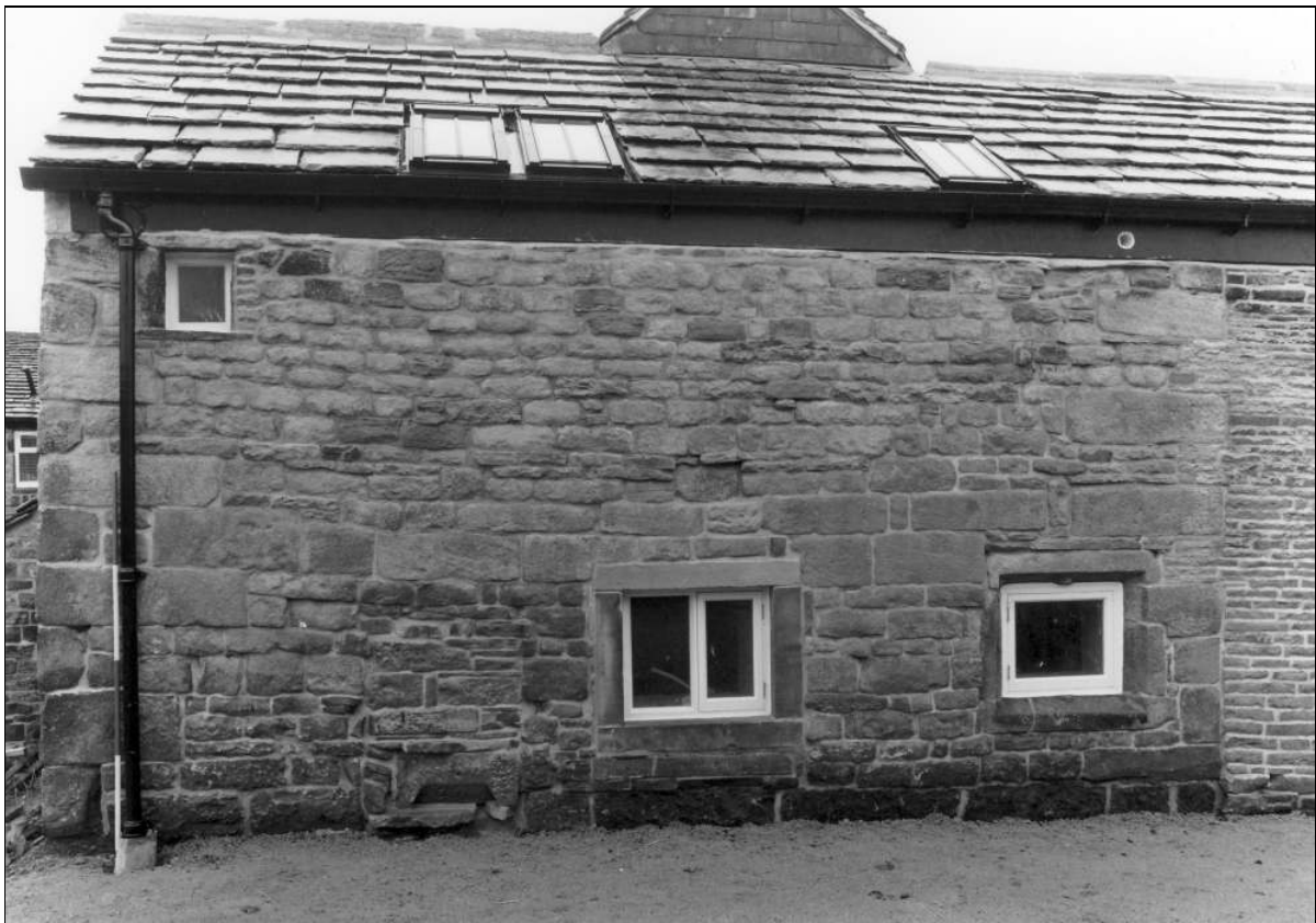
Photo 11: Early wing: north-east side, after building work and reduction in ground level (film 7, frame 3)
