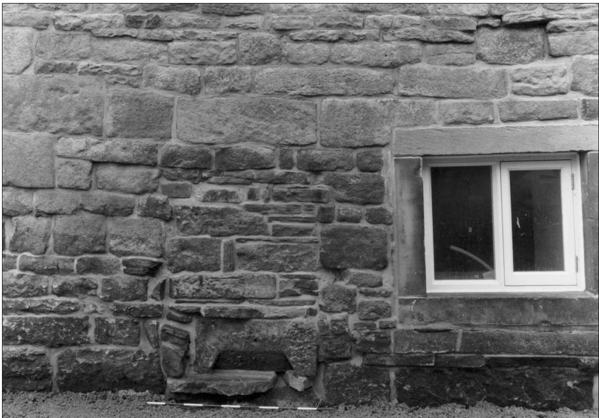
Photo 12: Early wing: detail of infilled opening, north-east side, after building work and reduction in ground level (film 7, frame 5)
