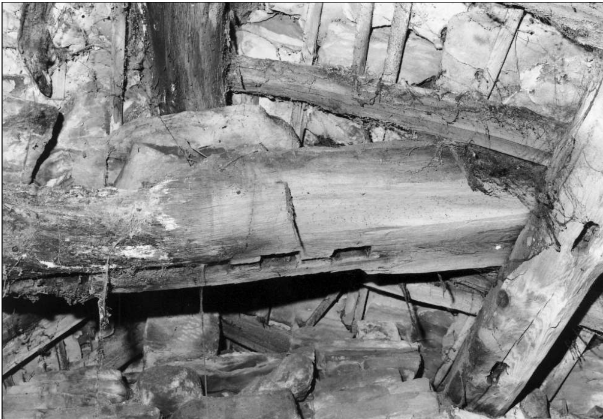
Photo 32: Early wing: detail of roof collar with mortices, from the south-east (film 3, frame 18)
