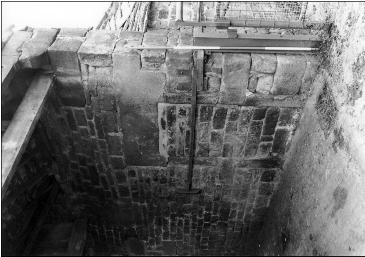
Photo 49: View into north-west entry of barn, showing blocked doorway to south-west (film 2, frame 6)
