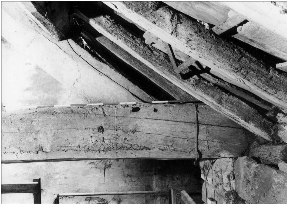
Photo 81: Barn interior: detail of south-east end of tie-beam to north-east roof truss, from the south-west (film 5, frame 11)
