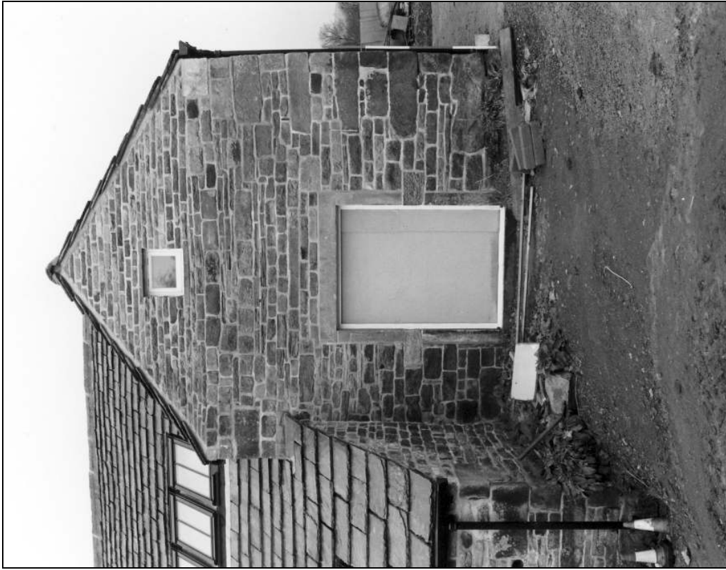
Photo 16: Early wing: south-east gable, after building work and reduction in ground level (film 7, frame 1)
