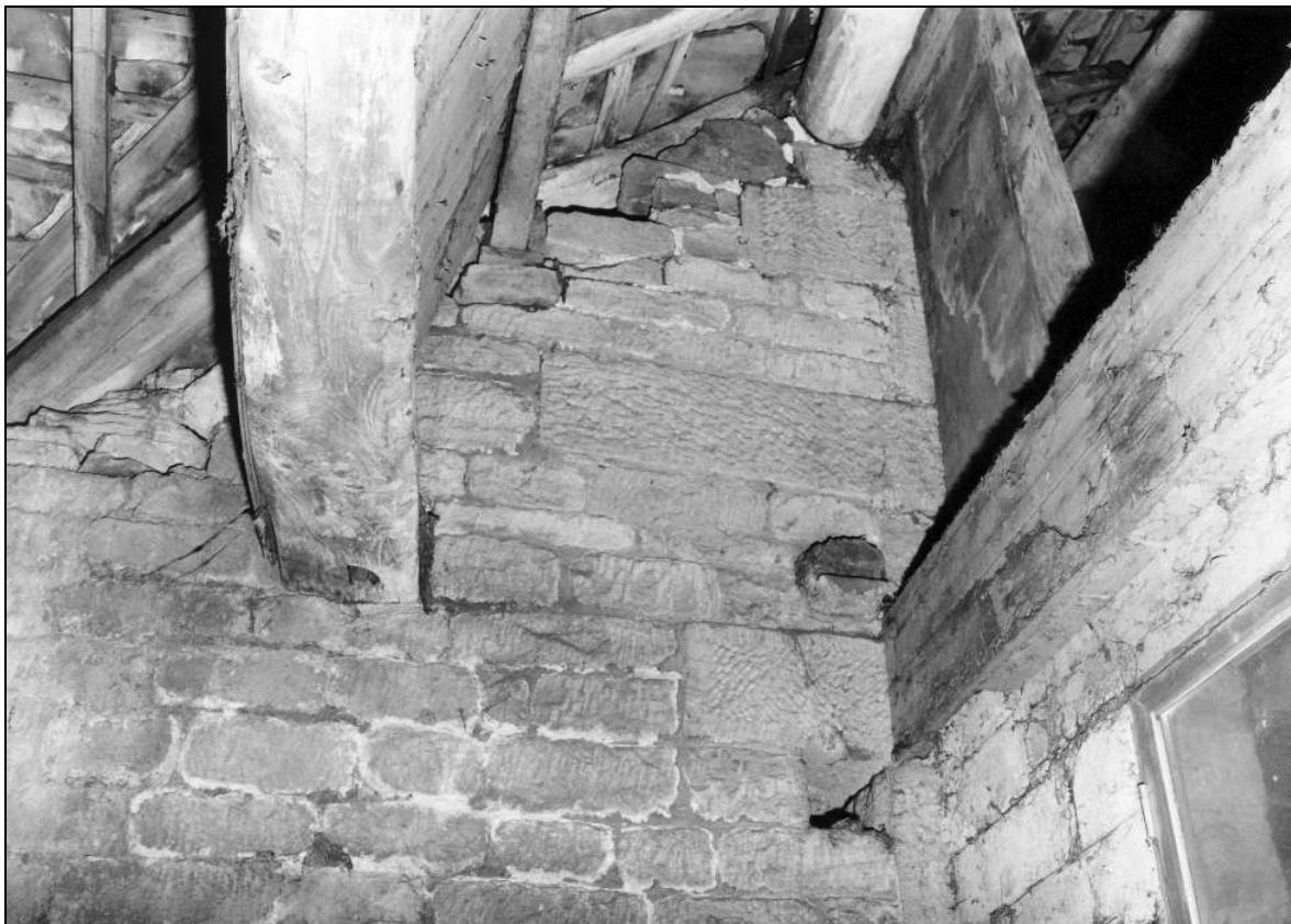
Photo 51: Interior of north-west entry, showing original door lintel (to left) with hinge hole (film 3, frame 4)
