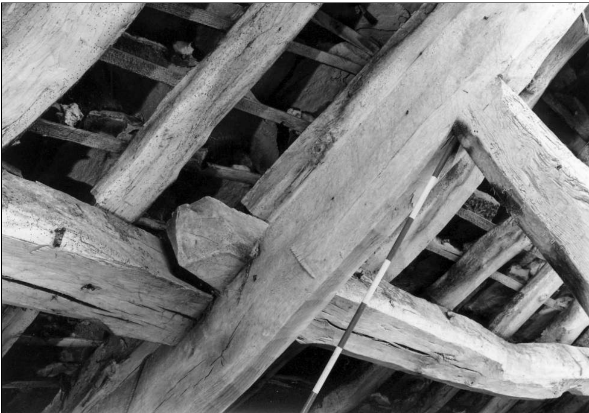
Photo 82: Barn interior: detail of purlin ends and joint numbering at strut in north-east roof truss, from the south (film 5, frame 10)
