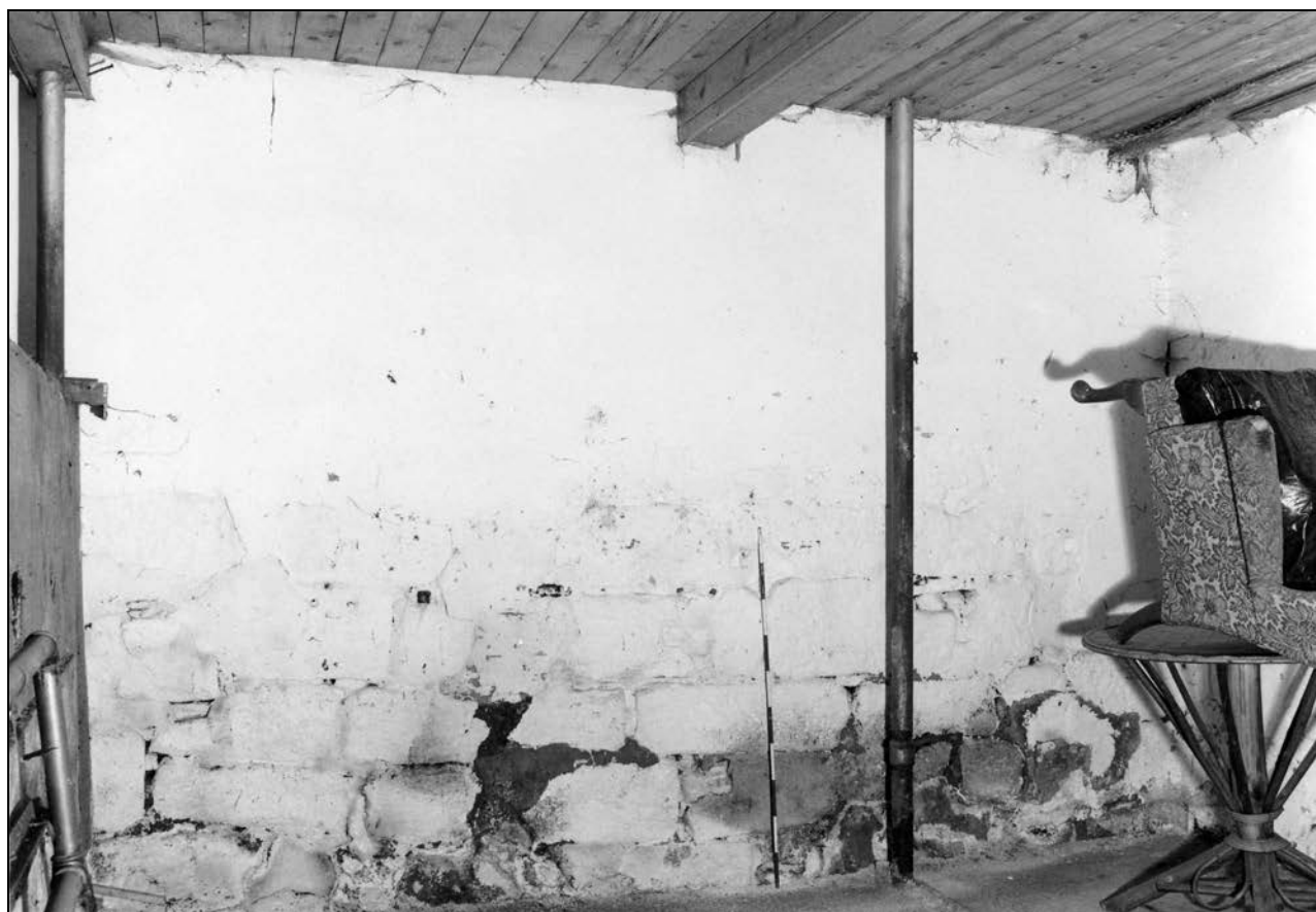
Photo 32: Retaining cross-wall in east end of barn, from the east (film 3, frame 7)
