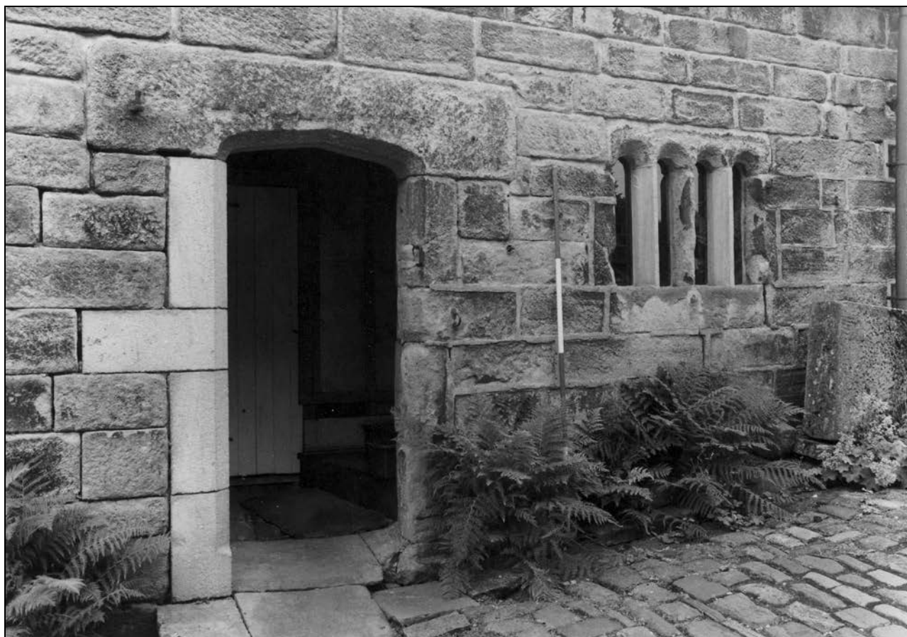
Photo 23: Doorway and window to former stable in north-east corner of barn (film 2, frame 15)
