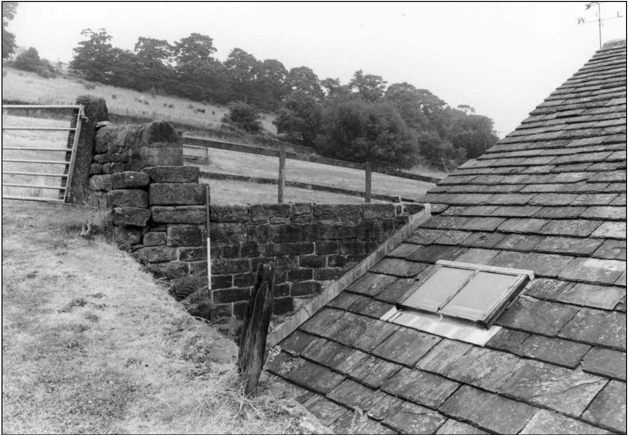
Photo 29: Parapet wall at south-west corner of barn, over later lean-to, from the east (film 1, frame 18)
