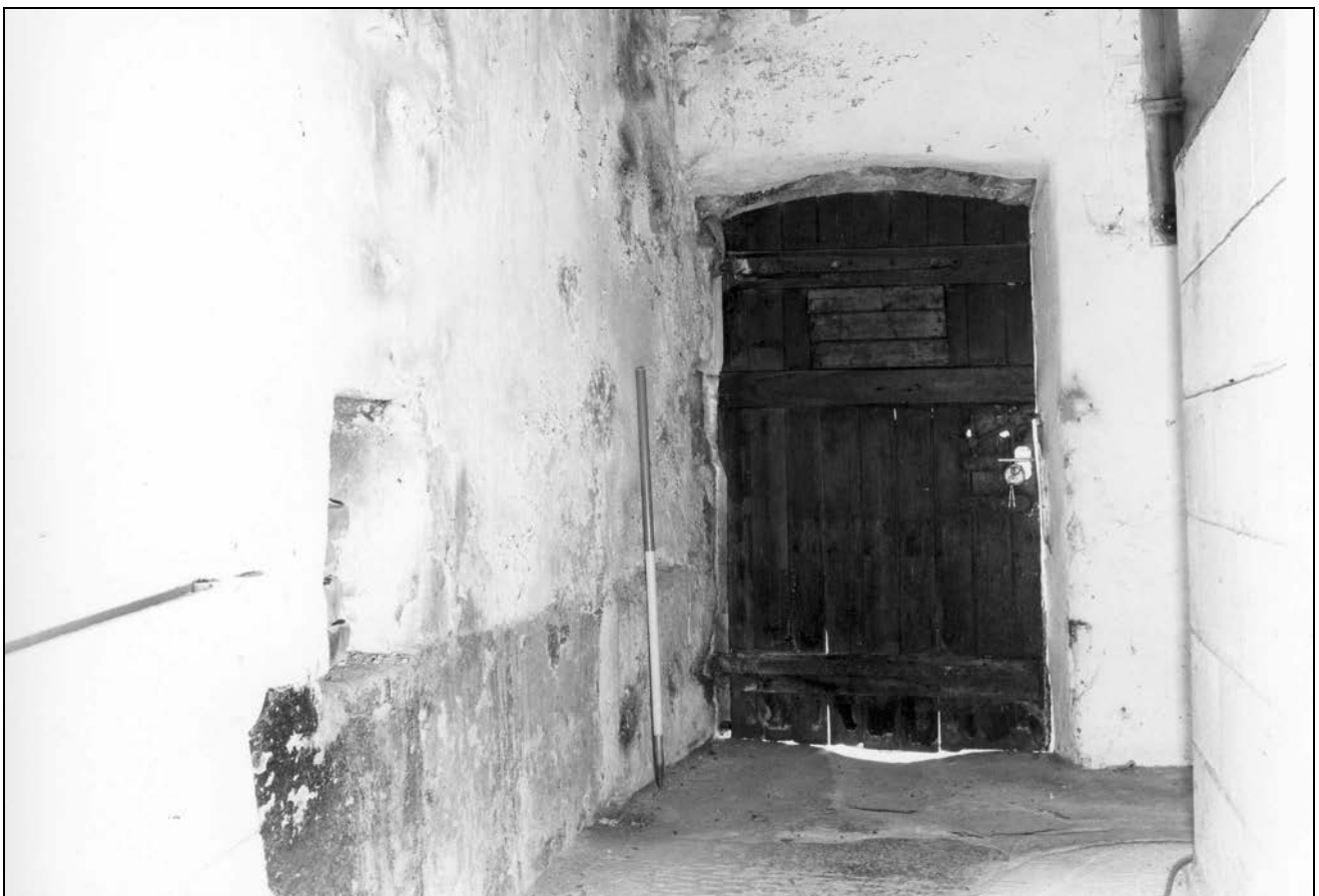
Photo 34: Interior view of doorway at south-east corner of the barn (film 3, frame 12)
