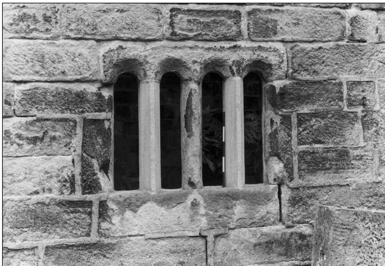
Photo 24: Detail of window to former stable in north-east corner of barn (film 2, frame 12)
