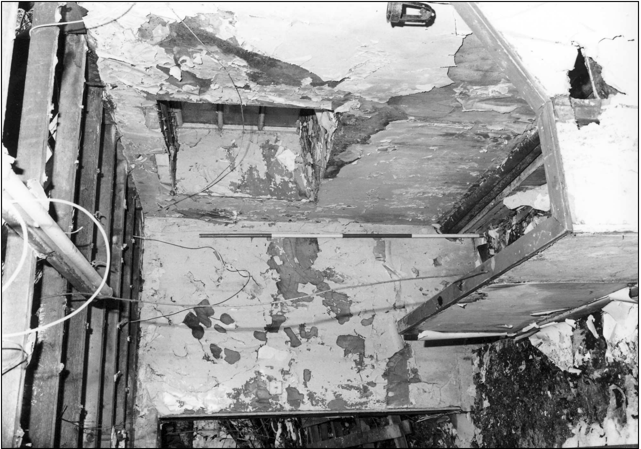
Photo 50: Cottage 3: modern stairs and inserted rear window on first floor (film 1, film 15)
