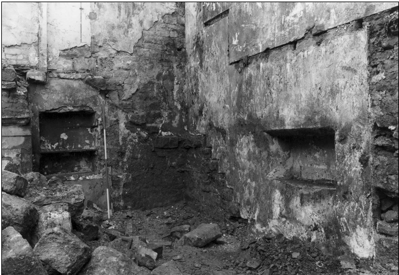
Photo 36: Cottage 1: rear part of former living room (formerly partitioned off), with recess in rear wall (film 5, film 10)
