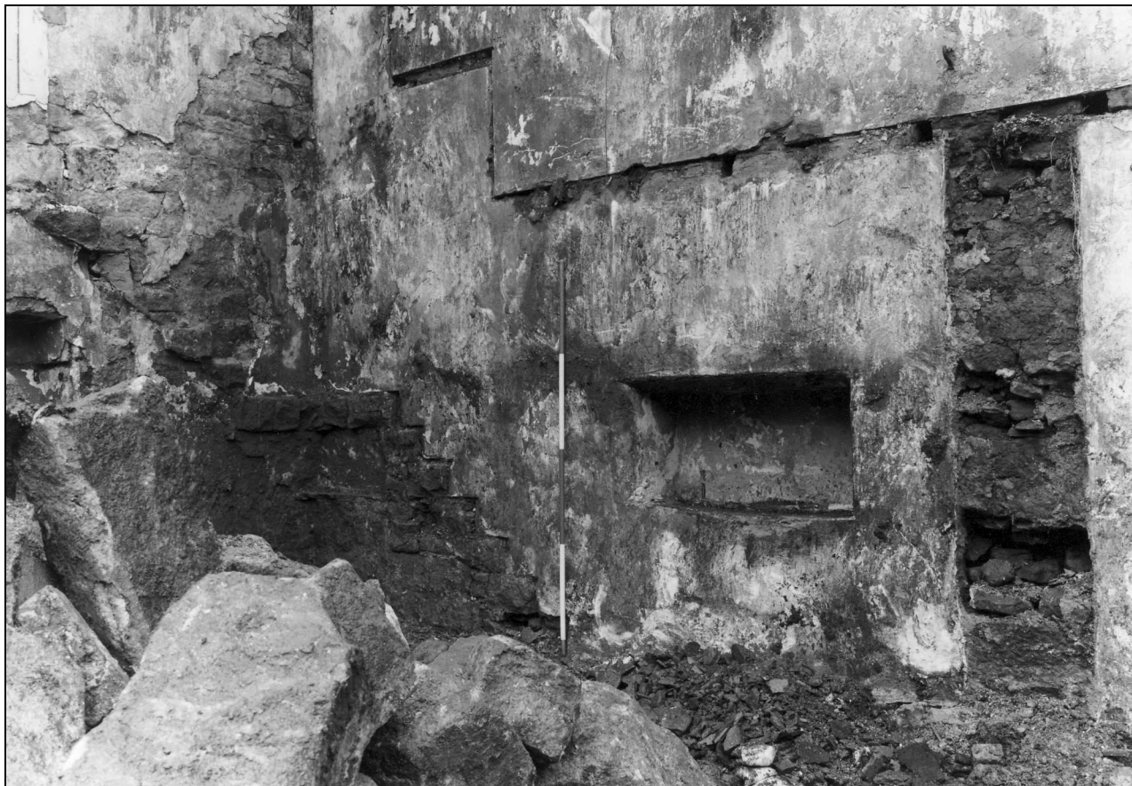
Photo 42: Cottage 1: ground floor interior during demolition, showing line of first floor and position of stairs (film 5, film 12)
