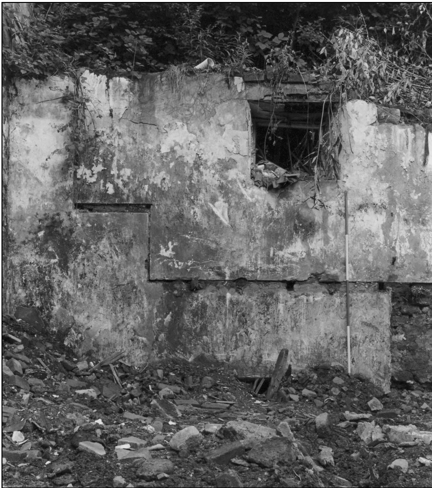
Photo 41: Cottage 1: rear wall, during demolition, showing line of first floor and position of stairs (film 5, film 8)
