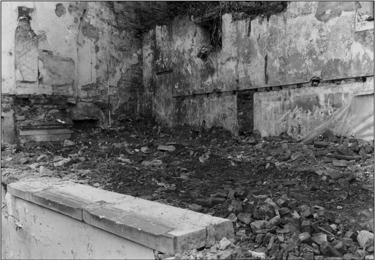
Photo 43: Cottages 1 and 2 during demolition (note modern window sill in foreground) (film 5, film 6)
