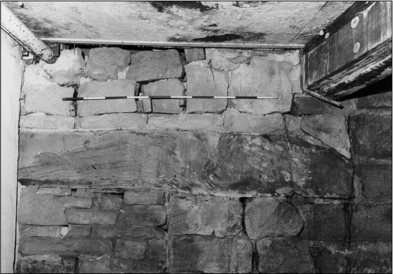
Photo 33: Cottage 2: south-west cross-wall on ground floor, showing oak timber (film 4, film 5)
