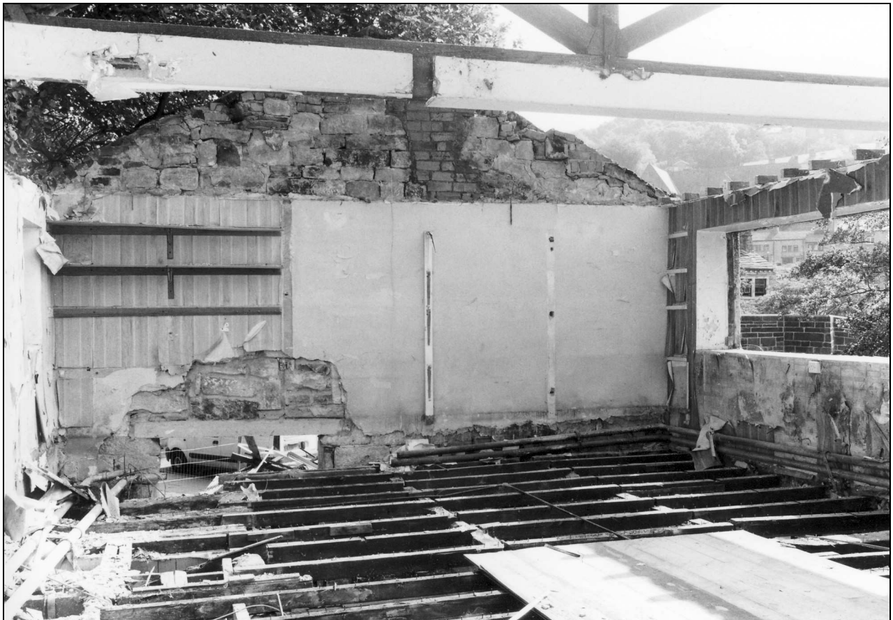
Photo 48: Cottage 4 during demolition, showing brick flue in gable and modern roof truss (film 4, film 2)
