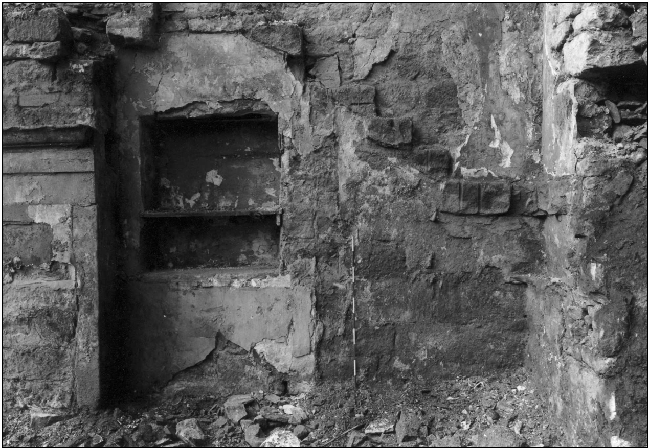
Photo 35: Cottage 1: remains of stairs in south-west gable (film 6, film 6)
