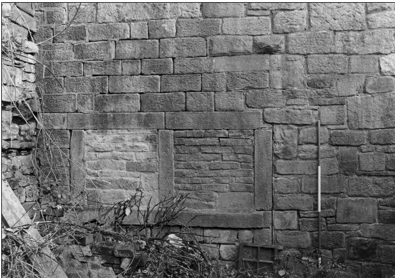
Photo 56: Retaining wall on north side of rear yard, with blocked windows of former building (film 3, film 1)
