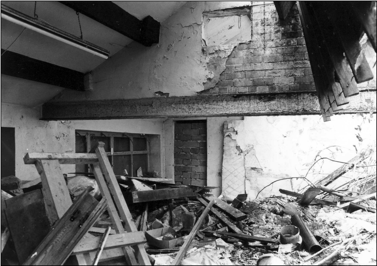
Photo 51: Cottages 2 & 3: first floor, with modern steel beam and roof structure, from the north-east (film 1, film 12)
