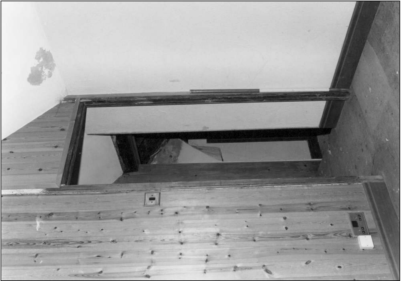
Photo 58: Doorway to bedroom 3, within historic partition with modern cladding, from the south-east (film 4, frame 16)
