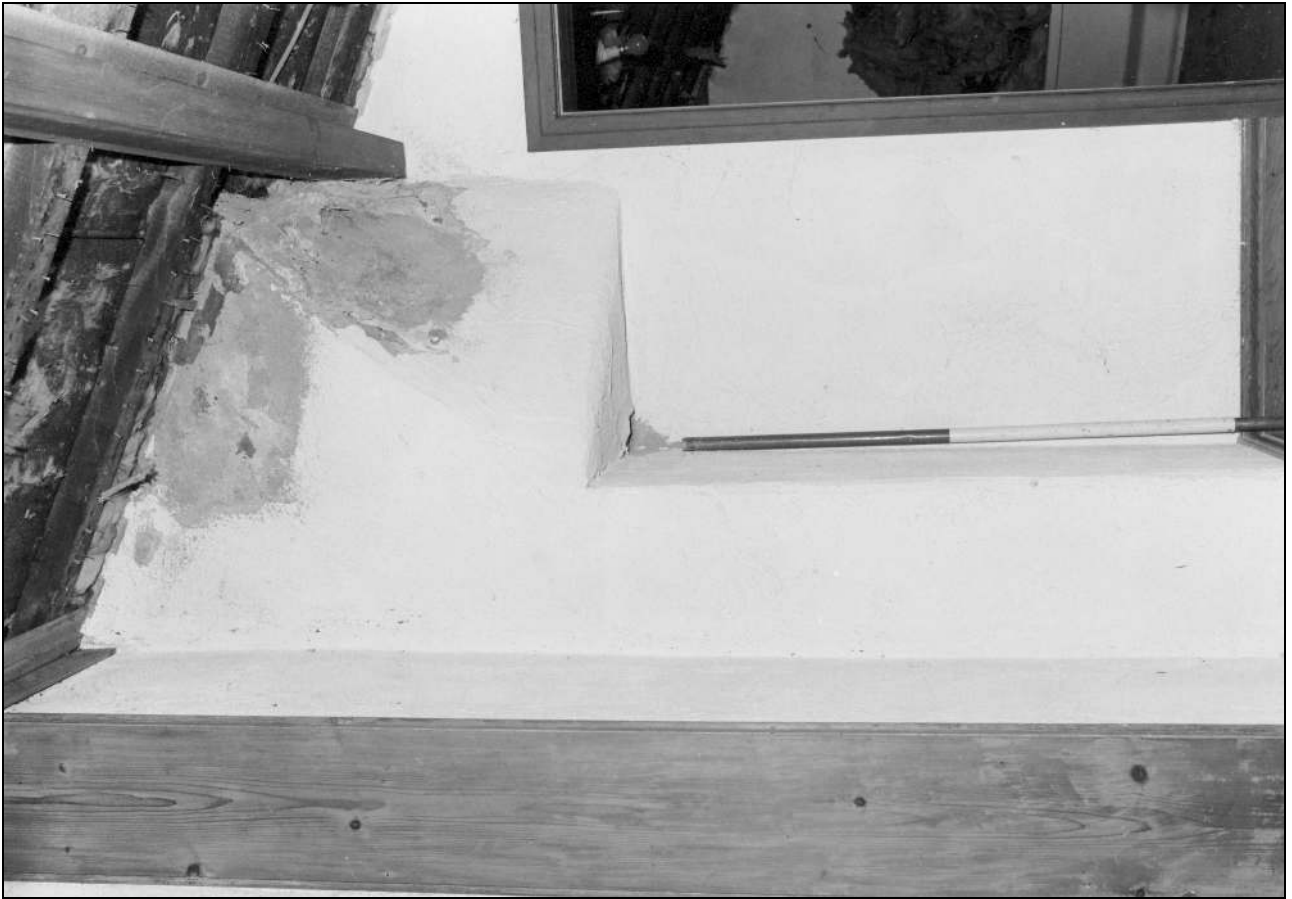
Photo 48: Detail of corbelled chimney stack on first floor, from the north-east (film 4, frame 4)
