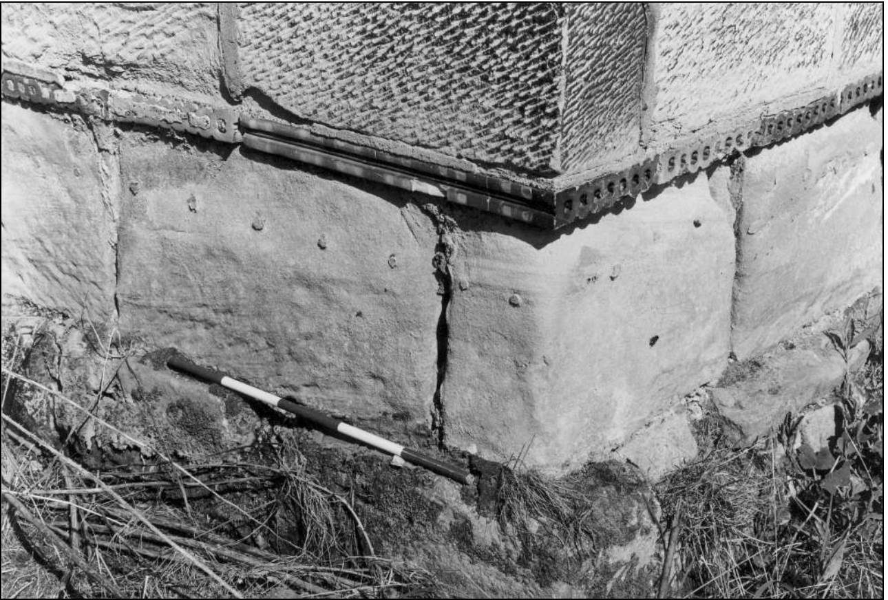
Photo 6: Detail of tile damp-course in front elevation (film 3, frame 13)
