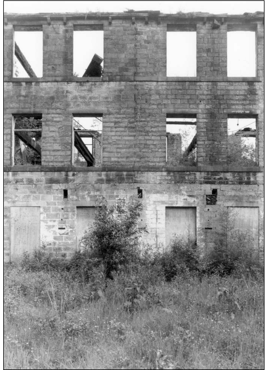
Photo 5: Spinning mill: straight joint in south elevation (film 3, frame 3)
