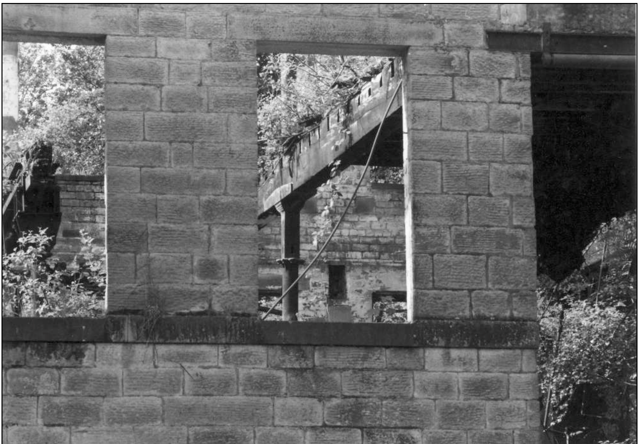
Photo 22: Spinning mill: view through north elevation to interior on first floor, showing cast iron column and timber beam (film 1, frame 7)
