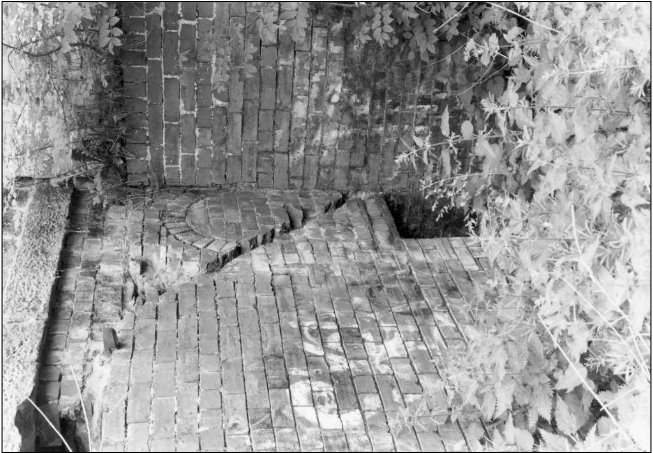
Photo 41: Flue(?) in south gable of boiler house (film 2, frame 13)
