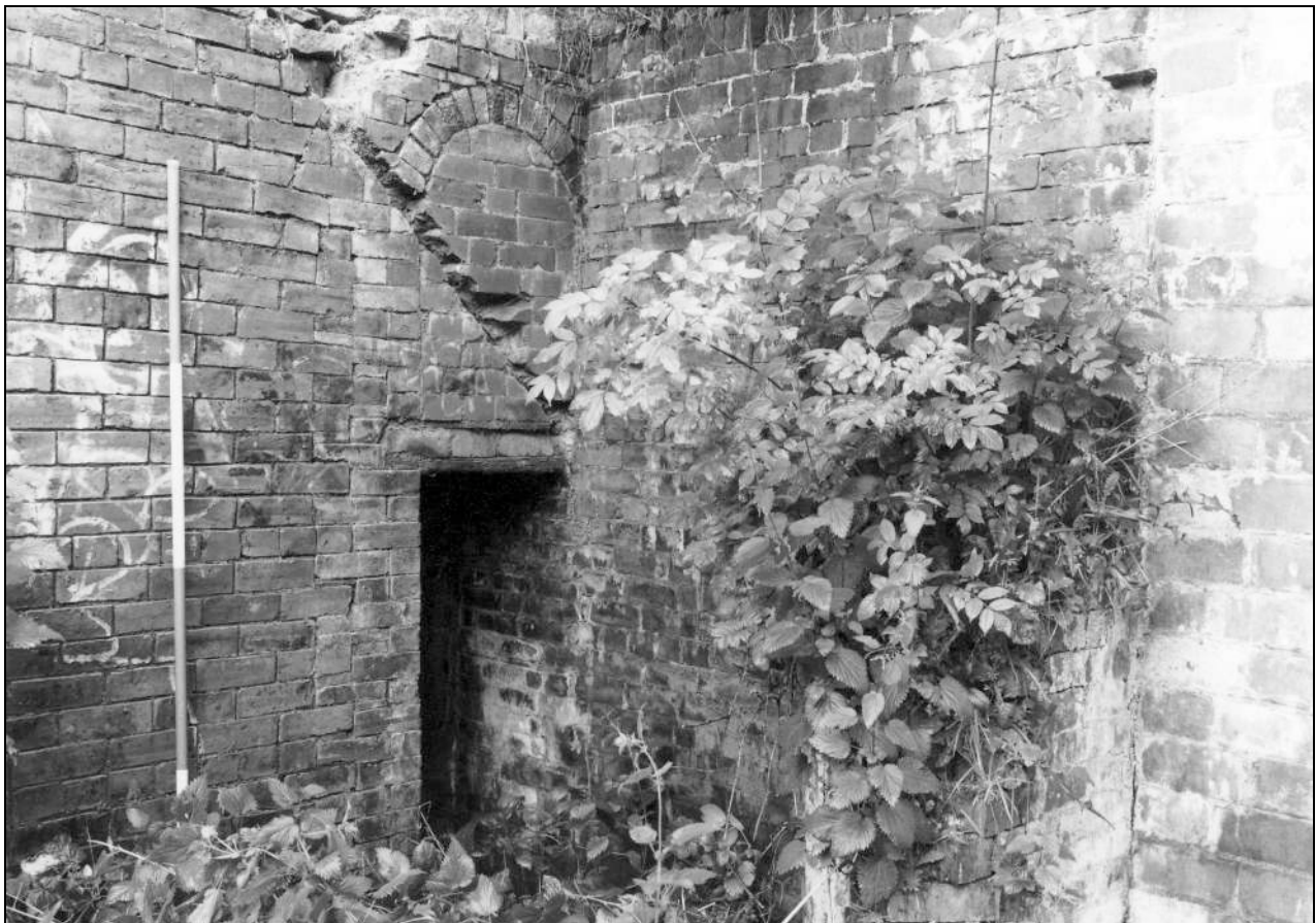
Photo 42: Flue(?) in south gable of boiler house (film 4, frame 4)
