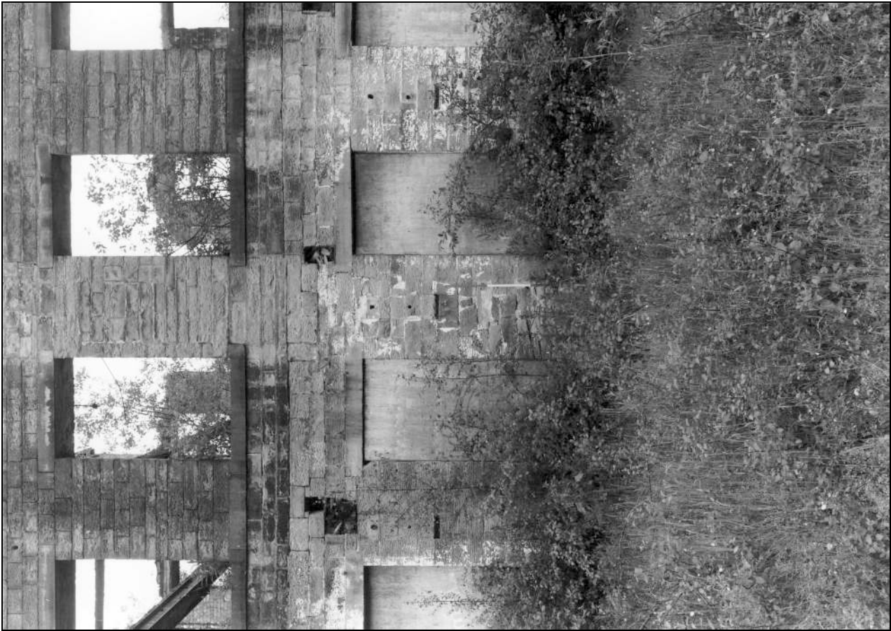
Photo 8: Spinning mill: break in sill band in south elevation (film 4, frame 1)
