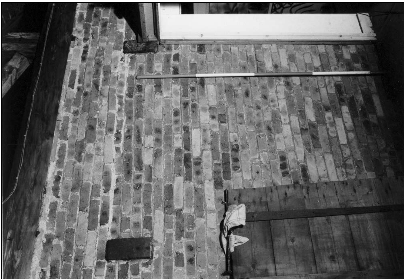
Photo 37: Detail of brick wall to east of central bay, at first floor level (film 3, frame 18)
