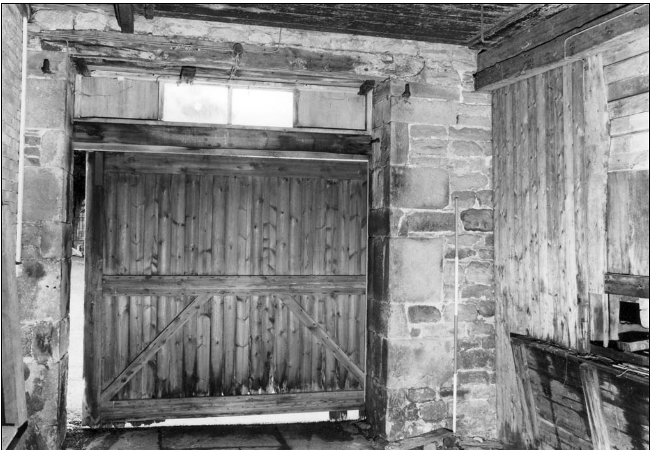
Photo 36: South doorway to central bay, with internal hinges for original doors (film 3, frame 5)
