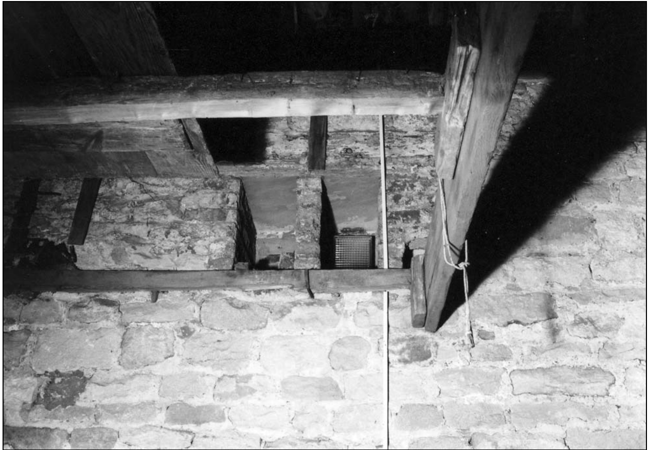
Photo 41: Internal view of entrance to former pigeon loft in central bay, with remains of timber structure (film 3, frame 16)
