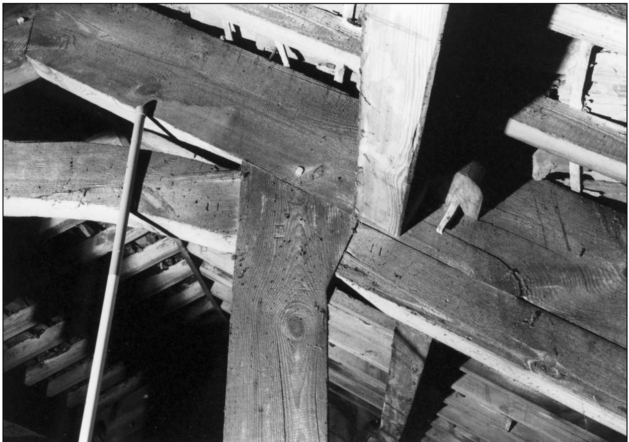
Photo 65: Detail of joints and numbering on east side of east roof truss (film 4, frame 17)
