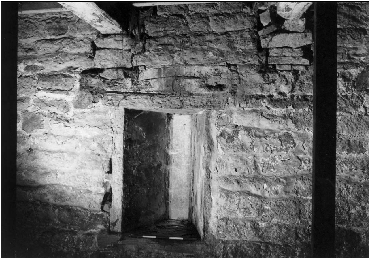
Photo 28: Internal view of breather in west side of stable, with raised loft beams above (film 2, frame 12)
