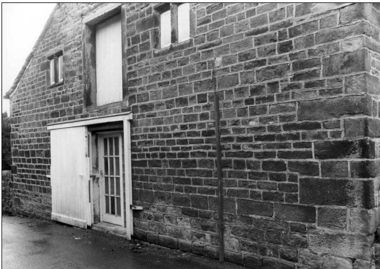
Photo 10: East gable, with doorways to first floor and attic of workshop (film 1, frame 17)
