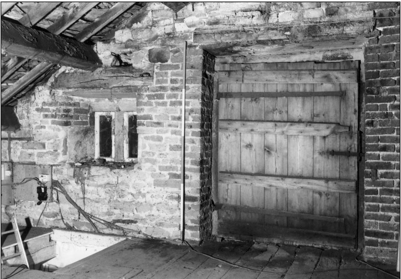
Photo 58: Attic over workshop, with gable taking-in doorway, from the south-west (film 4, frame 11)
