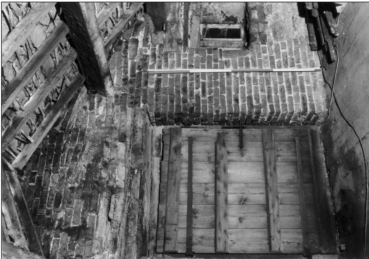
Photo 59: Attic over workshop, with gable taking-in doorway, from the north-west (film 4, frame 12)
