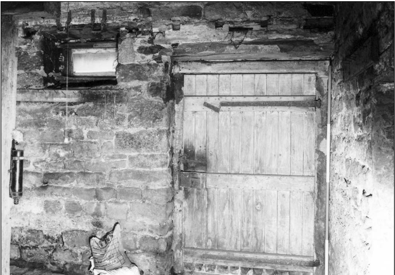
Photo 24: Internal view of doorway and window to stable, from the north (film 2, frame 17)
