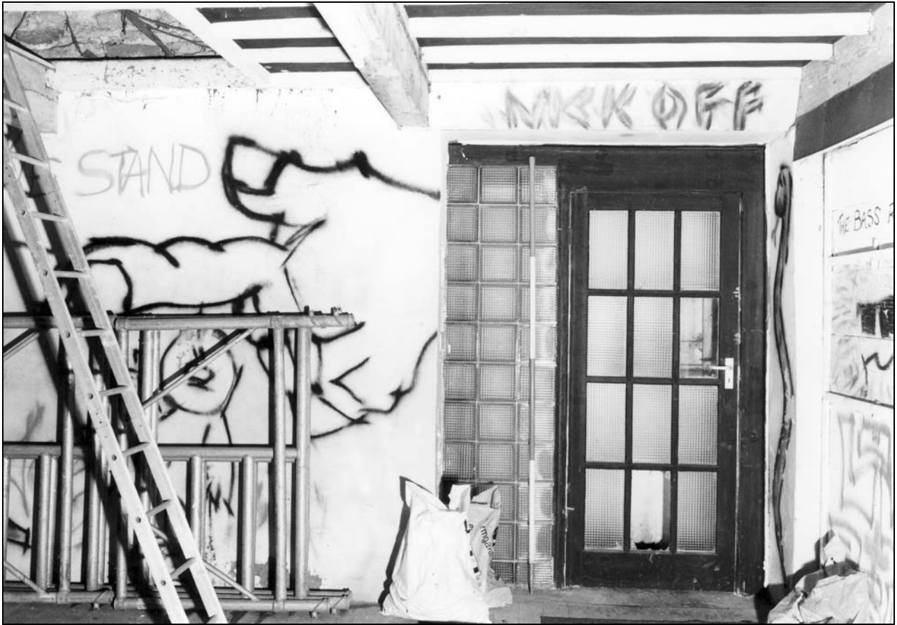
Photo 57: First floor of workshop (north part), with gable doorway to road level (film 4, frame 10)
