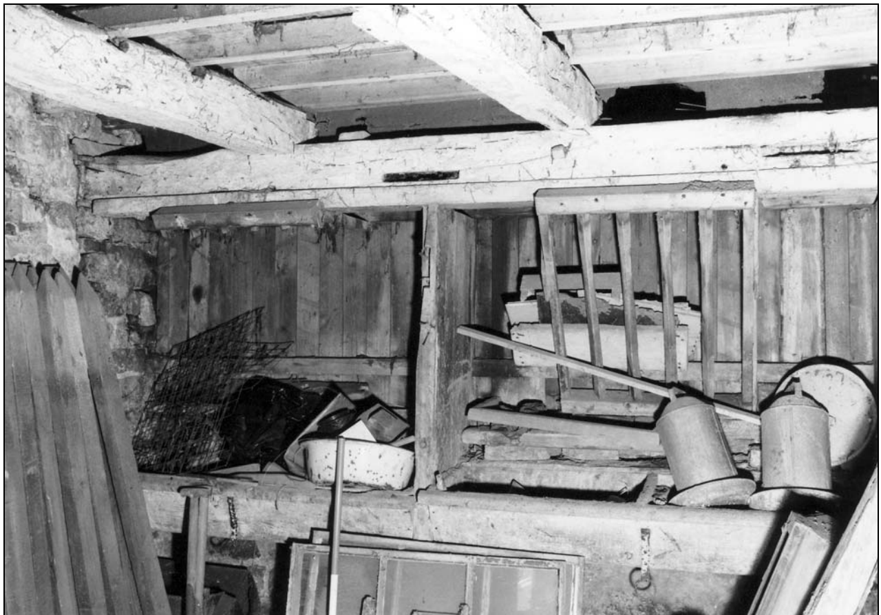
Photo 26: Stable fixtures in former shippon, from the west, with raised loft beams overhead (film 2, frame 11)
