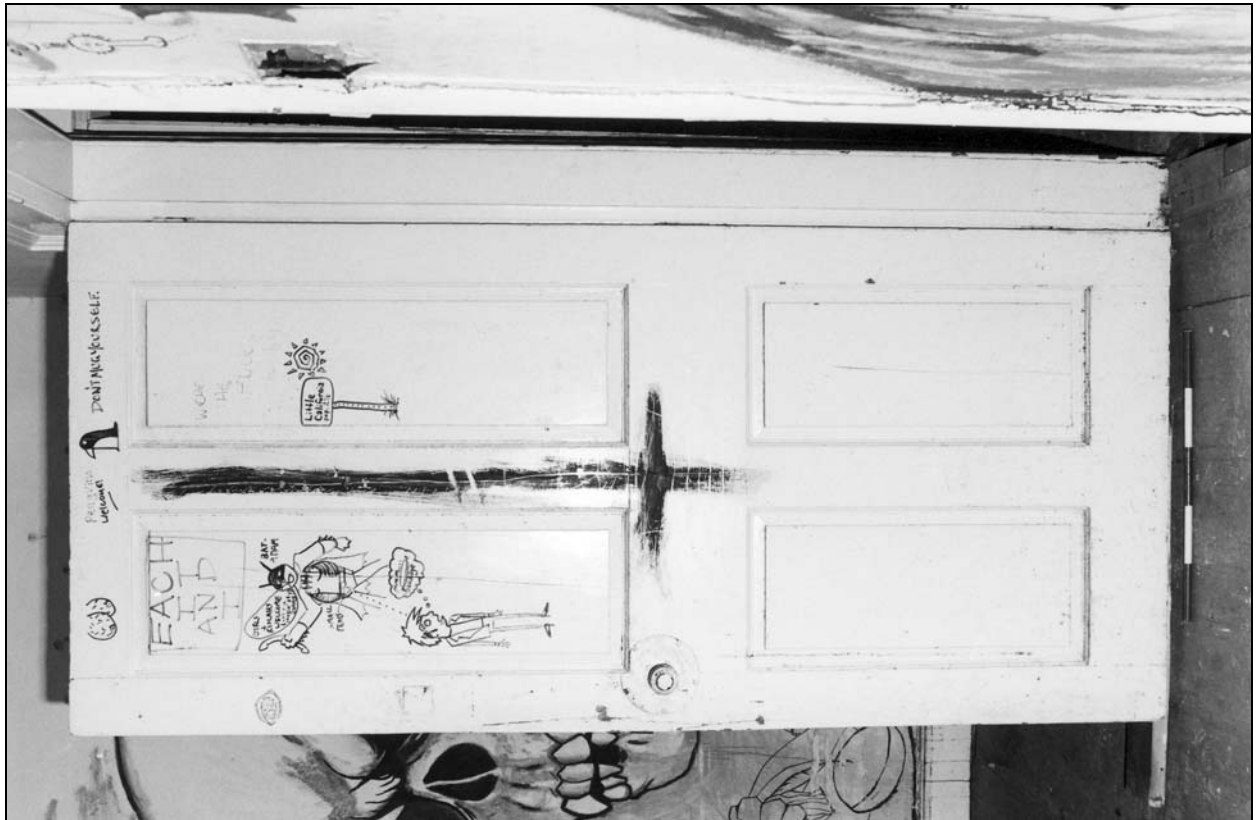
Photo 49: South wing: outer face of door to west second floor room S01 (film 6, frame 9)
