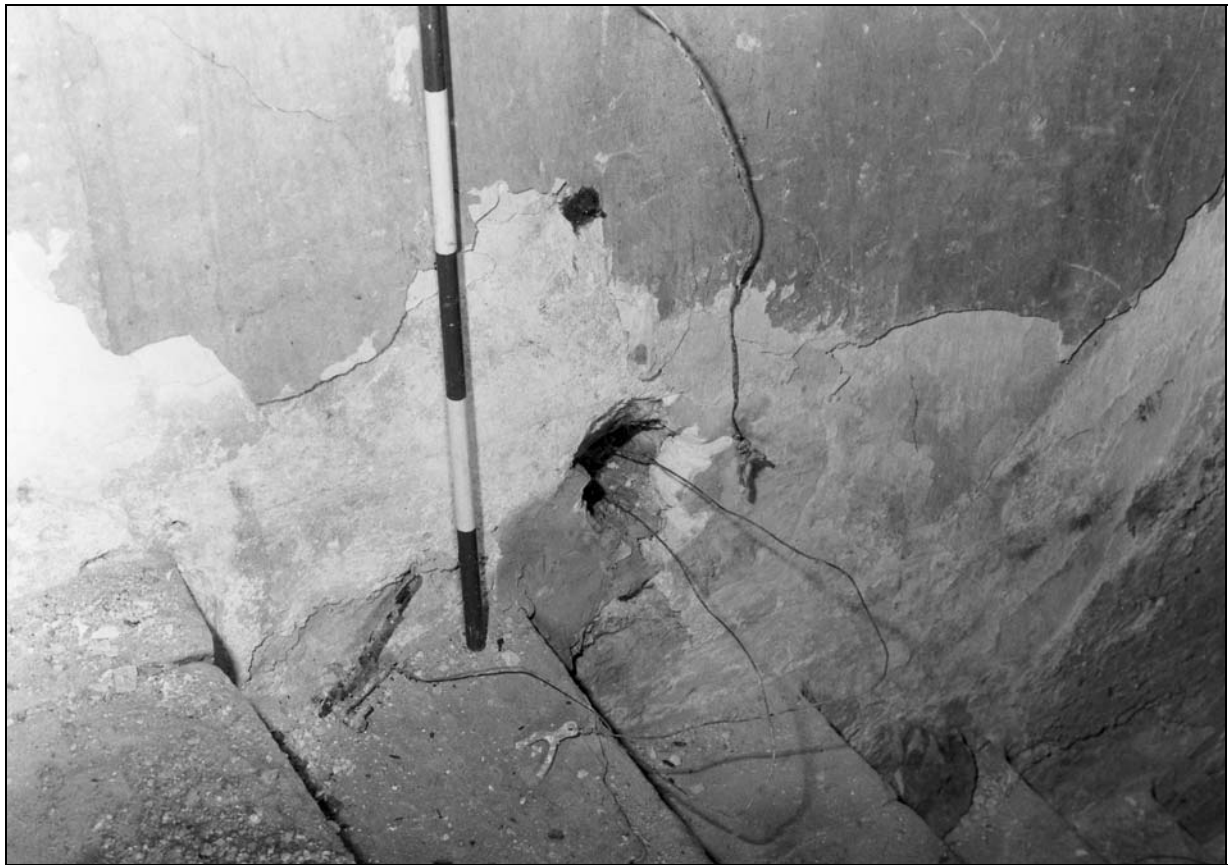
Photo 63: North wing: remains of bell wires at top of stairs down to cellar (film 2, frame 3)
