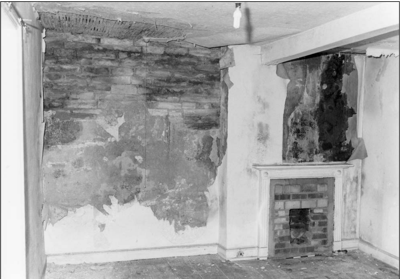
Photo 70: North wing: west first floor room F03, from the south-west (film 6, frame 12)
