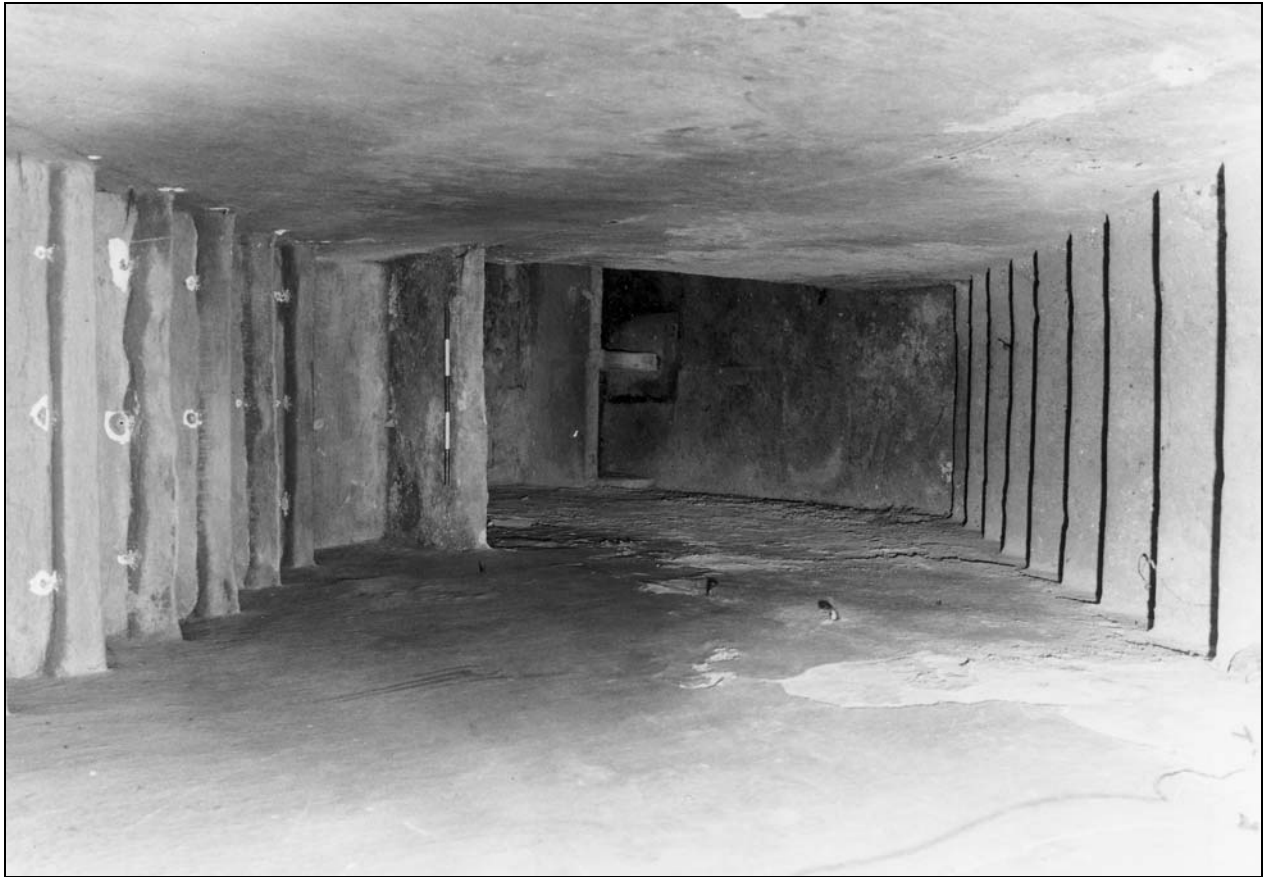
Photo 62: North wing: stairs down to cellar B01 (film 2, frame 1) 59: North wing: blocked fireplace in back kitchen G03 (film 3,
