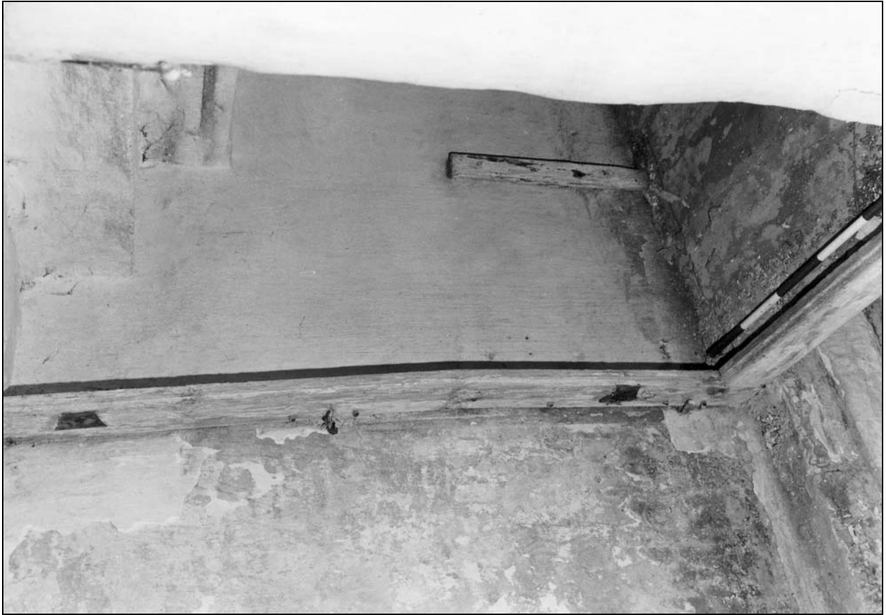
Photo 36: South wing: remains of cupboard by steps down to cellar B02 (film 1, frame 12)
