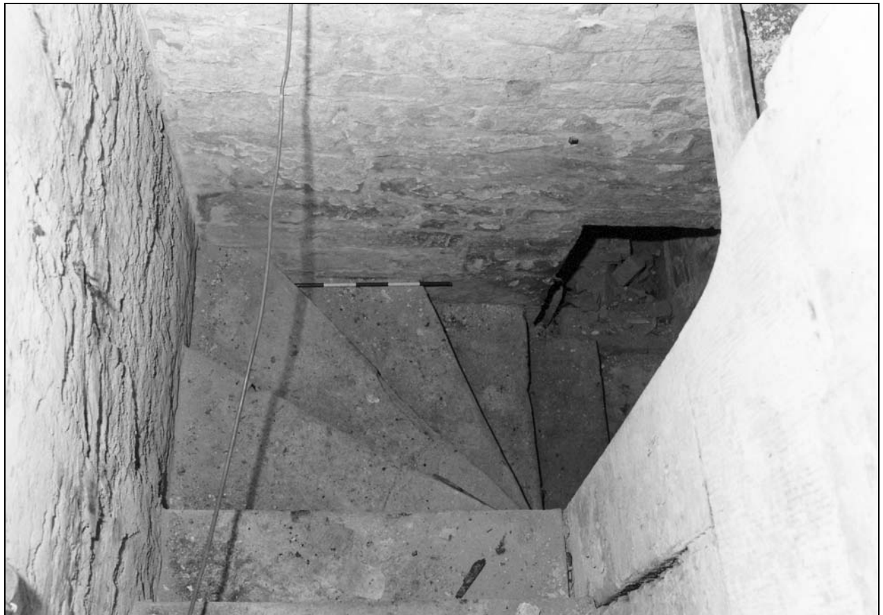
Photo 34: South wing: steps down to cellar B02, from the west (film 1, frame 13)
