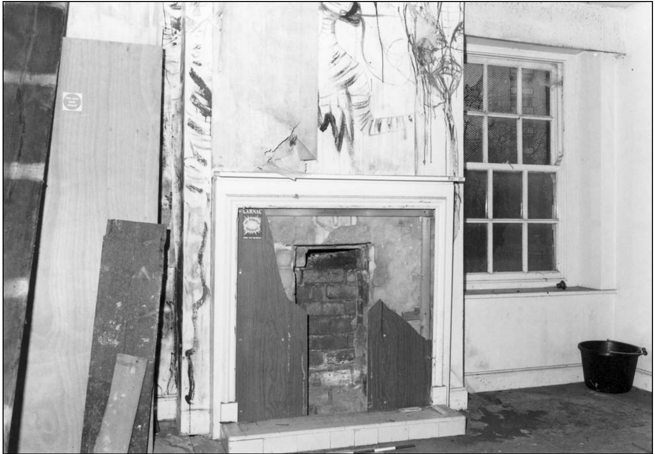
Photo 79: North wing: east second floor room S06, from the south (film 6, frame 16)
