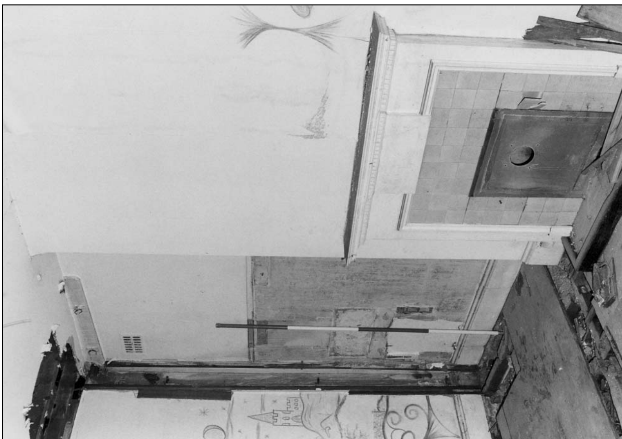
Photo 45: South wing: fireplace in east first floor room F02, from the south-west (film 4, frame 4)
