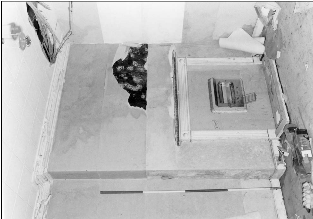
Photo 76: North wing: west second floor room S04, from the south-west (film 5, frame 18)
