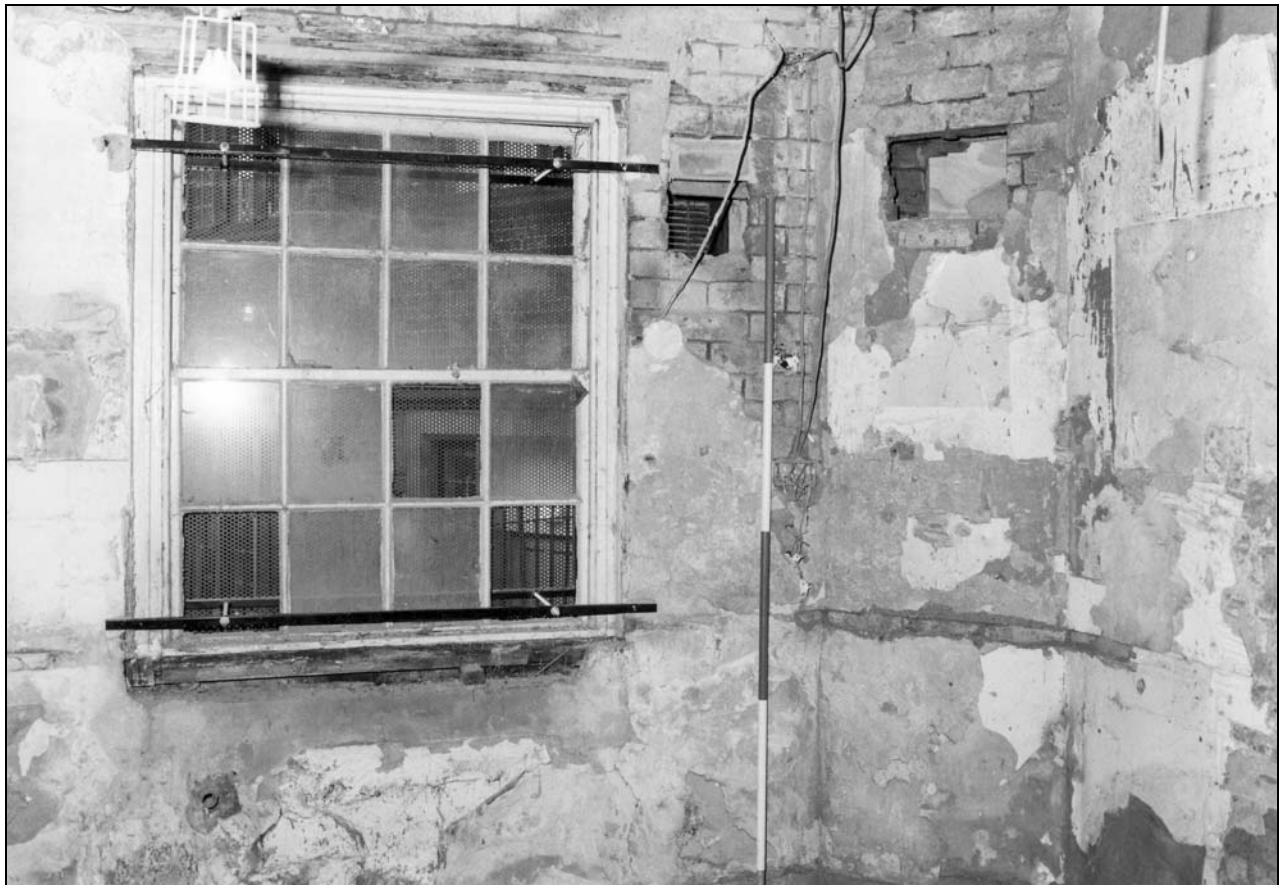
Photo 60: North wing: window in back kitchen G03, from the east (film 3, frame 17)
