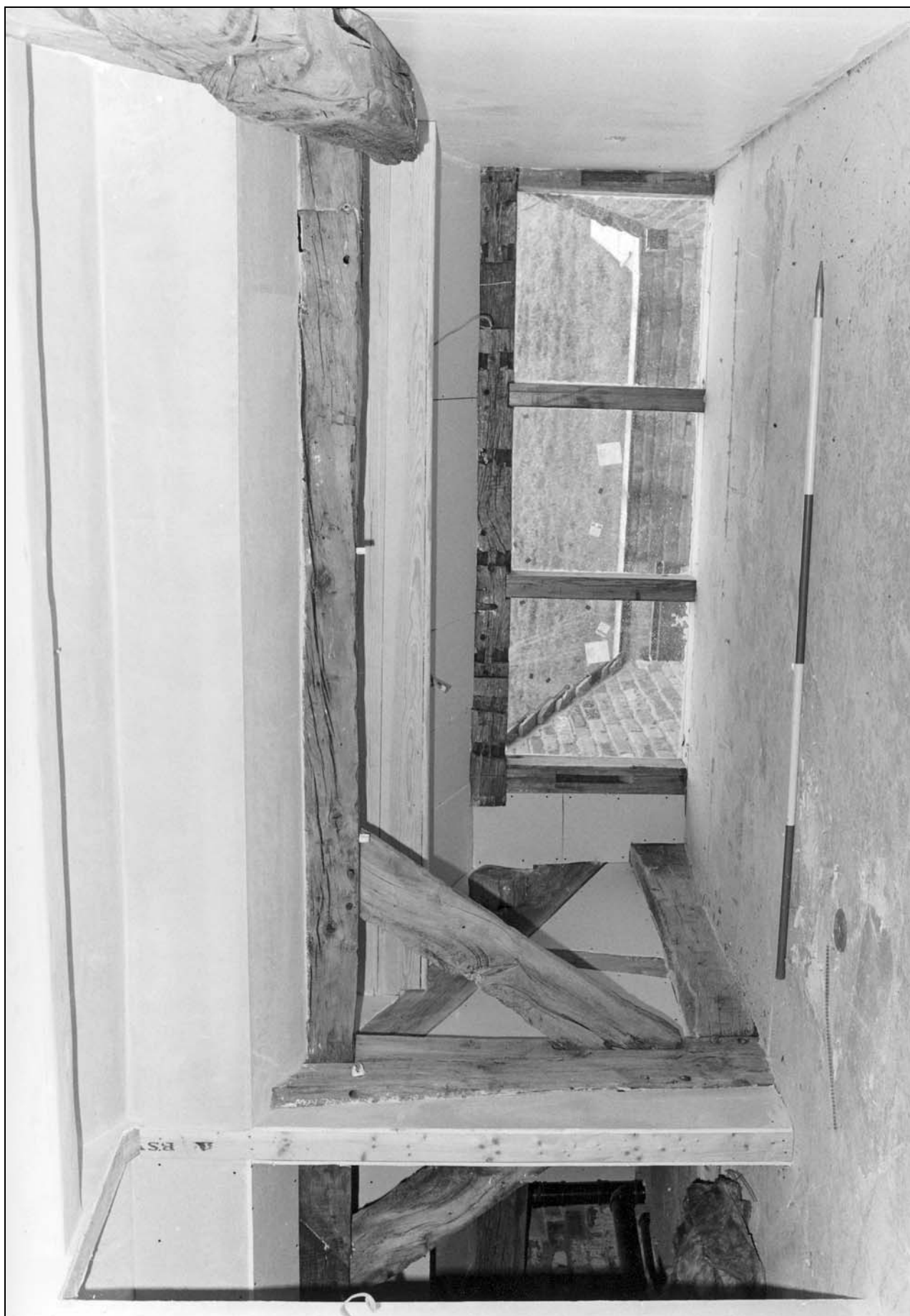
Photo 9: First floor view towards west cart entry, showing arcade post of truss 4 at left (film 1, frame 8)
