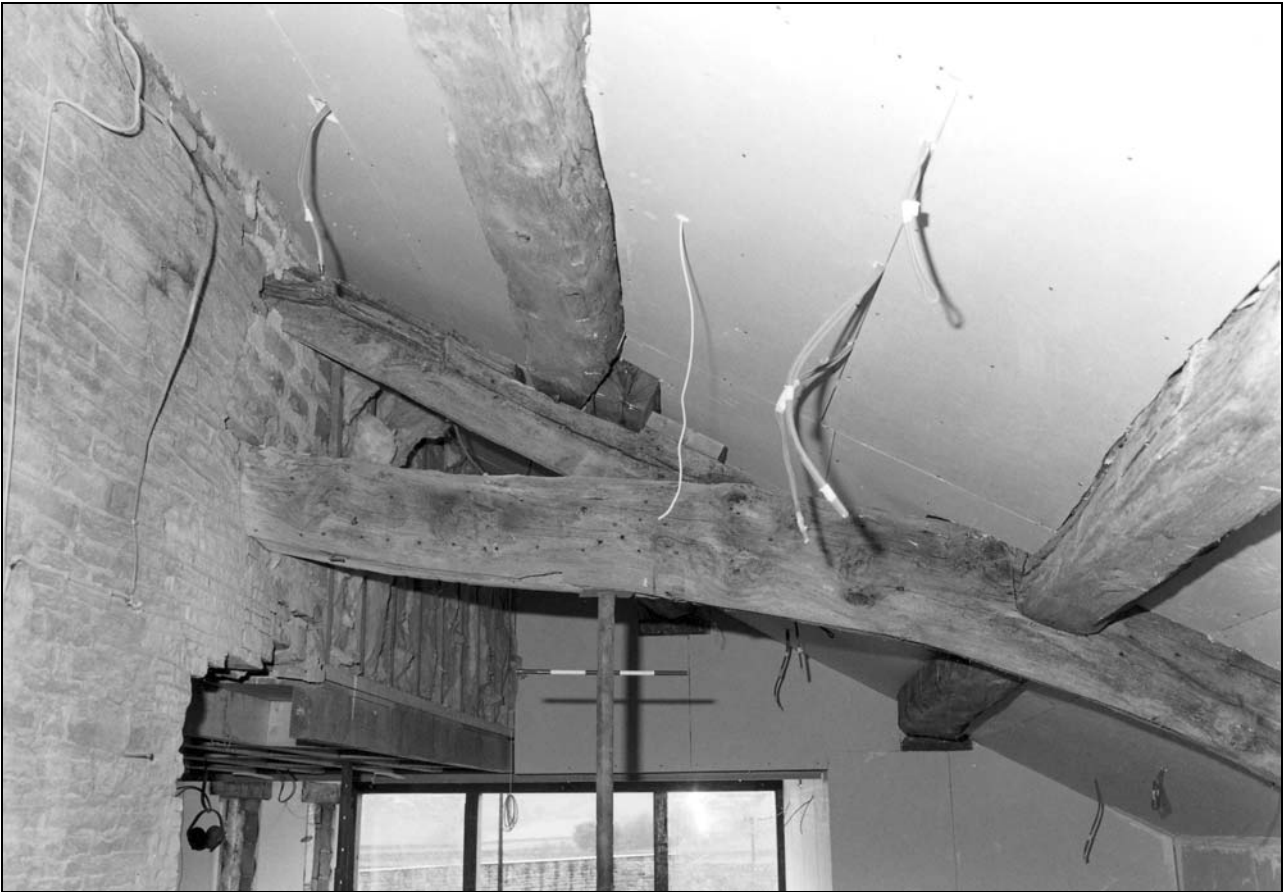
Photo 23: Baltic timber mark on softwood beam, crossing western cart entry (film 2, frame 3)
