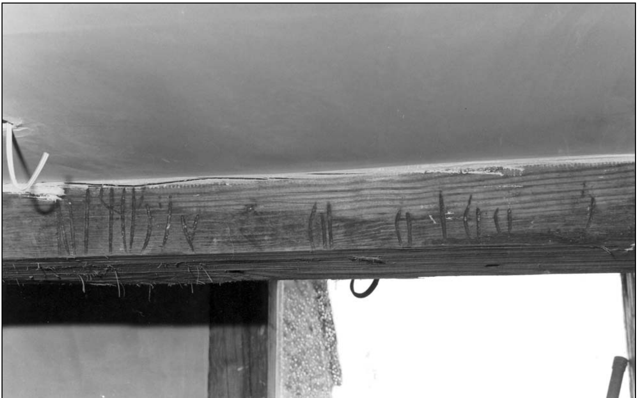
Photo 24: Roof structure in lean-to cart shed at north-east corner, from the south (film 1, frame 13)
