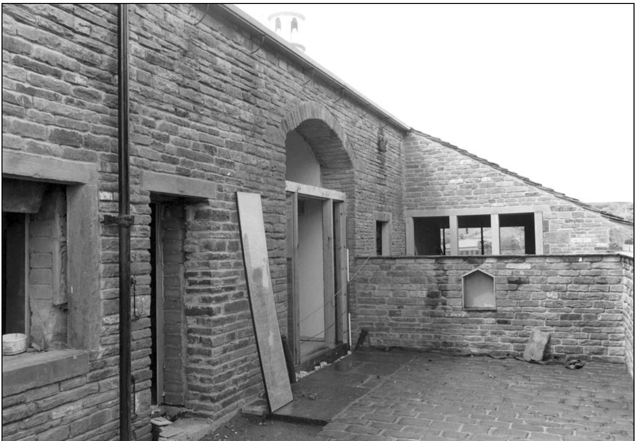
Photo 2: The east elevation, with arched cart entry and lean-to cart shed beyond (film 2, frame 7)
