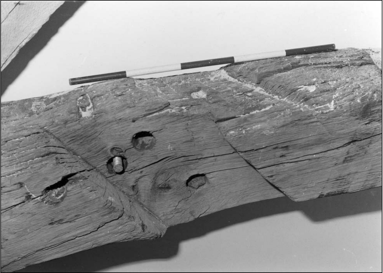
Photo 17: Detail of halving surviving from former cruck blade, tie beam of truss Y (film 1, frame 11)
