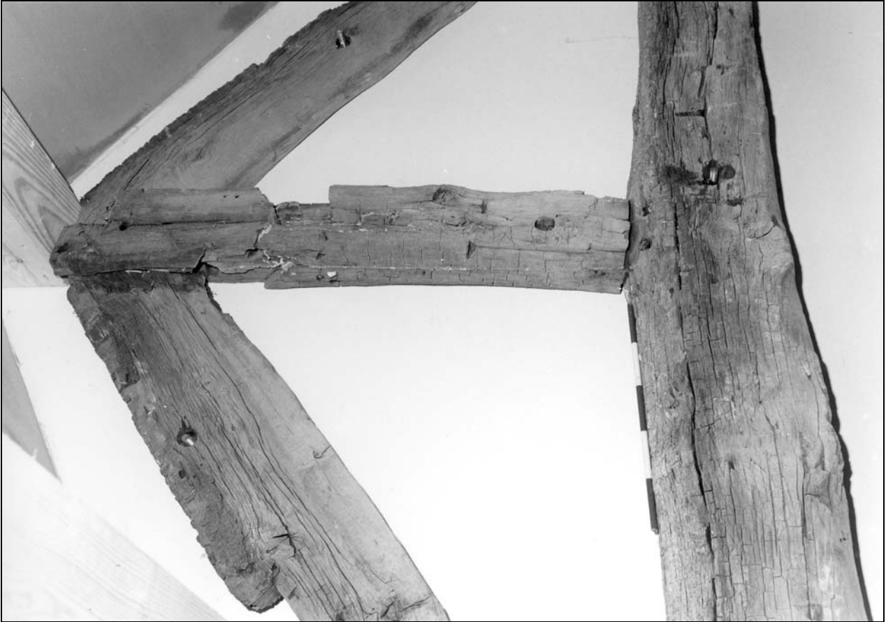
Photo 21: King post of truss Z, showing diagonal halving on side (film 1, frame 18)
