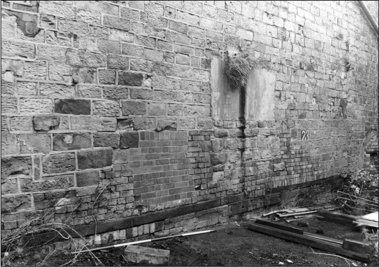
Photo 13: Building 1: external view of west wall with tops of furnace openings at ground level (film 1, frame 13)
