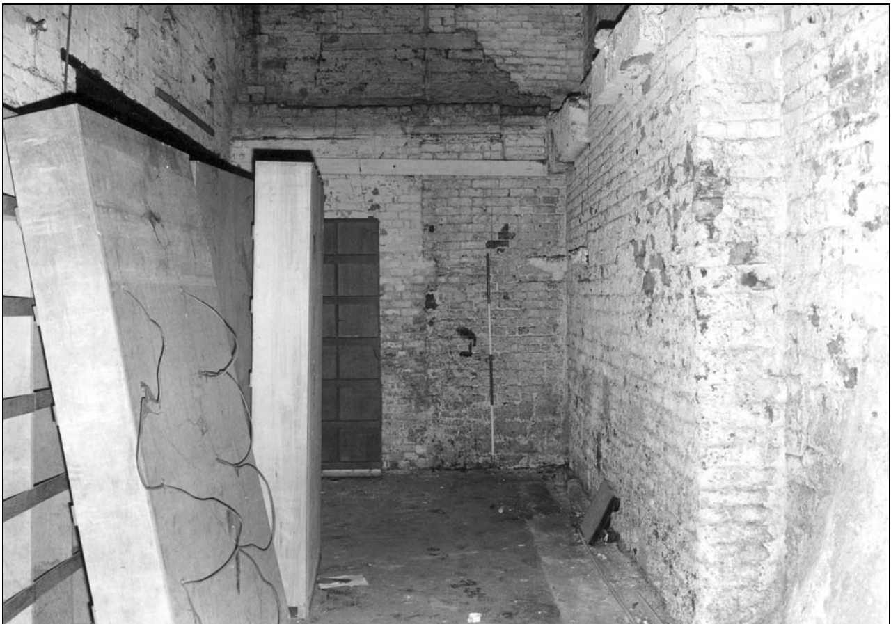
Photo 24: Building 1: enclosed area at ground floor, by south wall, from the west (film 3, frame 14)
