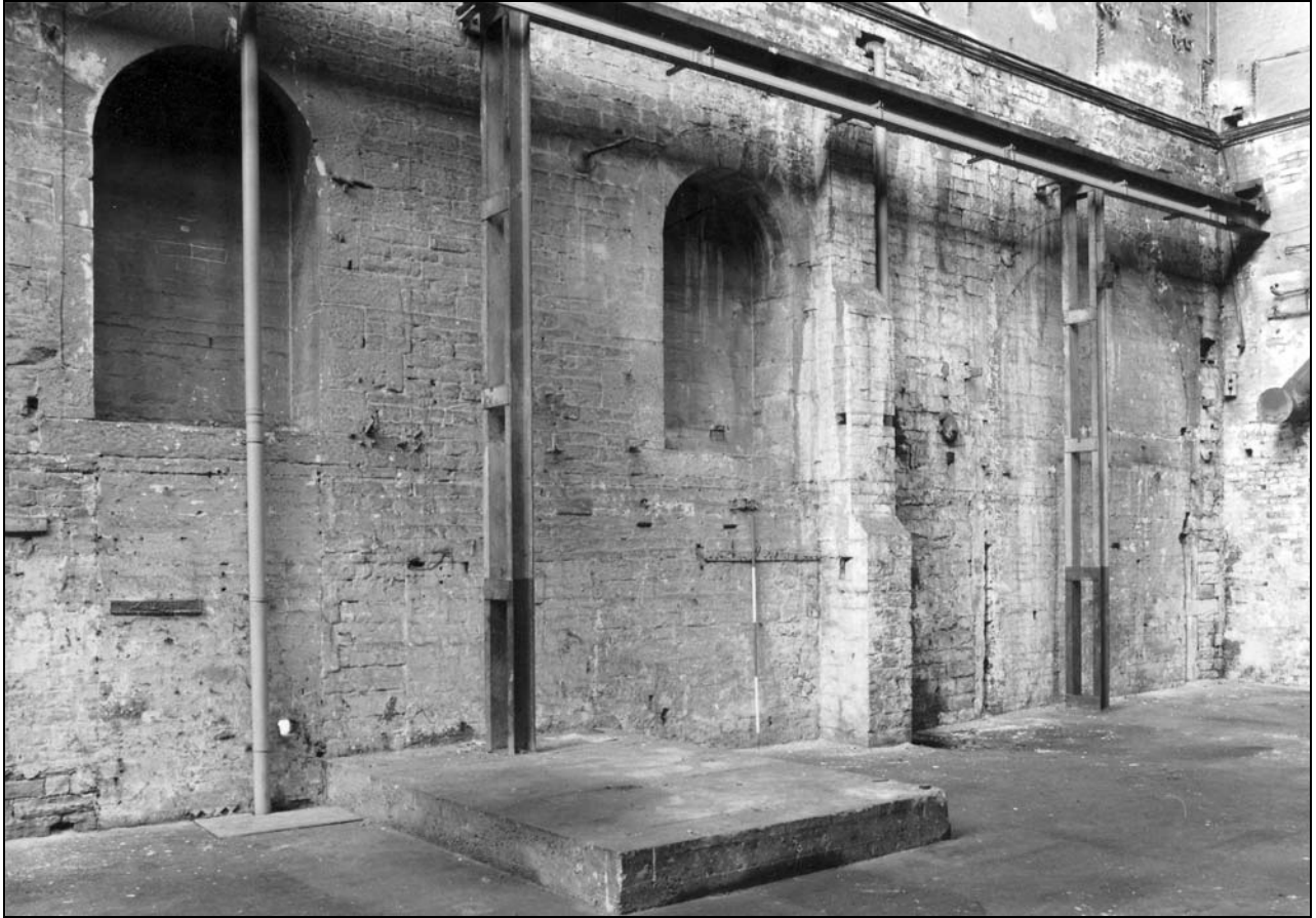
Photo 42: Building 1: external view of east wall, north end, now within Building 2 (film 2, frame 10)
