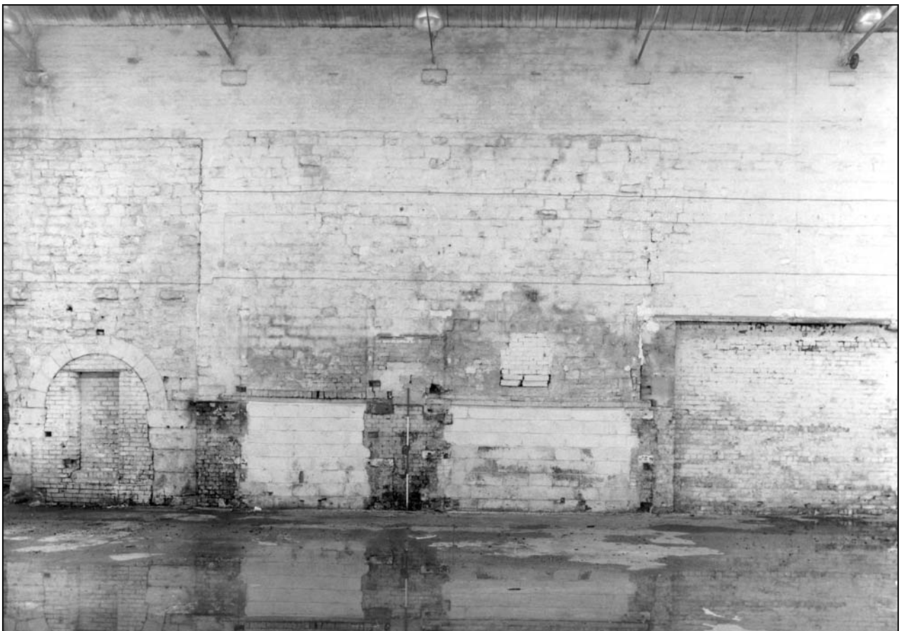
Photo 14: Building 1: internal view of west wall, with former openings to furnaces (film 4, frame 11)
