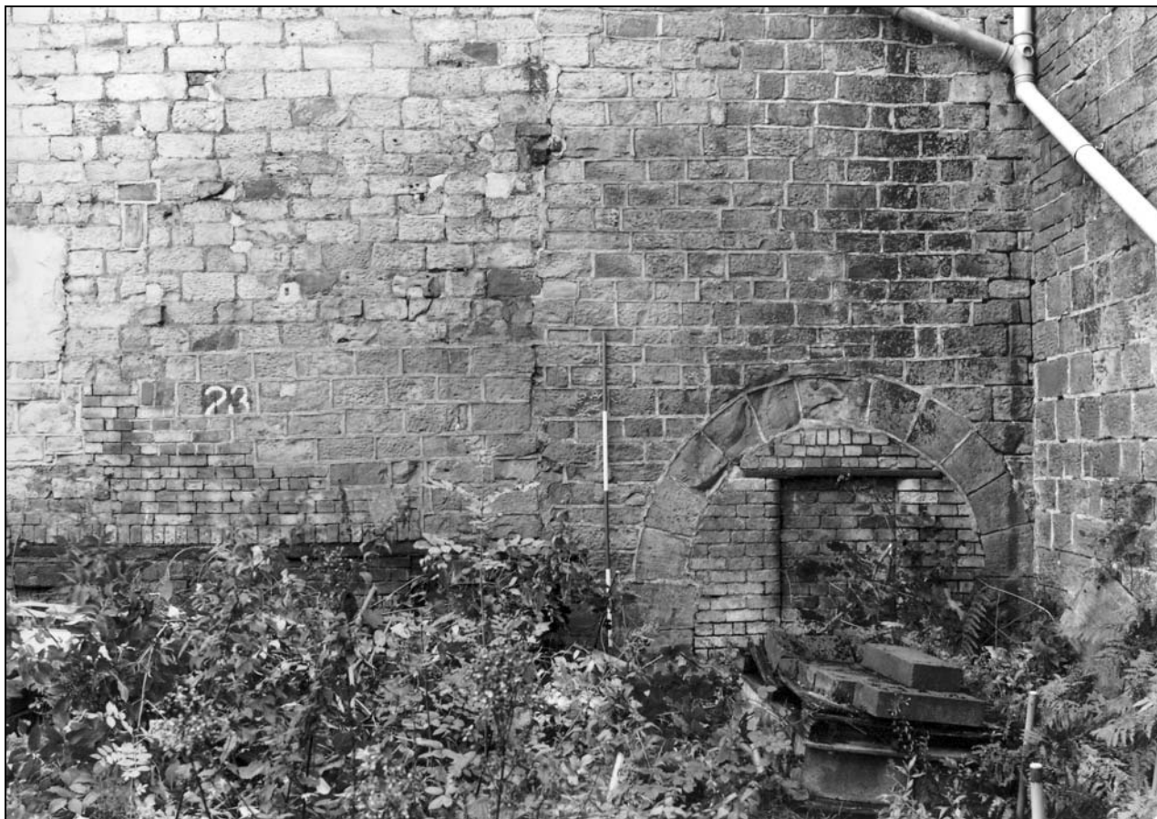
Photo 7: Building 1: external view of arched doorway in phase 1 wall in west side, with later phase to left (film 1, frame 12)
