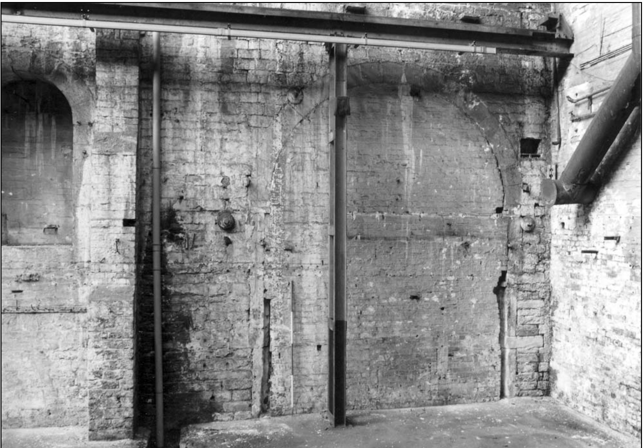
Photo 47: Building 1: external view of doorway at north end of east wall (film 2, frame 11)
