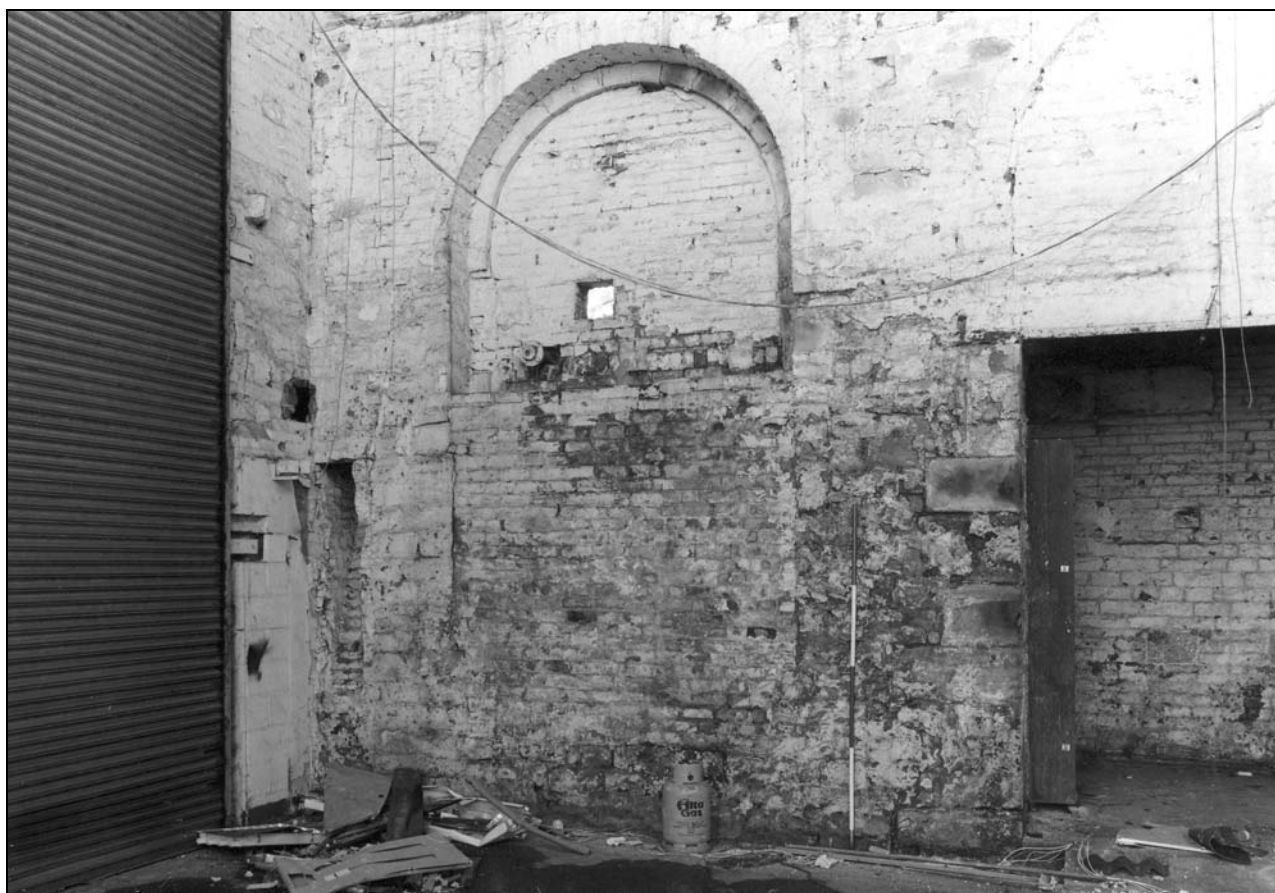
Photo 28: Building 1: interior view of south-east corner, with blocked window and corner flue (film 3, frame 4)
