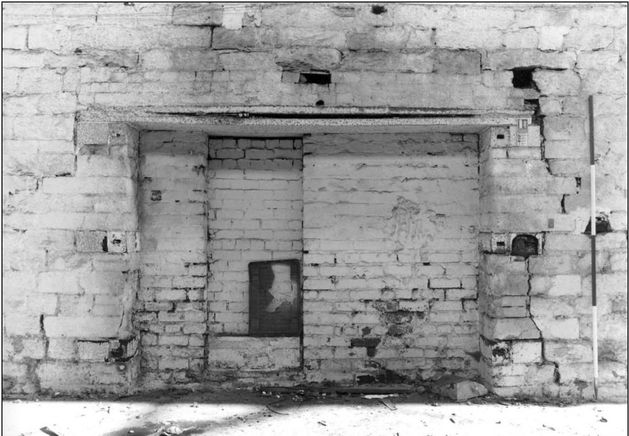
Photo 51: Building 1: internal view of blocked opening to former furnace, east wall (film 4, frame 3)
