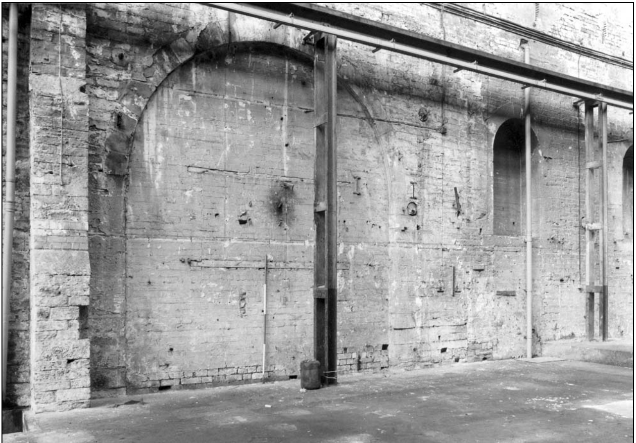
Photo 39: Building 1: external view of east wall, now within Building 2, with blocked, tall arched doorway (film 2, frame 9)
