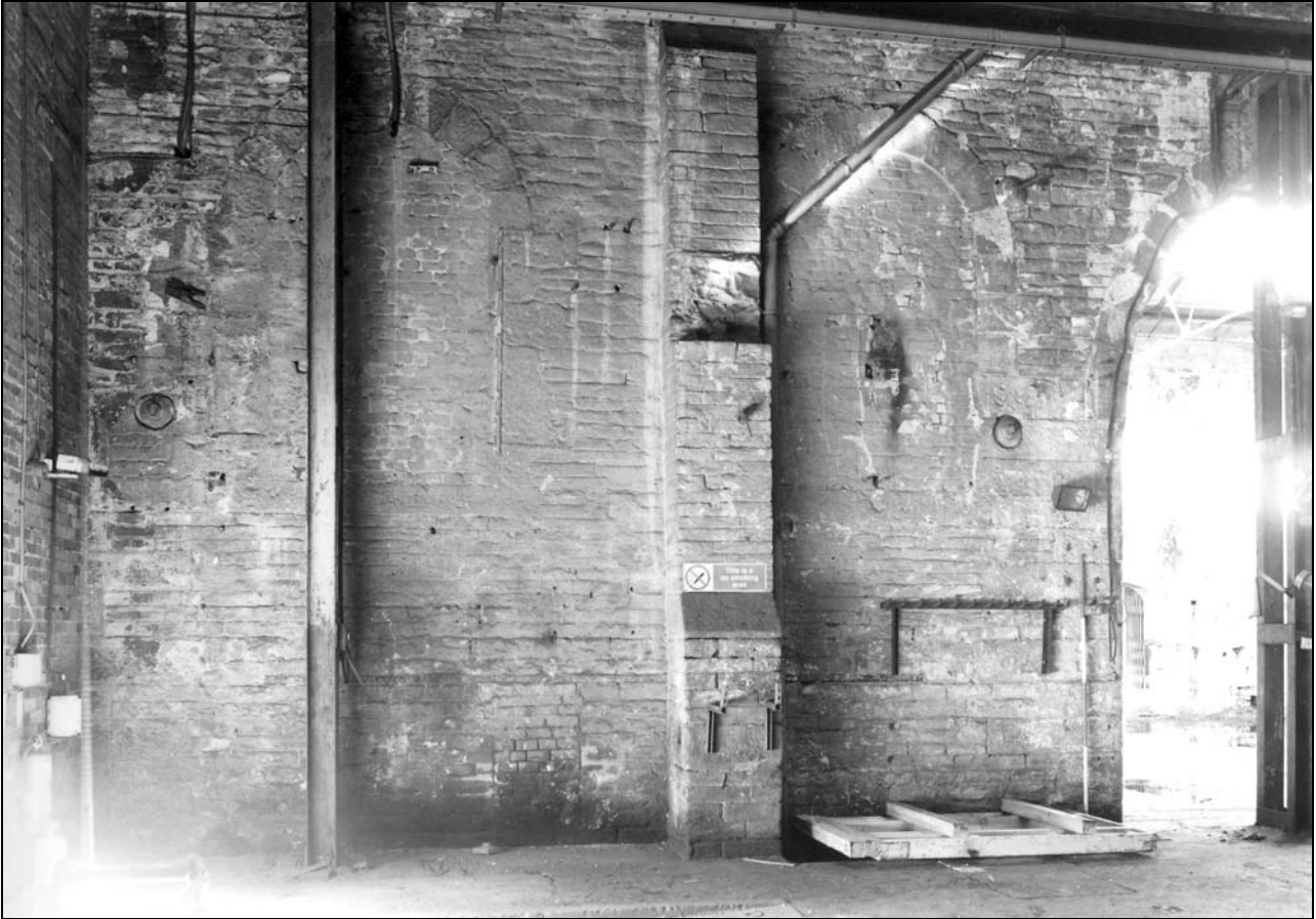
Photo 38: Building 1: external view of east wall, now within Building 2, with mid-height arched windows (film 1, frame 18)
