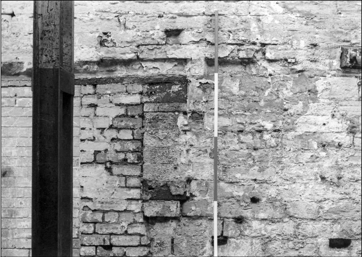
Photo 50: Building 1: external detail of refractory jamb to blocked opening to former furnace, east wall (film 2, frame 5)
