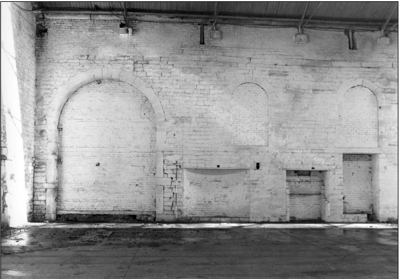
Photo 49: Building 1: internal view of doorway at north end of east wall (film 4, frame 1)
