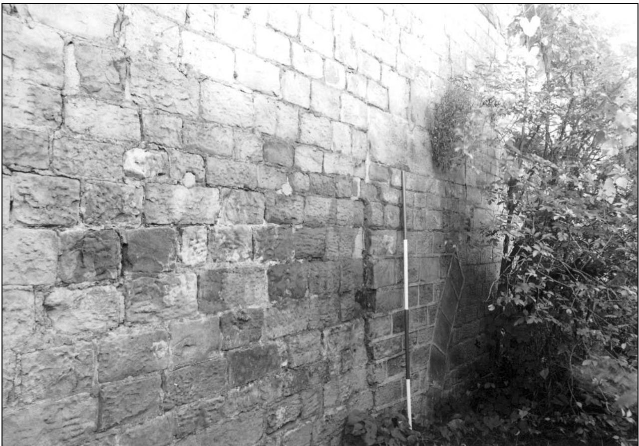
Photo 20: Building 1: external view of west wall, north end, showing arch slighted by inserted colonnade (film 1, frame 17)
