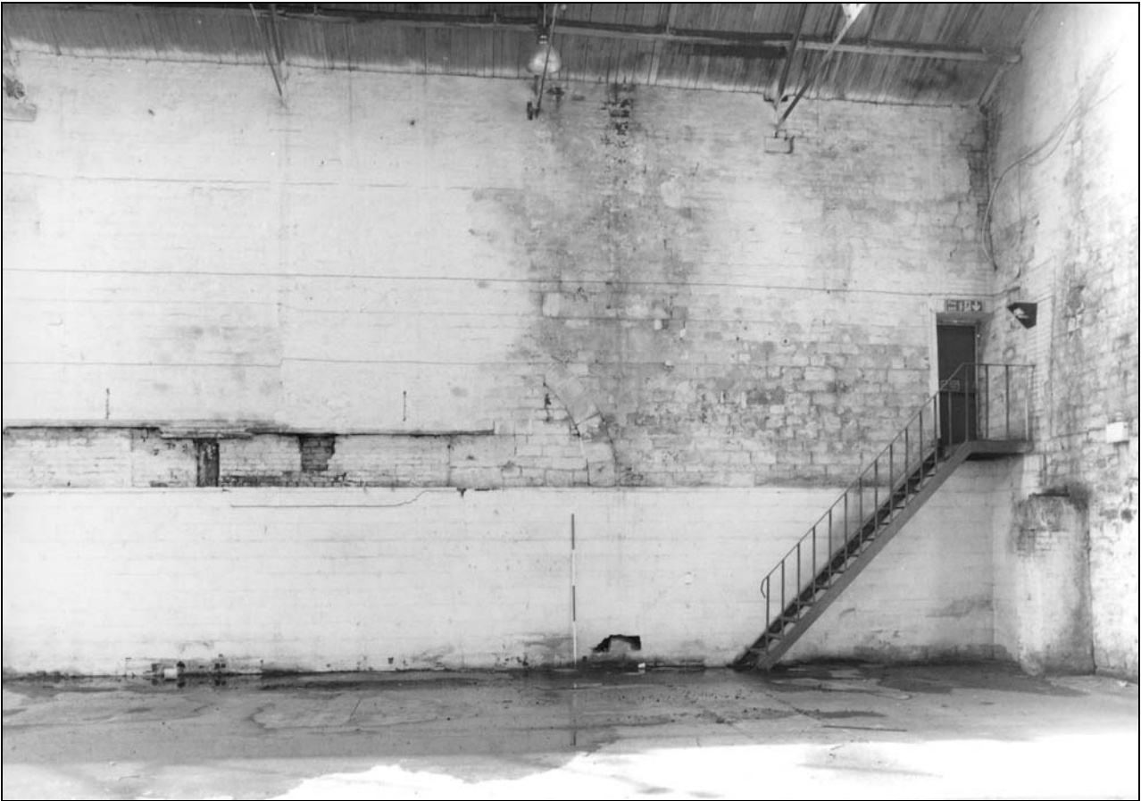
Photo 21: Building 1: internal view of west wall, north end, showing arch slighted by inserted colonnade (film 4, frame 13)
