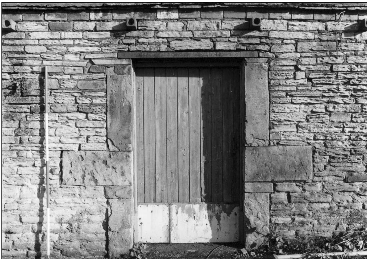
Photo 12: Doorway in west side of Building 1, at upper ground floor level (film 3, frame 7)
