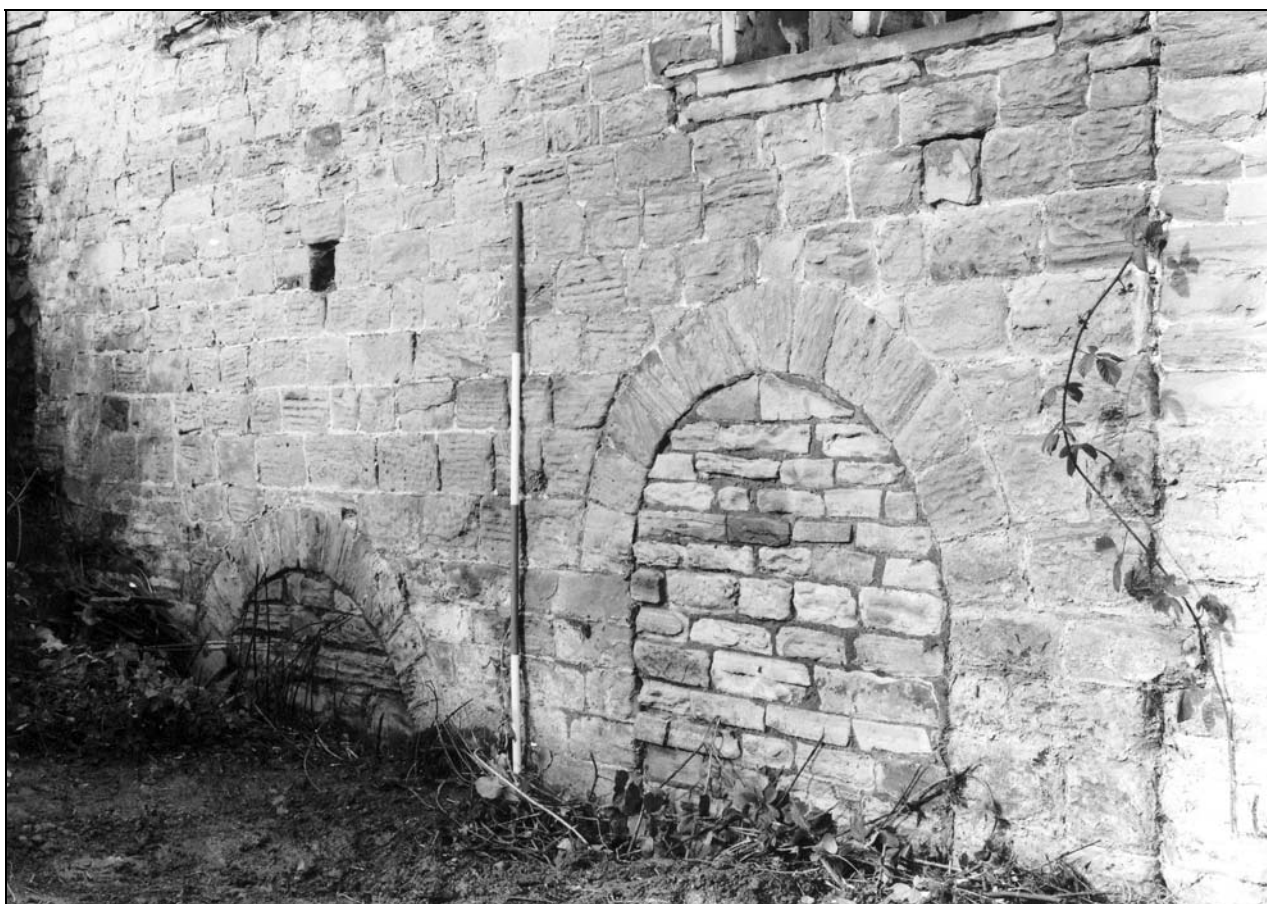
Photo 5: Blocked arches in south side of Building 1 (film 1, frame 17)
