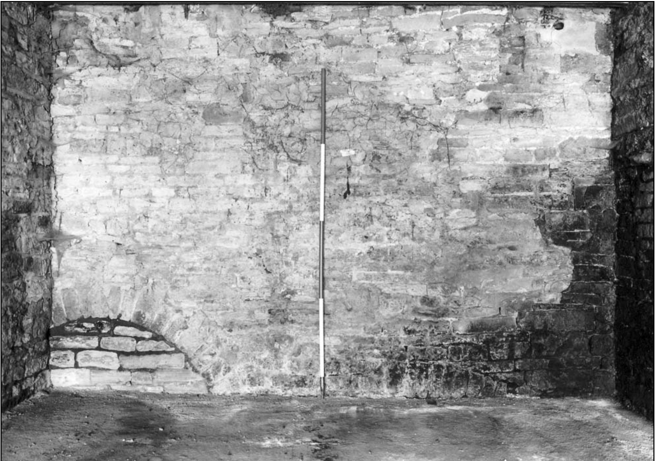
Photo 18: Building 1: tops of blocked arches in south side of west ground floor room (film 2, frame 6)
