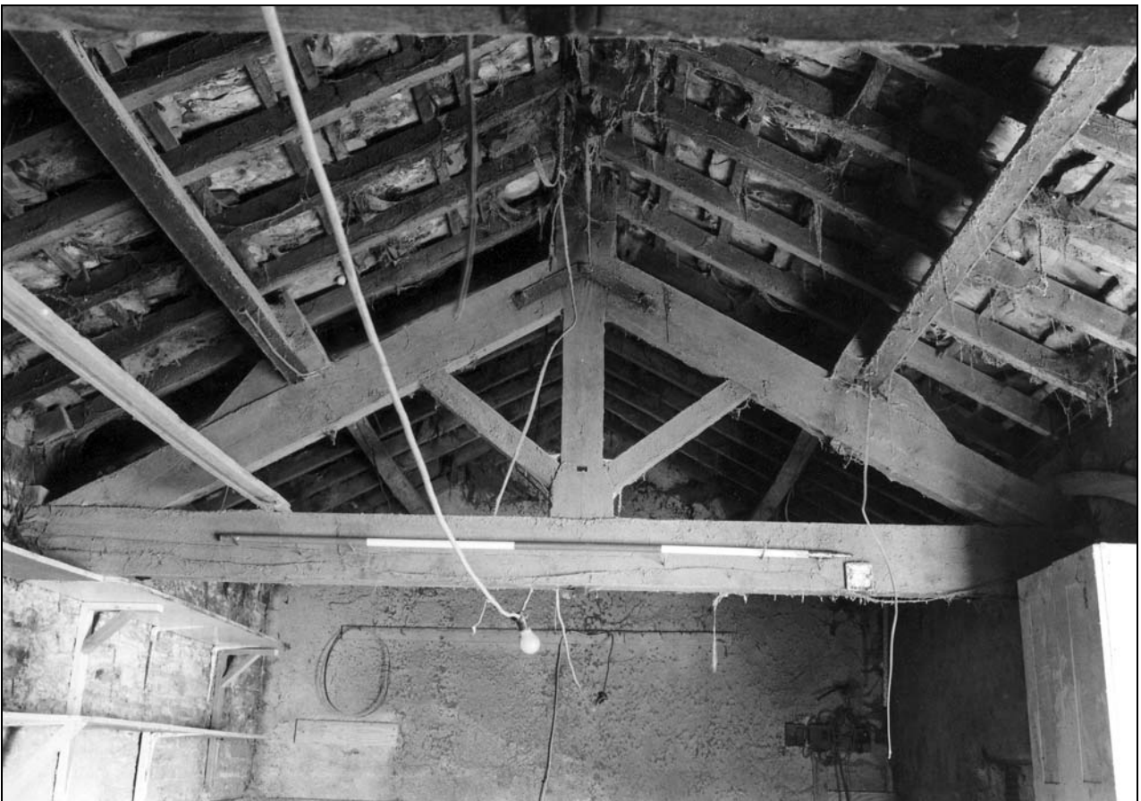
Photo 31: Building 1: roof truss over upper ground floor room, from the north (film 3, frame 5)
