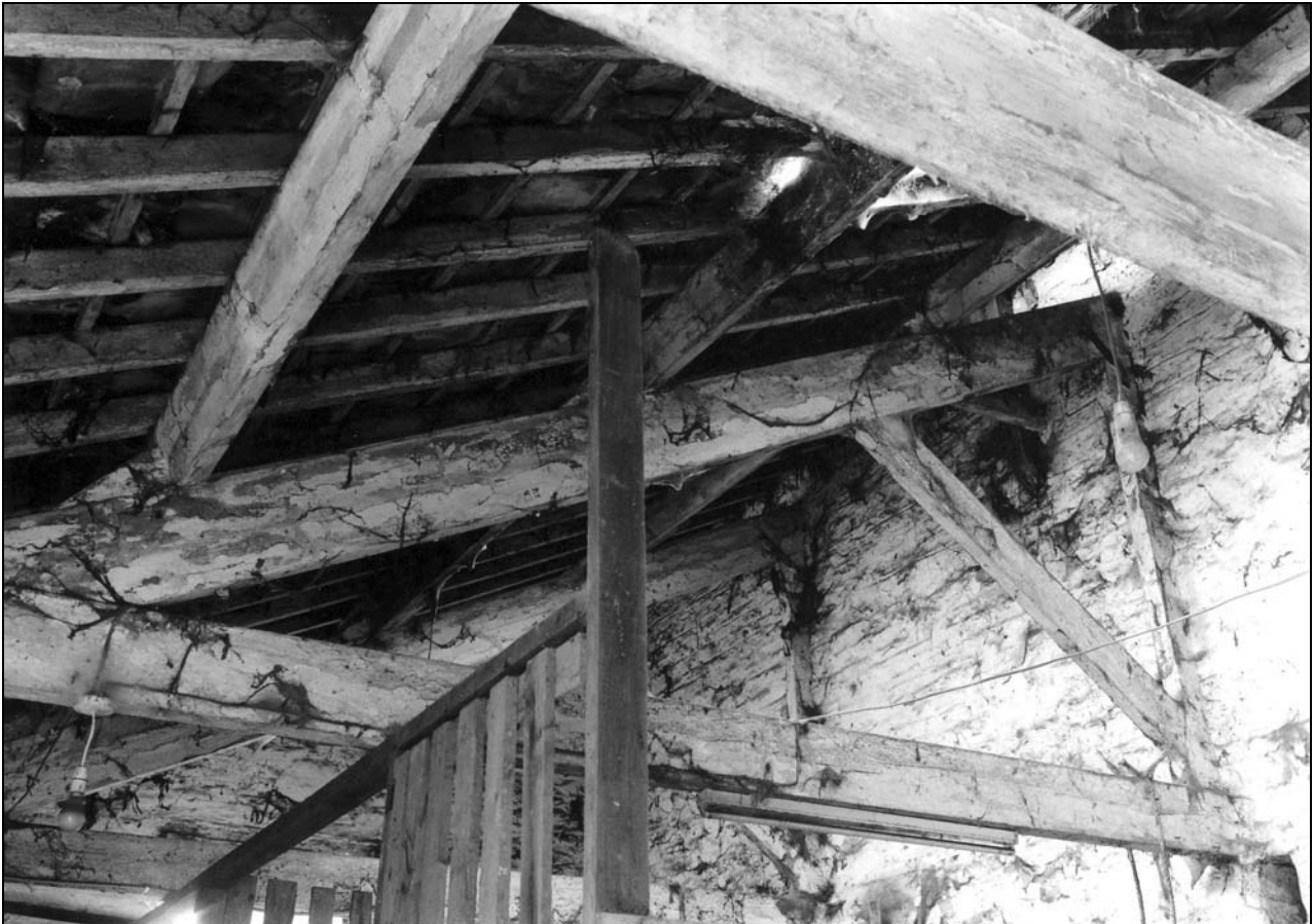
Photo 28: Building 1: roof structure over east ground floor room, from the north (film 2, frame 1)
