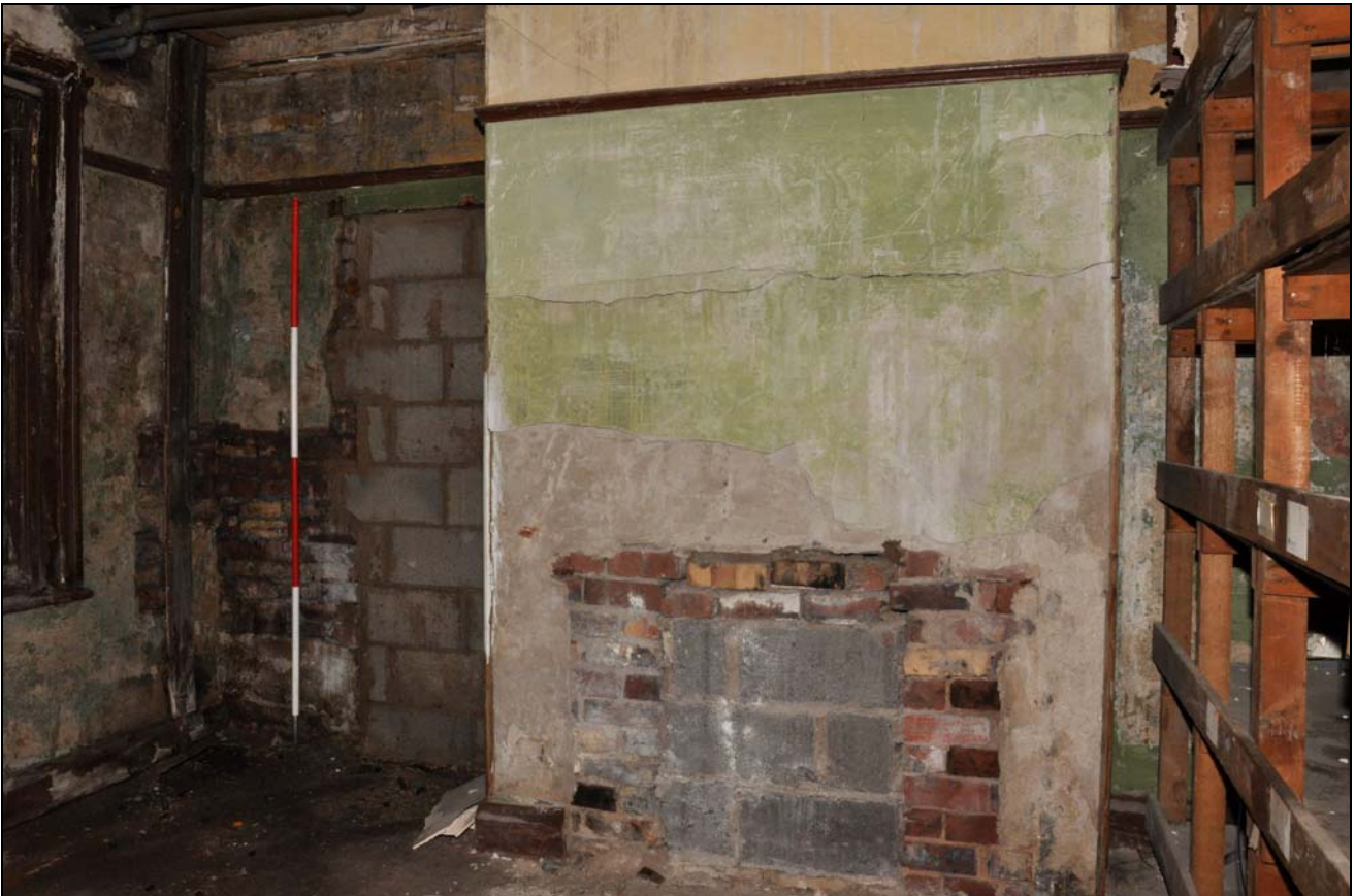
Photo 13: Building 1 – interior of later addition on ground floor, phase 2, from the south-east
