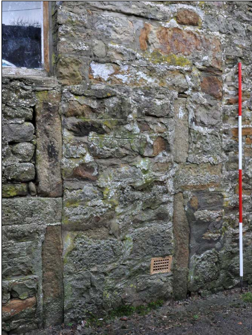
Photo 5: Blocked doorway in south gable
