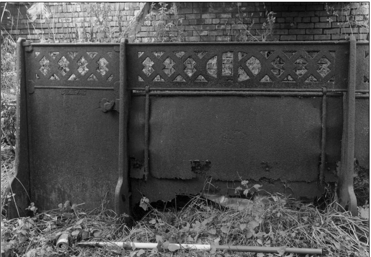
Photo 39: Building 3 (west end): cast iron pig pen front panel, by Ouden King (film 3, frame 1)
