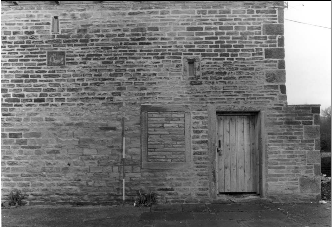
Photo 9: Building 1 (barn): mistal doorway and blocked window in south elevation (film 1, frame 11)
