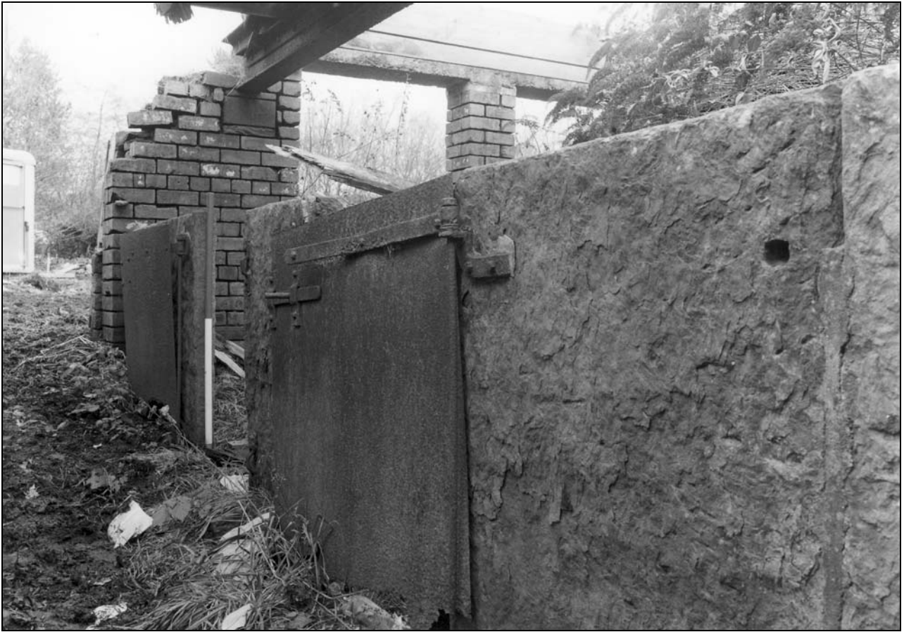
Photo 36: Building 3 (east end): flagstone wall and cast iron door to pig pen (film 3, frame 2)
